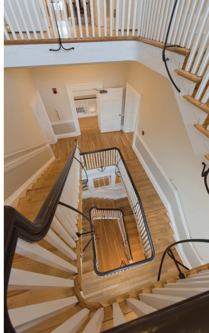
Above. Looking down the east stair, new heart-pine flooring is seen on the lowest level and refinished floors on the other levels.
