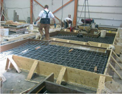
Panel fabrication. Bricks are set face down in rubber liners, reinforcement and embeds are placed and concrete is poured. For large runs, multiple liners can be cast from the master for the simultaneous production of identical panel types.
