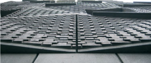
Completed and installed panel details. The joints between panels are integrated with the global design of the facade and panel order. Panels at the south wall, residential entrance and store front are cast from the tinted grey concrete that is used as the mortar material on the brick panels.
