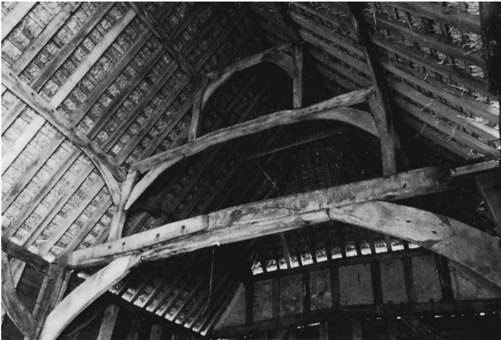
Fig. 3.10 Fifteenth-century timber-framed barn at Newton Flotman, Norfolk showing fine double queen-post roof. (Photograph by Stephen Heywood.)
