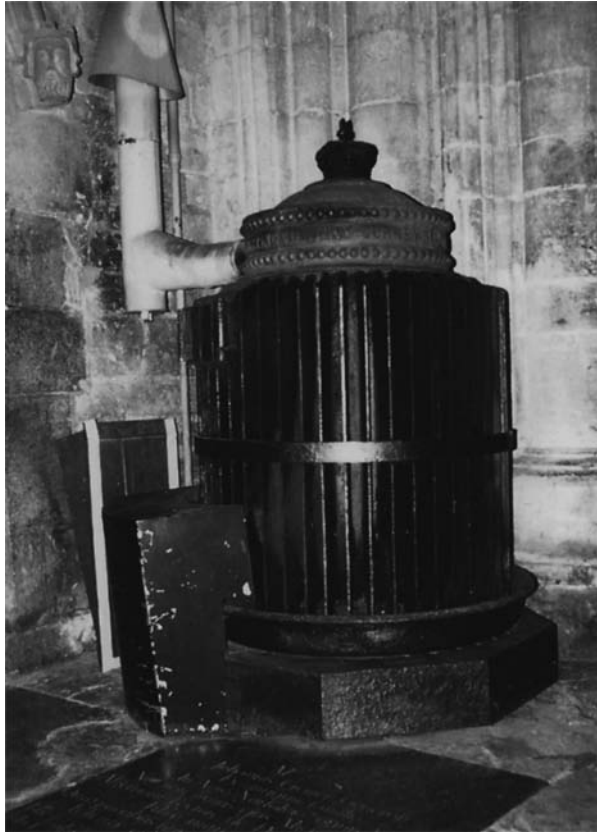
Fig. 3.30 The Gurney coke-fired stoves in Ely Cathedral, Cambridgeshire were converted to gas in the 1970s.
