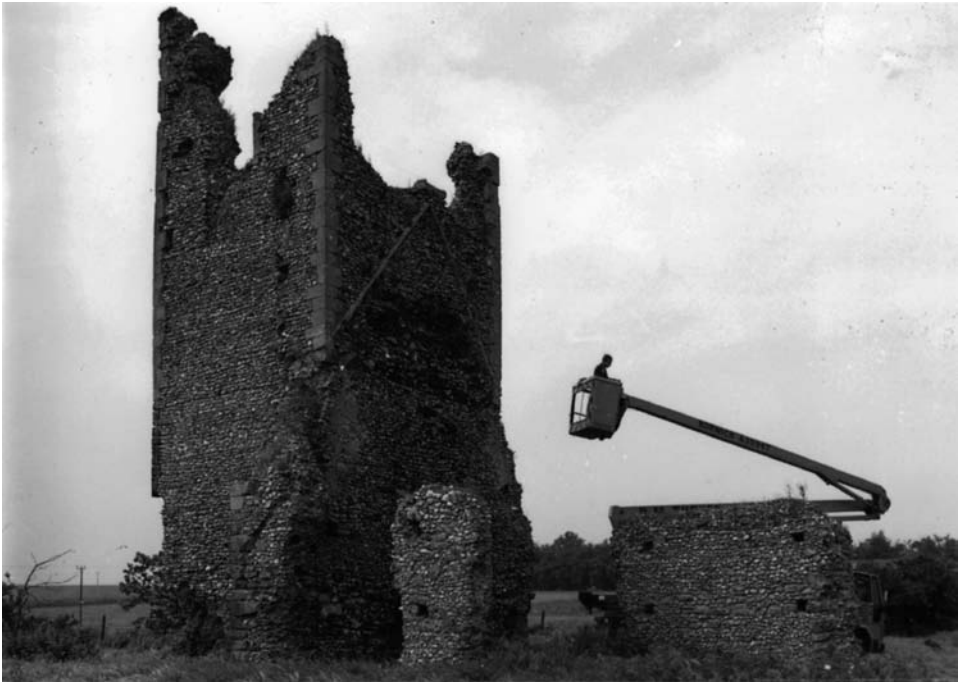
Fig. 5.1 Mobile hoist used in the preliminary inspection of an unstable masonry structure.
