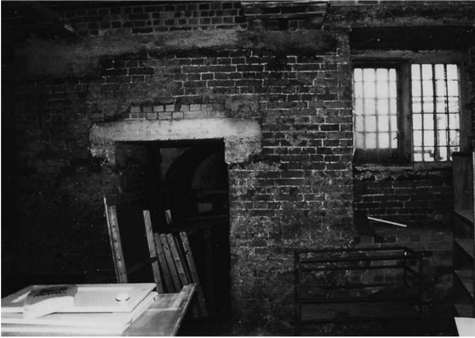
Fig. 6.9 Basement wall with crystals of pentachlorophenol following earlier irrigation treatment.
