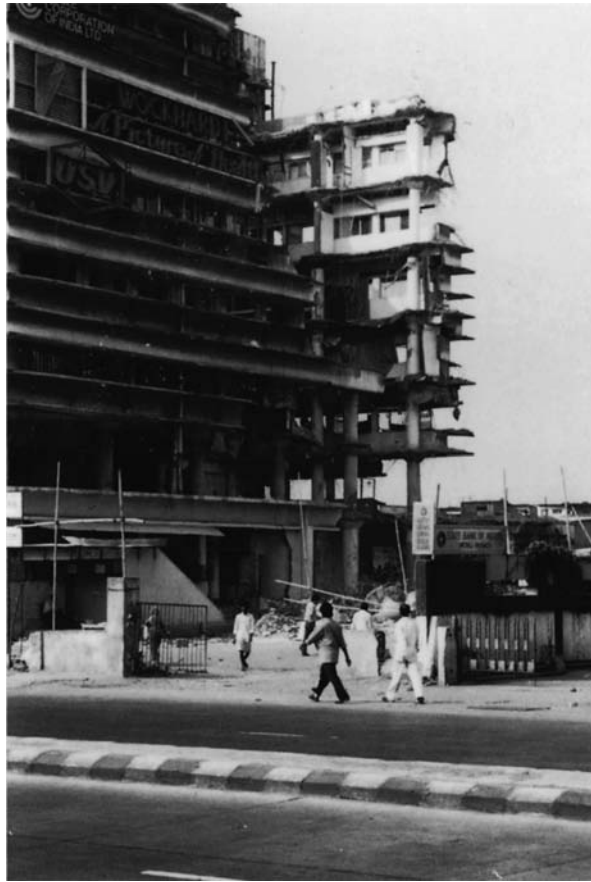
Fig. 3.1 Collapse of a concrete-framed building in Mumbai as a result of ill-conceived structural alterations and lack of maintenance.
