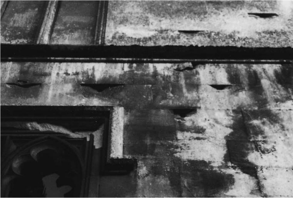
Fig. 4.16 Corrosion of embedded ironwork resulting in damage to stone.
