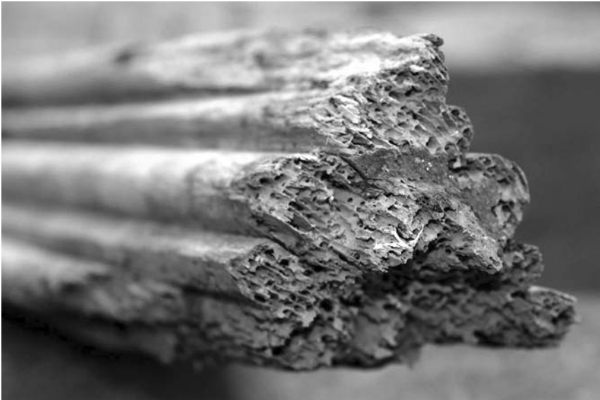
Fig. 4.23 Damage caused by deathwatch beetle ( Xestobium rufovillosum ) to roof timber.
