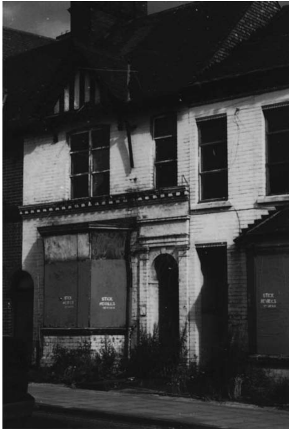
Fig. 5.8 Unoccupied buildings with boarded lower windows, missing lead flashing to bay window, broken glass, pigeons inside upper rooms, broken downpipes, vegetation growth to frontage and guttering, and slipped roof slates and tiles.
