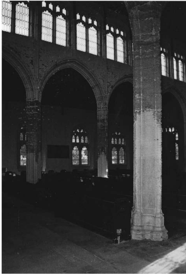
Fig. 6.4 Evidence of dampness and salt crystallisation to stonework of arcade piers.
