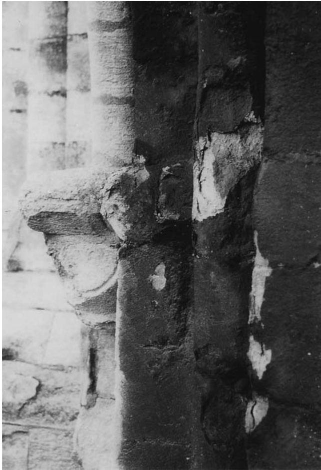
Fig. 4.10 Splitting and spalling of limestone surfaces in areas sheltered from direct rain-washing, due to the formation and subsequent failure of crystalline sulphate skins.
