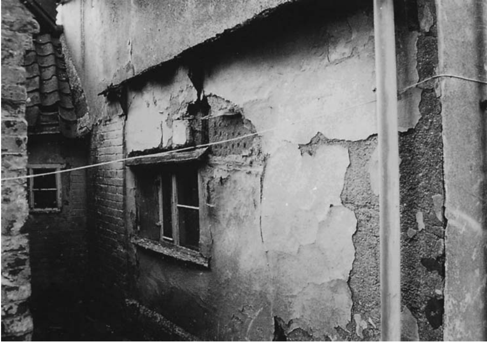
Fig. 7.7 A lack of maintenance will result in accelerated deterioration and decay, with long-term consequences for the use of the building.
