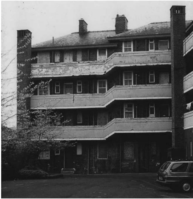
Fig. 7.12 Keeping unoccupied buildings, of whatever age or construction, in good order requires careful planning and appropriate levels of protection.
