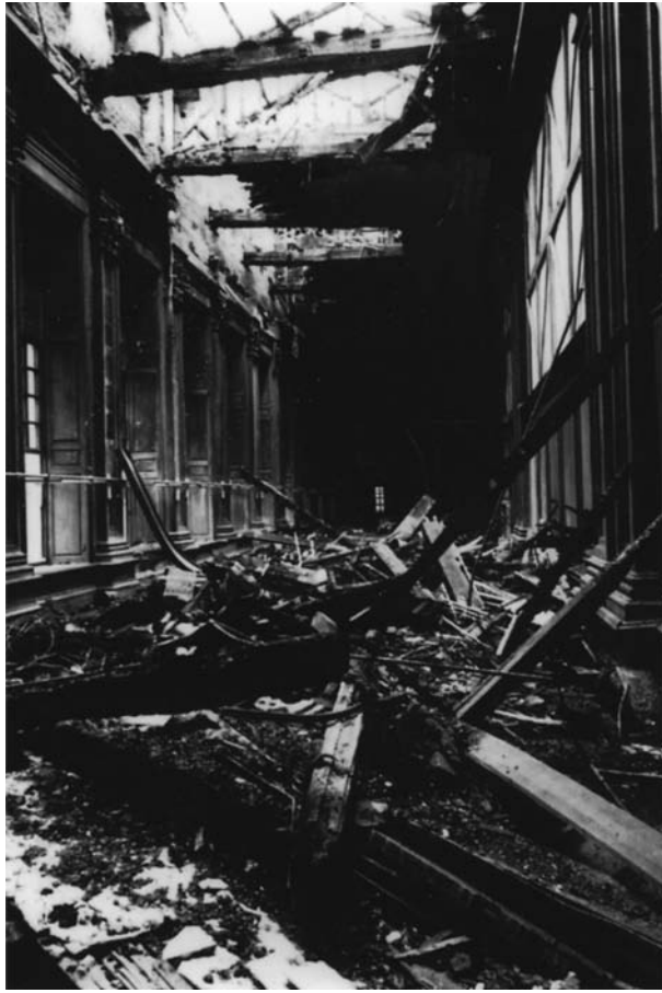
Fig. 4.24 Damage caused by fire within the Cartoon Gallery of Hampton Court Palace in April 1986. (Crown copyright: Historic Royal Palaces.)
