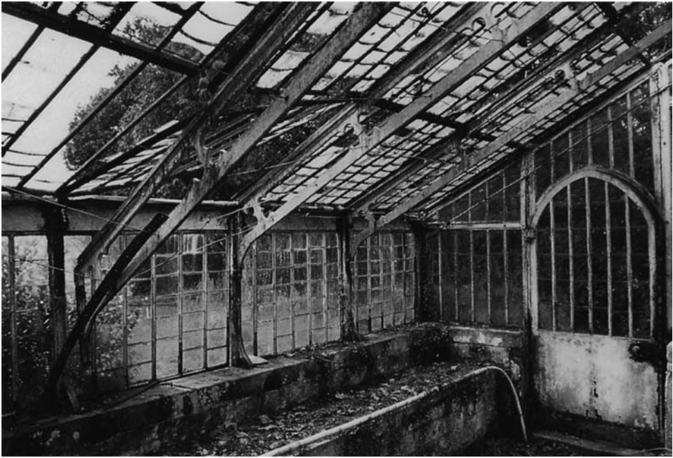
Fig. 4.15 Corrosion and failure of the connections between the decorative cast-iron rafters and frame members in a mid-nineteenth-century glasshouse.
