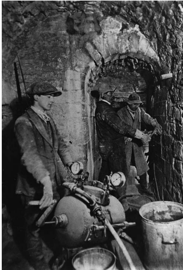
Fig. 3.32 Powered by compressed air, a pump was employed to fill the voids in the masonry corework at Lincoln Cathedral with Portland cement grout as part of the Special Repair Programme (1922–32). (Lincoln Cathedral Works Archive.)
