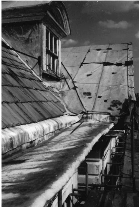
Fig. 4.17 Copper sheet used as a covering for the pediment and dormer roof, and lead for the dormer cheeks and as a weathering for the timber cornice. Both sheets metals have suffered from thermal movement on this south-facing section of the roof.
