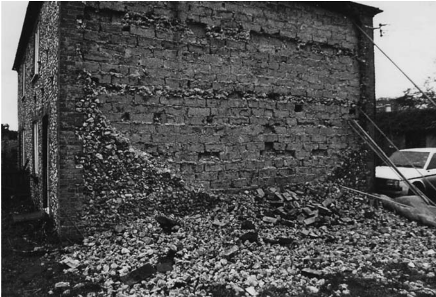
Fig. 3.5 Collapse of the flint facing to a clay-lump wall in south-west Norfolk. The bond between the two materials was minimal, making it susceptible to deformation and failure.
