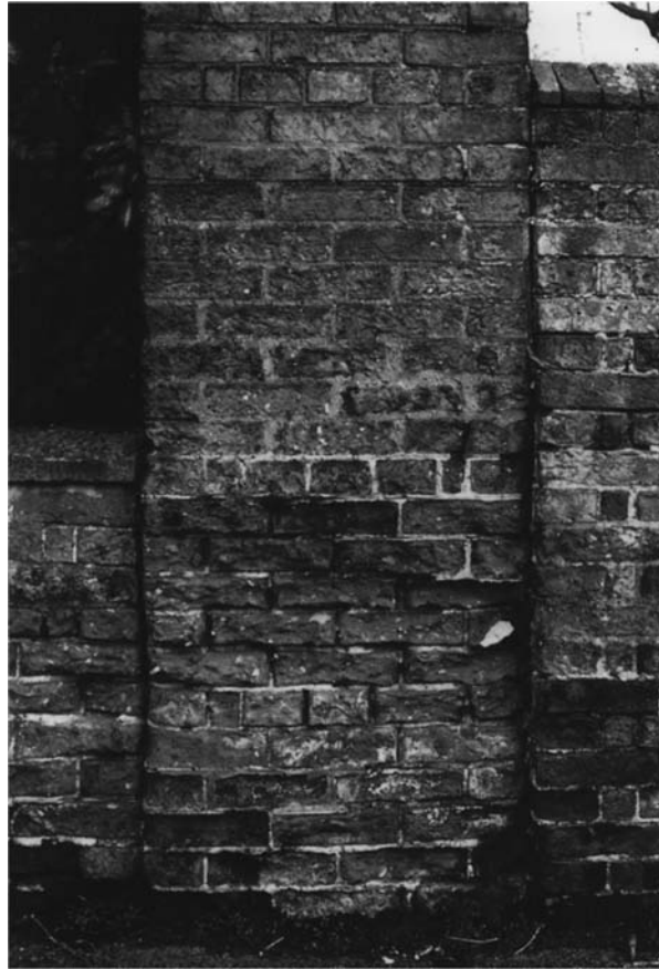
Fig. 4.8 Failure of brickwork caused by the frost action.
