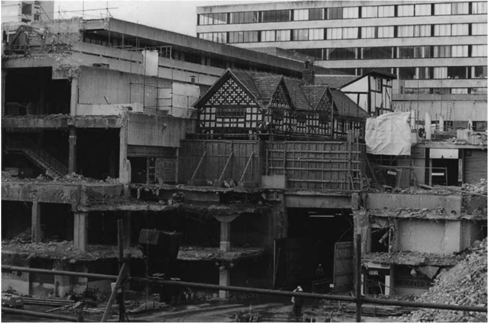
Fig. 3.7 The medieval timber-framed Old Wellington Inn and nineteenth-century Sinclairs in Manchester following extensive bomb damage to adjacent buildings in 1996. Both buildings had been raised up by over 1.4 m during the 1970s to accommodate a reinforced-concrete deck for a shopping development, and were again moved and resited as part of a recent redevelopment scheme. (Photograph by Stephen Welsh, Buttress Fuller Alsop Williams.)
