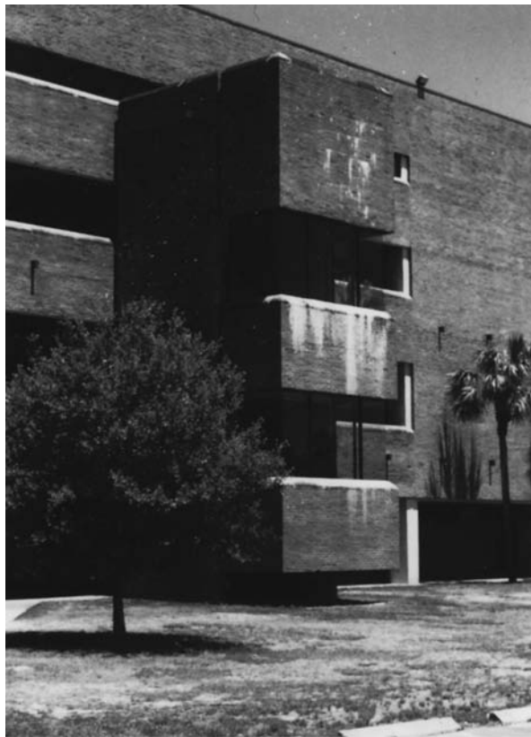
Fig. 4.18 Persistent efflorescence on brickwork where rainwater is not effectively removed from the construction.
