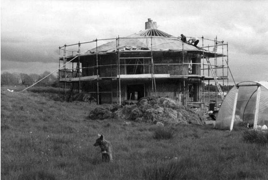
Fig. 3.14 The Spiral House in County Mayo, Ireland is Europe's first two-storey, load-bearing straw-bale house and was constructed by Amazon Nails and volunteers in 2000–01. (Photograph by Amazon Nails.)
