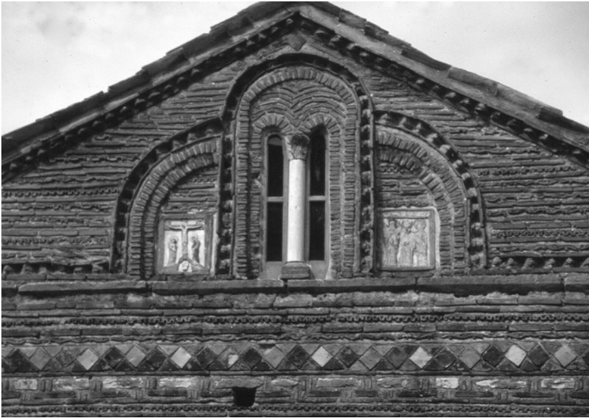
11.16. Arta, Church of H. Vasileios, east end; detail, gable, twelfth century. Photo Slobodan Ćurčić.
