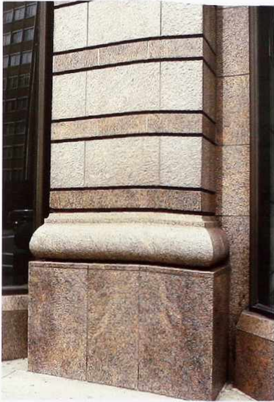
CP-45 Banded granite veneer pilaster on Tuscan-style base, entry of modern commercial building
