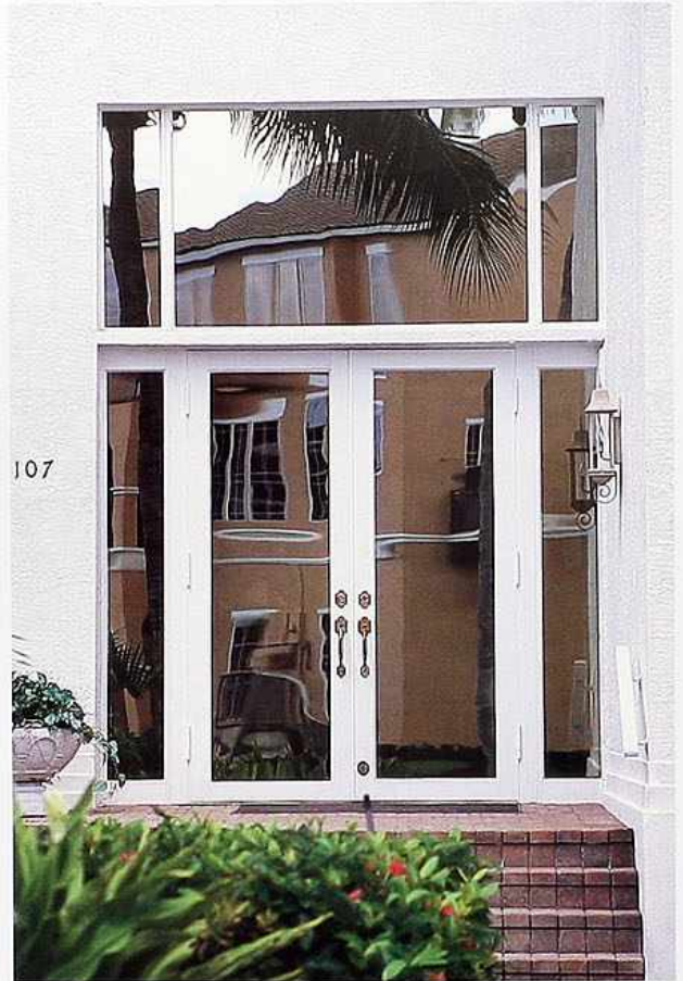
DW-67 Full glass double doors and side lights with three-light transom, modern house
