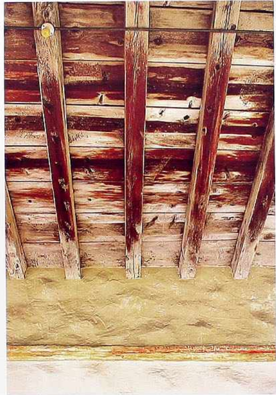
CR-2 Roughly hewn exposed rafters anchored in adobe wall and covered with rough-sawn planks; 18th-c. American Southwestern mission
