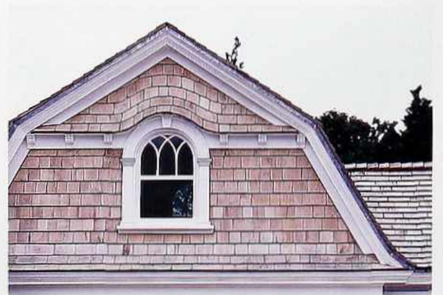
FA-52 New Alaskan yellow cedar shakes in common coursing, eyebrow window, gambrel roof
