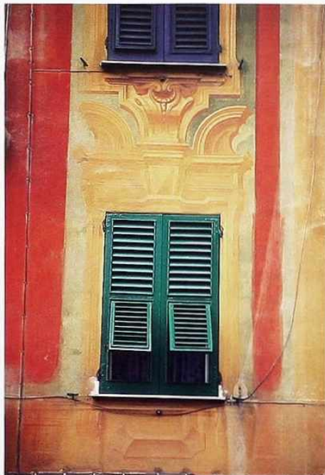
FA-83 Weathered trompe l'oeil moldings and pediment around shuttered windows on Tuscan wall
