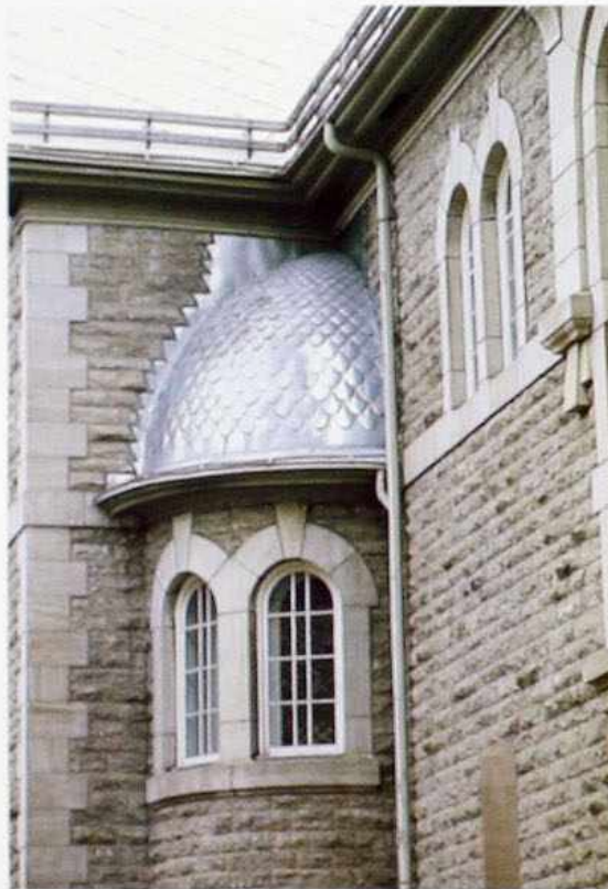
CR-32 Quilted sheet metal on dome roof of corner turret with flashing at juncture of dome and wall
