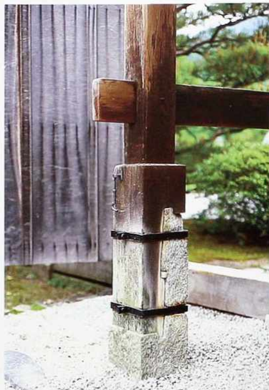
CP-106 Timber post connected to stone plinth with rabbeted scarf joint and metal hoops. Horizontal brace joined by mortise-and-through-tenon joint
