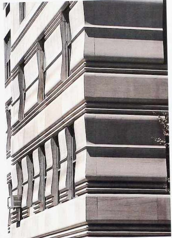
WA-98 Outside corner probably of Amherst gray limestone, sand-finished in shaped panels
