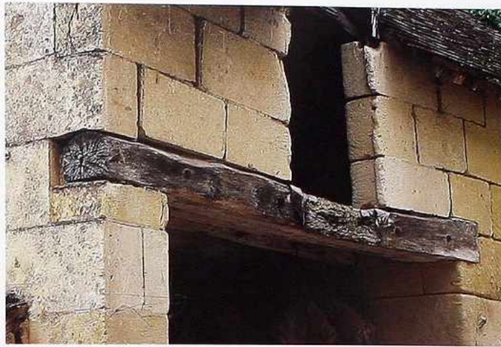
CP-109 Timber lintel in stone wall
