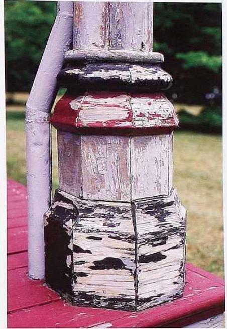
CP-55 Heavily weathered painted octagonal wood base in Carpenter Gothic style
