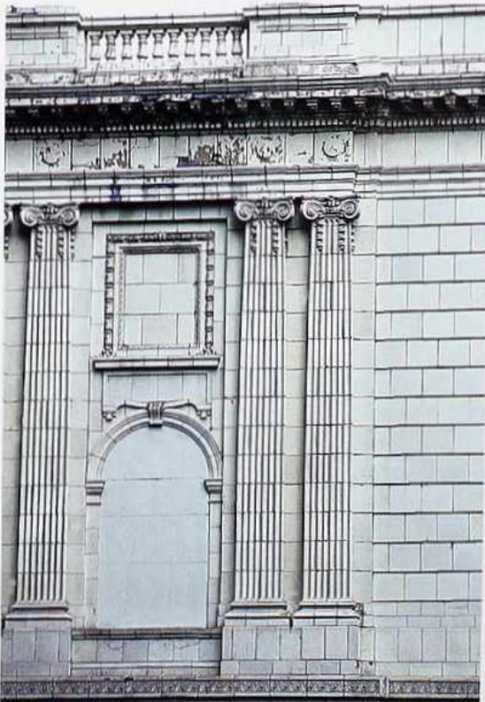
CP-86 Glazed architectural terracotta ionic pilasters with fluted shafts and angle-capitals; entablature with festoon, capped with balustrade
