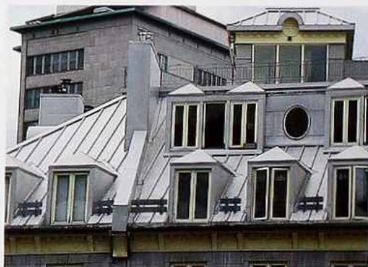
CR-102 Hipped-roof dormers on metal hipped roof with pipe snow guards, modern apartment house
