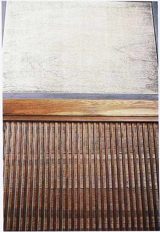
FP-5 Top to bottom: framed-wood raised floor; door sill; closely spaced narrow strips of wood over sawn planks
