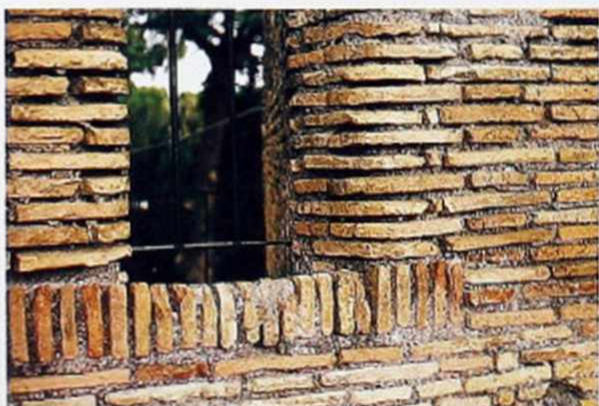
WA-158 Roman bricks with soldier course and shaped bricks forming crenel, ancient parapet wall
