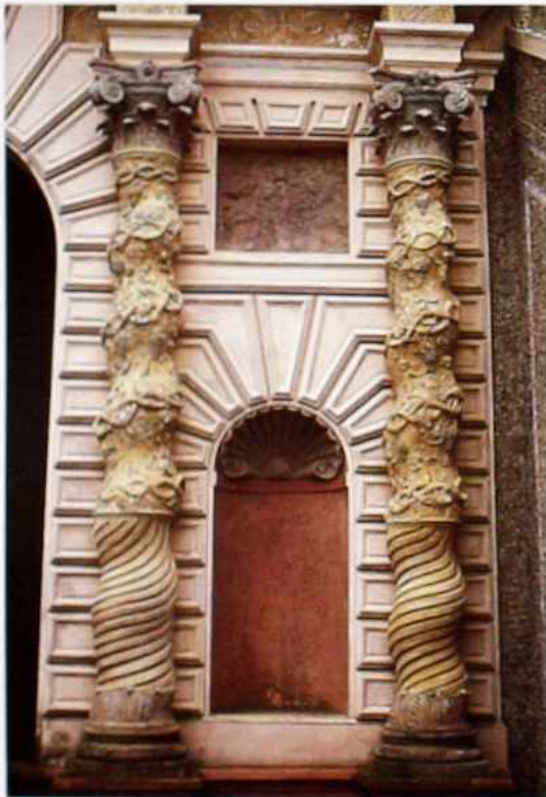
CP-67 Stone entryway with partially fluted Salomonic columns, garland ornament, and Composite capitals
