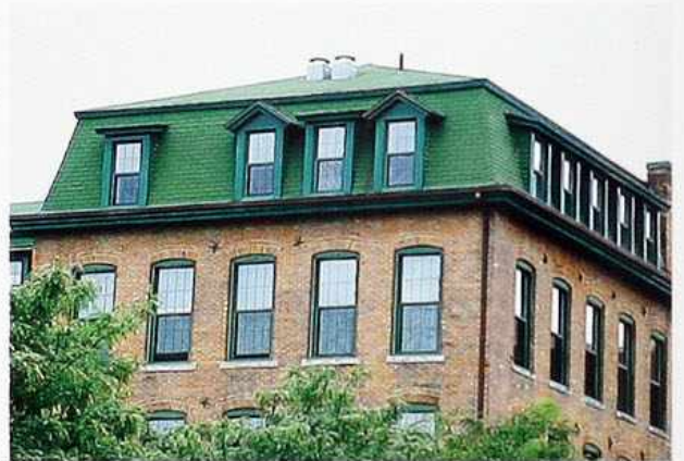
CR-118 Mansard with row of shed dormers (right) and alternating gable and shed dormers (left)
