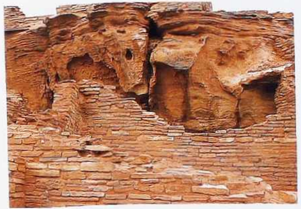
WA-77 Roughly squared sandstone in random ashlar attached to natural stone wall
