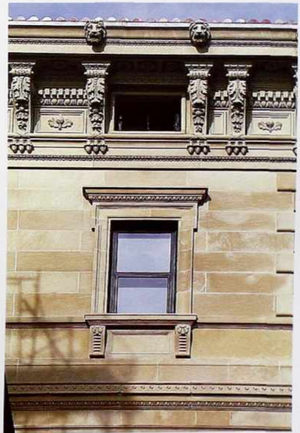
WI-125 Stone classical-style window casings with crown molding capping lower window; consoles supporting sill and cornice
