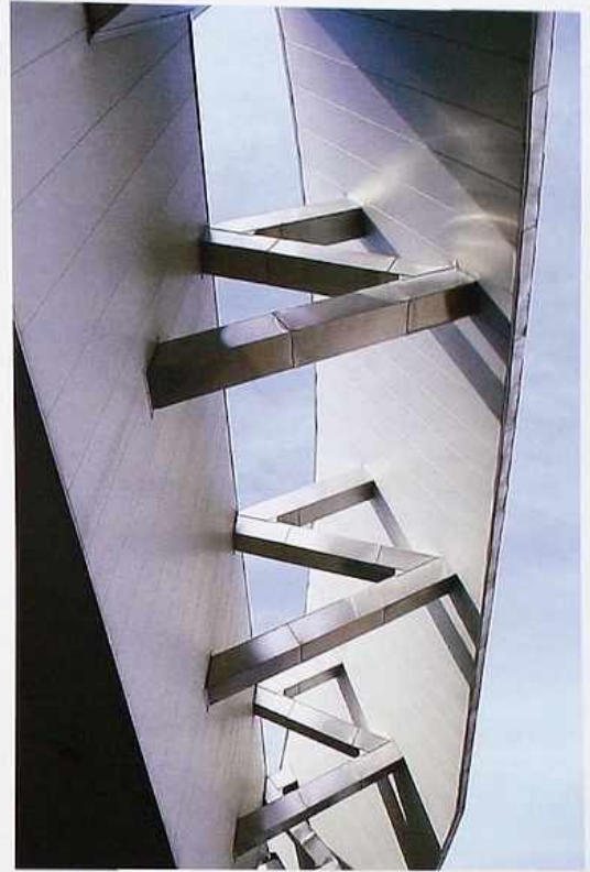
CR-110 Semidetached extension of metal roof connected to facade by Z-shaped brackets, modern commercial building
