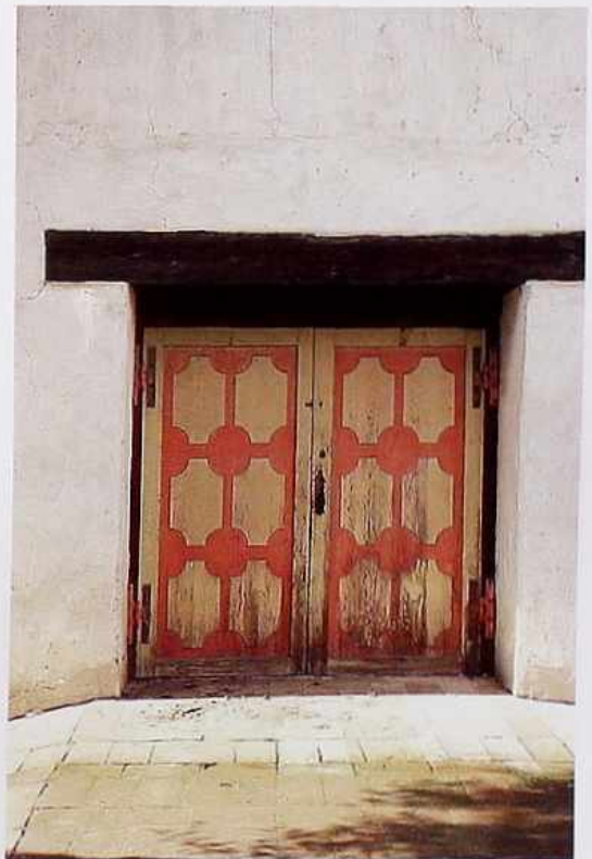
DW-44 Weathered double doors with painted panels; doorway recessed in stucco reveal with exposed timber lintel
