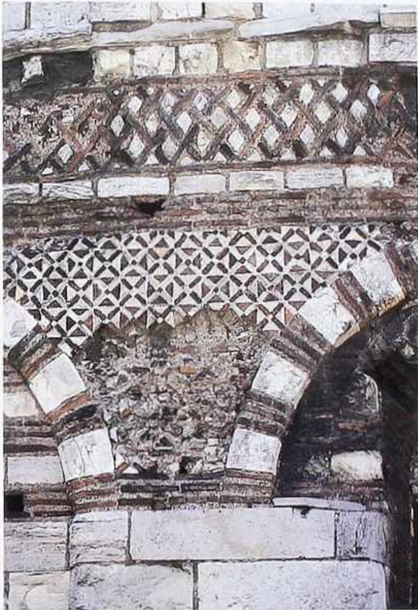
WA-286 Ancient arcade. Top to bottom: roughly squared stone; diaper brickwork; courses of stone and Roman brick, weathered tile with substructure, brick-and-stone arches; coursed-ashlar stone
