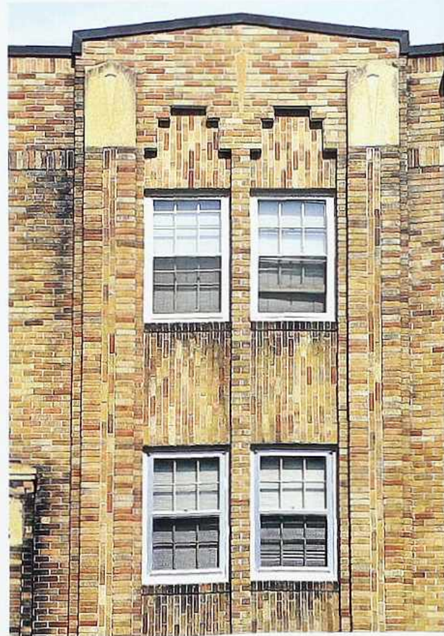
WA-184 Idiosyncratic collection of stacked bond and horizontal and vertical running bonds on pilasters and spandrels; rowlock window sills
