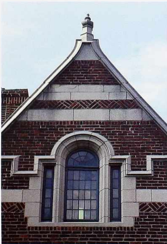
WI-96 Fanlight in Palladian window with fixed leaded lights and stone frame
