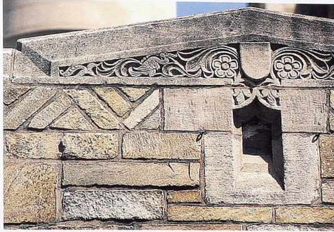
WA-86 Sandstone and quartzite in coursed ashlar below herringbone pattern; Indiana limestone ornamented cap
