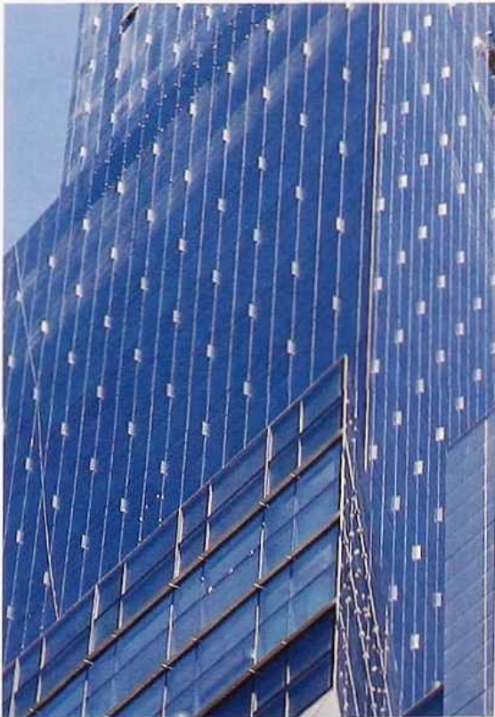
FA-38 Fully glazed curtain wall, shading louvers visible at lower level. Projections may be structural bracket system or ornamental
