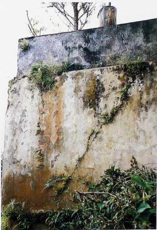
WA-262 Weathered whitewashed mud-stucco with invasive tropical vegetation on garden wall
