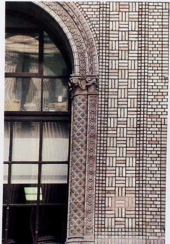
WA-204 Bands of decorative brickwork. Left to right: terracotta arch, stacked header rows, basket-weave, stacked header rows, English bond
