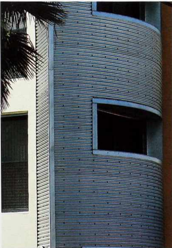
FA-21 Painted curved corrugated metal panels with visible fasteners and strip windows, modern residential building
