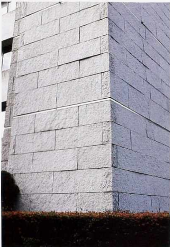
WA-133 Corner of split-face granite in shelf, running bond with metal banding, modern commercial building
