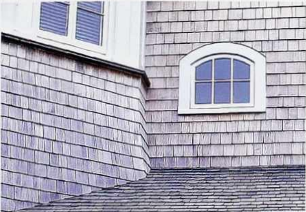
FA-49 Weathered Alaskan yellow cedar shakes in common coursing and segmental arch window, corner and roof detail
