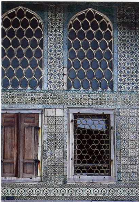
FA-70 Glazed patterned tiles around square windows with metal grille and wood shutter and ogee windows with grille, Turkey
