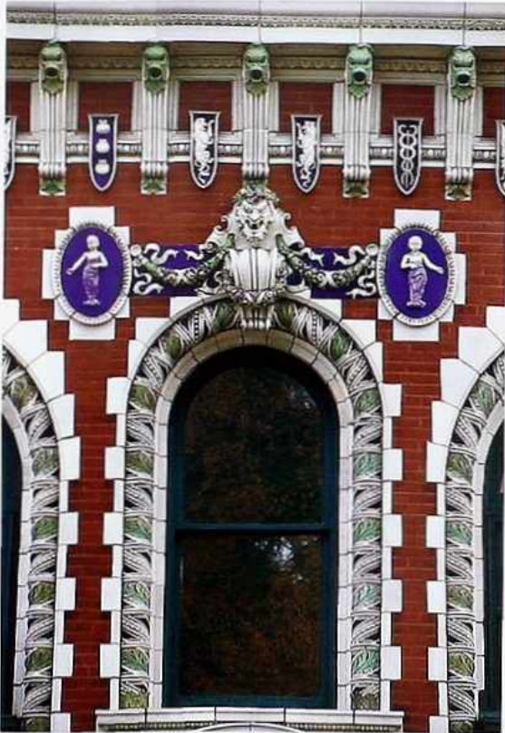
FA-59 Brick facade with polychrome glazed ornamental details: bracket cornice, cartouches, garlands, ancon, and rope molding around semicircular windows
