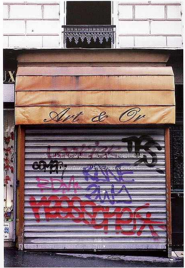
DW-53 Rolling galvanized-metal security door with graffiti
