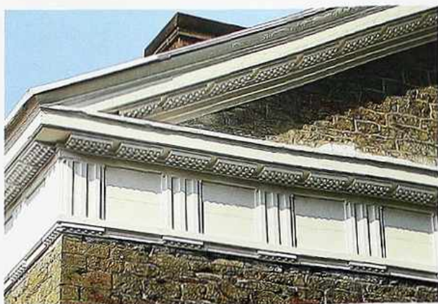
OM-86 Triglyphs with guttae alternating with plain metopes; mutules with guttae in the soffit
