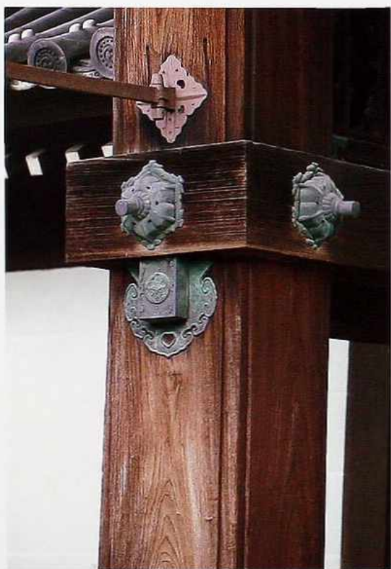
CP-107 Intersection of post and beam. Post appears to go directly through a mortise and is held in place by decorative tie irons
