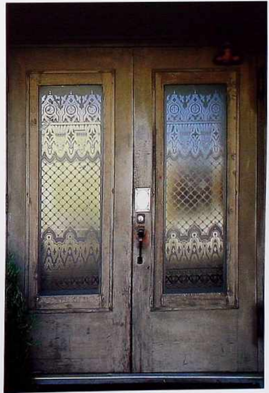
DW-22 Weathered wood double doors; single glass panels frosted and etched with zigzag and diaper patterns
