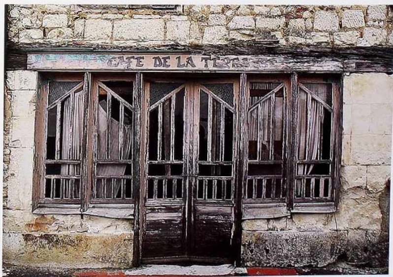
DW-106 Café entry in ruins: wood-paneled double doors with lights flanked by wood-framed windows
