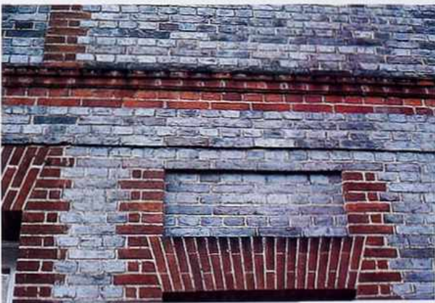
WA-173 Jack-arch window and dog-tooth course of contrasting brick in English bond wall with recessed panel
