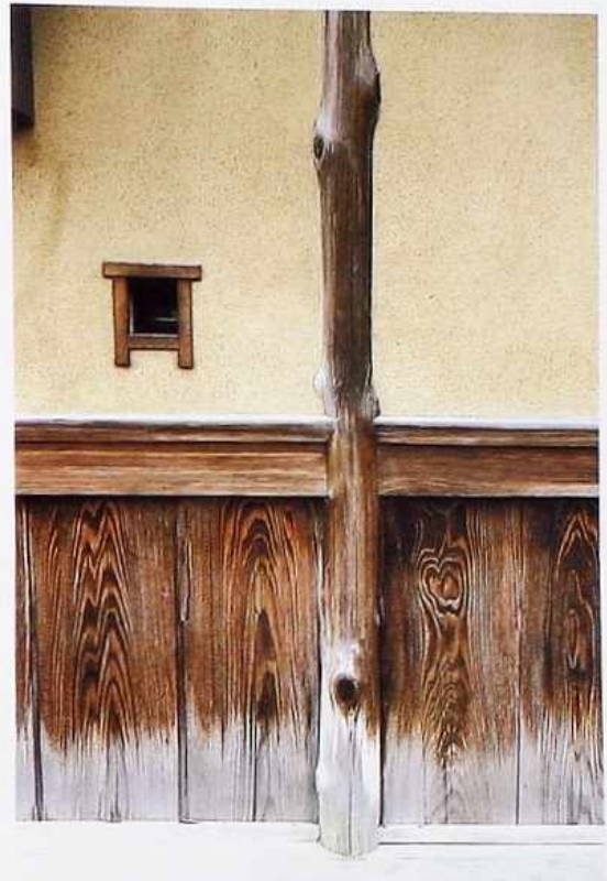
WA-279 Post-and-beam construction with stucco and wood-plank infill; partially dressed timber post, traditional Japanese building
