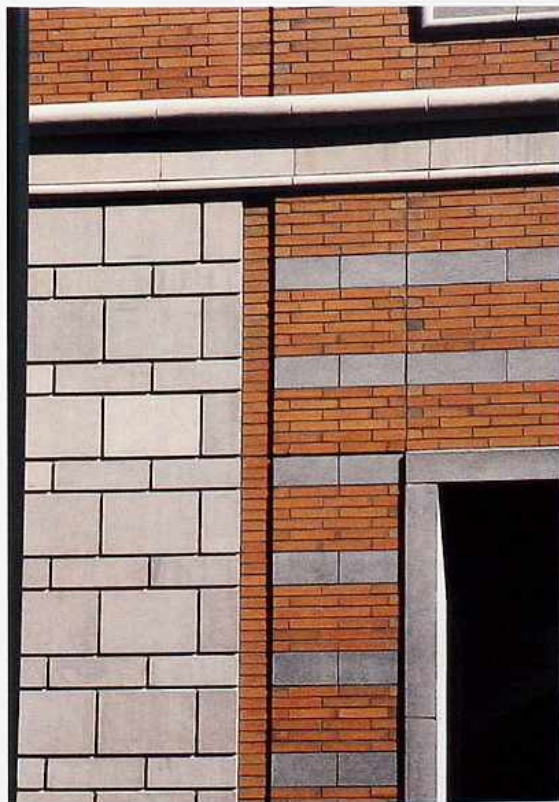
WA-295 Brick in running-bond bands with stone or pre-cast concrete, modern commercial building
