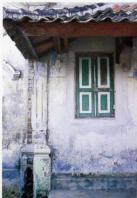
FA-95 Weathered painted stucco over brick
