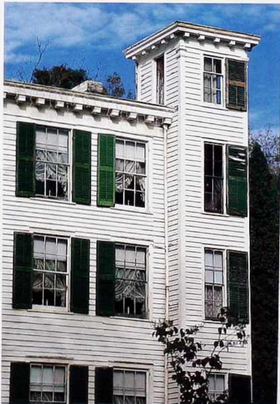
WA-34 Painted clapboard and block modillion cornice on corner tower, Italianate house
