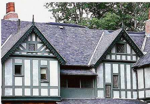
CR-95 Half-timber wall gables with scalloped bargeboard flanking shed roof and flashing in roof valleys
