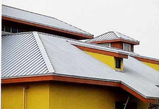
CR-101 Shed-roof dormer on metal hipped roof with standing seams, modern house
