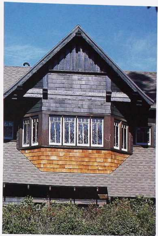
CR-90 Three-sided roof dormer with windows and wood beam spanning gable roof, Arts and Crafts cedar-shingle house
