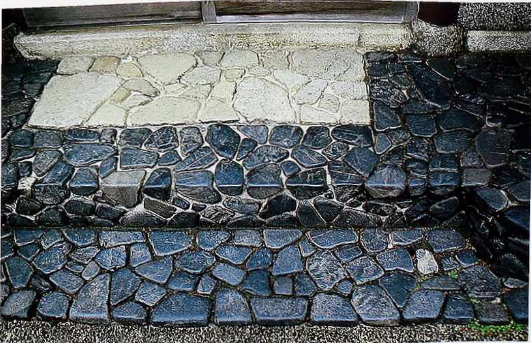
FP-42 Small, split, polished fieldstones set in concrete and bordering light-colored flagstone, forming steps
