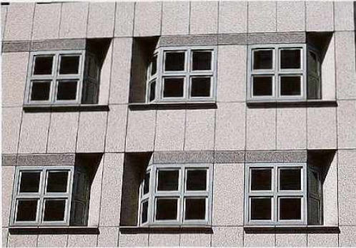
WI-160 Stone spandrels dividing recessed square metal fixed windows, modern commercial building
