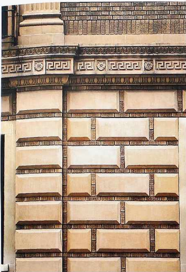
WA-290 Rusticated stone blocks in running bond, surrounded by brick; egg-and-dart pilaster cap and molding, with relief ornament band between stories
