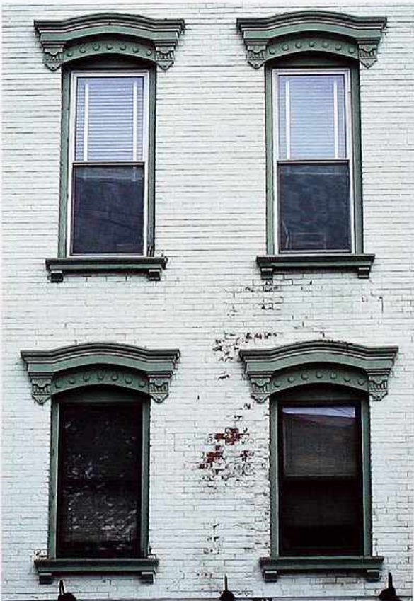
WI-109 Flat trim echoing arch profiles of window openings, 19th-c. American mixed-use building
