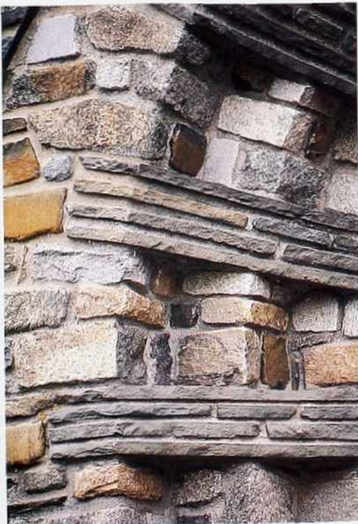
WA-91 Roughly squared stone in random ashlar wall with flagstone voussoirs in compound arch
