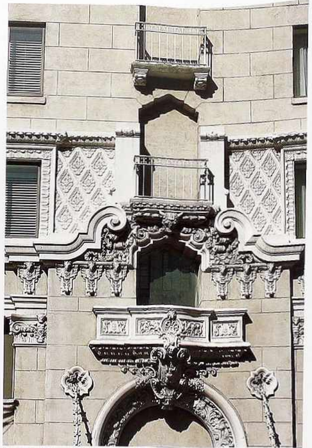
FA-113 Balconies over portal, broken pediment, and ornate details on multistory masonry facade
