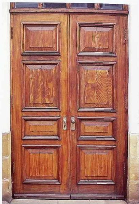
DW-5 Four panels, wood double doors with flush molding and raised panels
