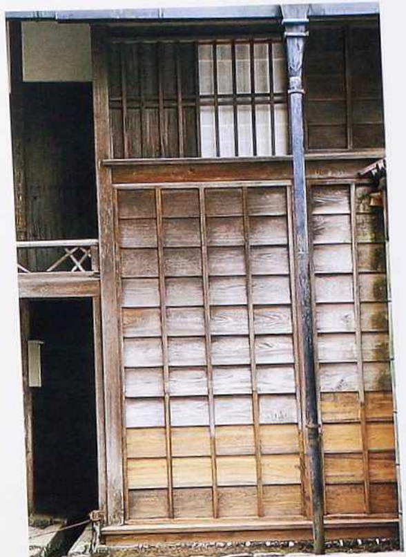
WA-41 Timber frame with infill of plain-sawn cedar planks; gutter with rainwater head
