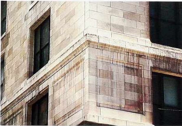
WA-103 Limestone in coursed ashlar with molding course and framed, recessed panels, water-damage weathering
