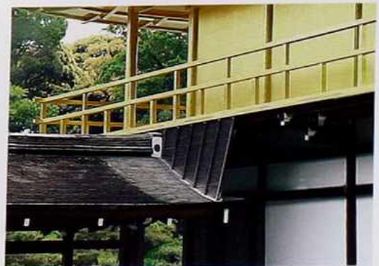
CR-114 Eave of shed roof connected to balcony to shelter courtyard walkway, traditional Japanese house
