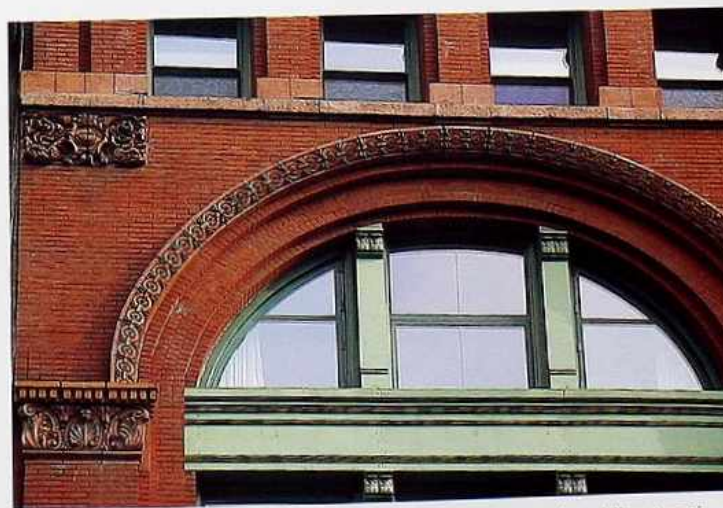
CP-161 Windows in semicircular arch; extrados with carved molding terminating at capitals
