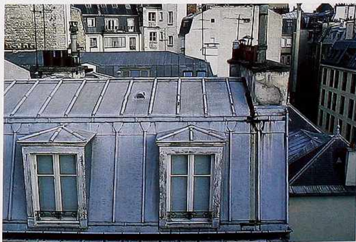
CR-29 Sheet metal with batten seams on gambrel roof and dormers, 19th-c. French apartment house
