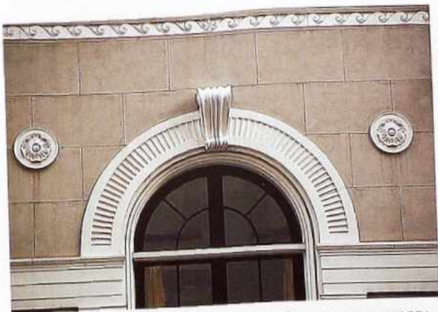
CP-141 Semicircular arch with an ancon keystone on masonry running-bond wall with Vitruvian scroll trim and rosette medallions
