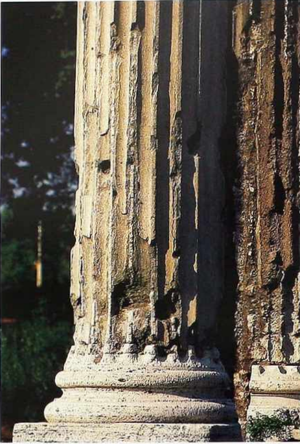
CP-58 Heavily weathered marble ancient Roman fluted column with Attic base
