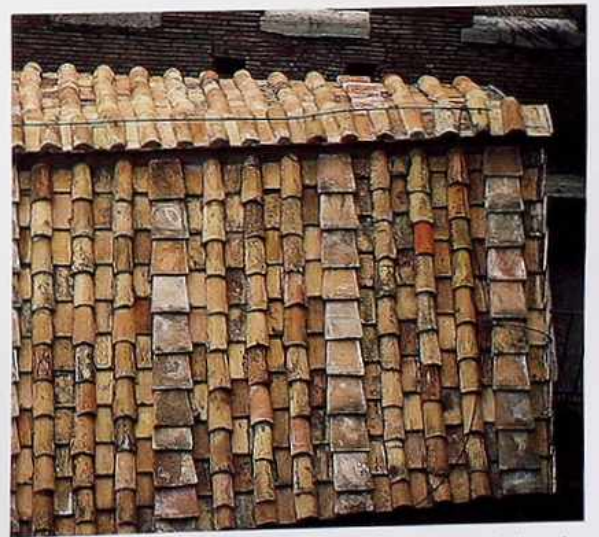
CR-43 Weathered terracotta mission and flat tiles on shed roof
