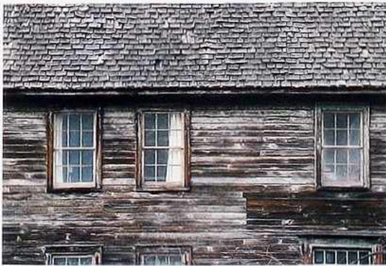
WA-24 Unpainted clapboard showing evidence of repair, with double-hung windows, American colonial house
