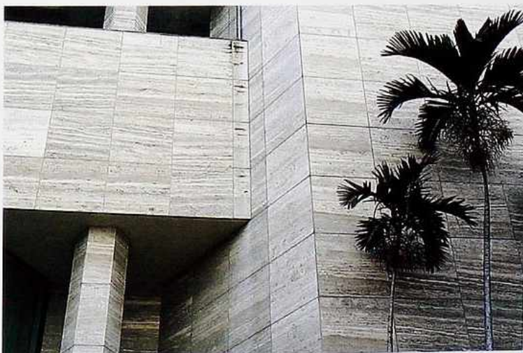
WA-130 Inside and outside corners of end-matched travertine veneer on walls and post, modern commercial building
