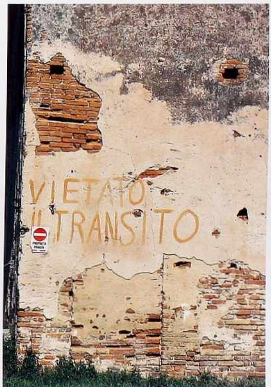
WA-263 Weathered stucco with concrete patches, graffiti, and exposed structural brick and stone
