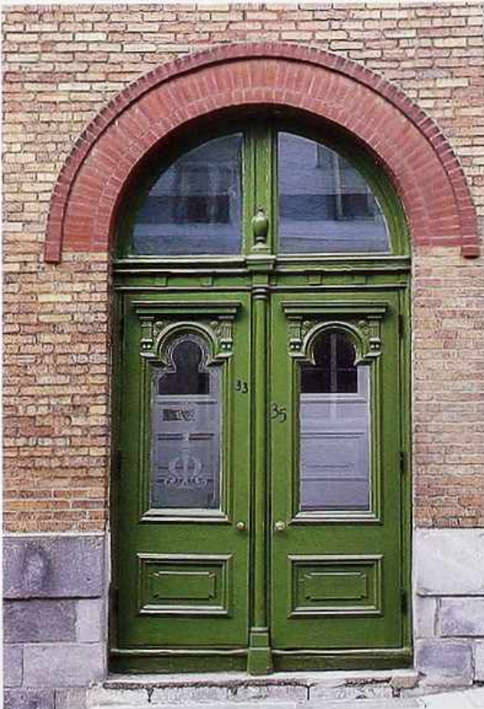
DW-21 Wood double doors with glass upper panels and flush-molded lower panels; split transom light in segmen-
