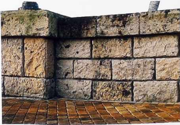
WA-78 Split-faced and rusticated Mexican volcanic stone in running bond, footbridge wall
