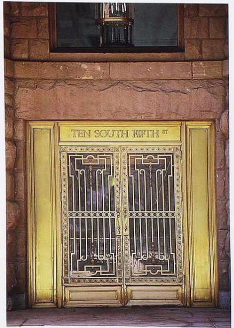
DW-50 Brass double doors; full glass behind ornate brass grille; brass panels flanking doorframe
