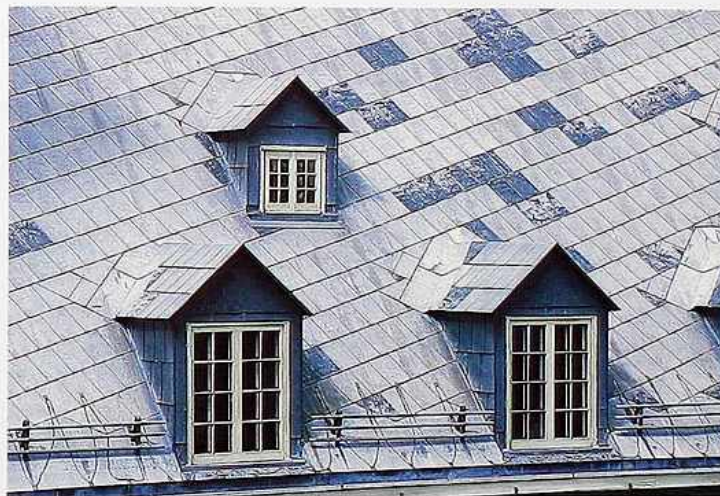
CR-28 Sheet-metal shingles with flat seams on roof and dormers; pipe-style snow guard on lower edge
