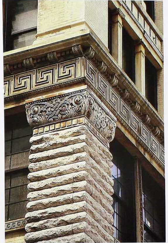
OM-83 Top to bottom: modillion band; frieze with Greek-key pattern; foliated arabesque capital; banded neck; rusticated corner pier
