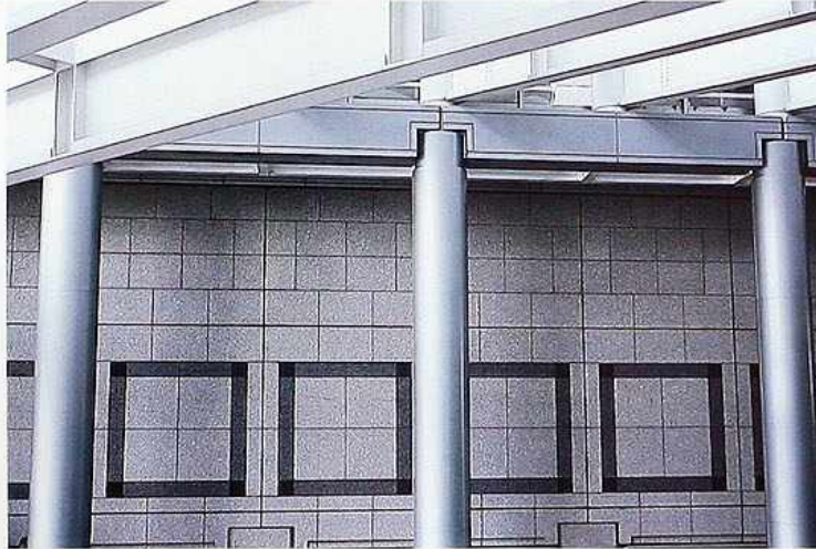
CP-138 Steel frame with metal-clad column and beam beneath exposed riveted plate girders, modern commercial building
