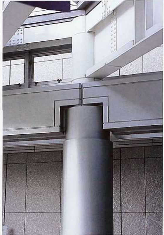
CP-123 Detail of steel frame with metal-clad column and beam beneath exposed riveted plate girders, modern commercial building
