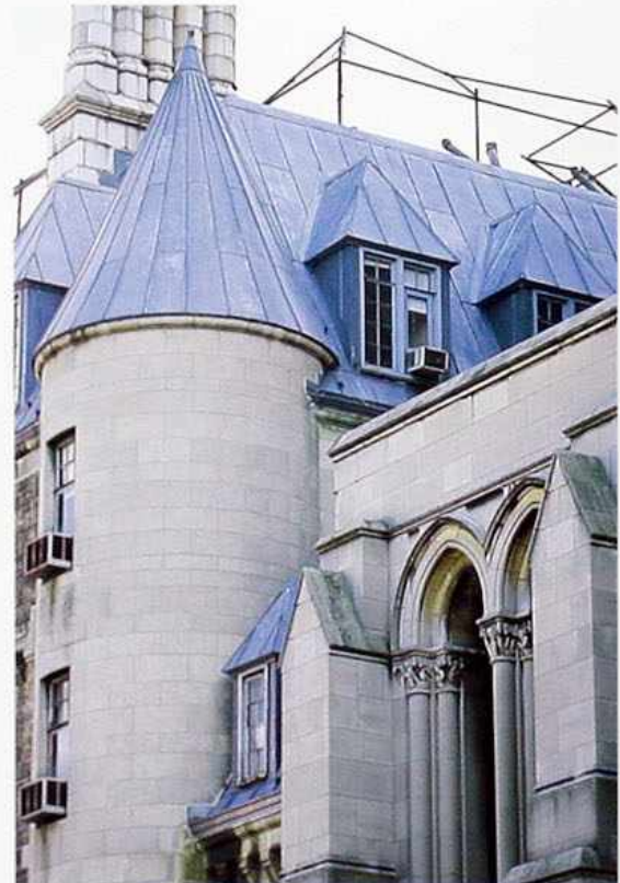
CR-33 Sheet metal with standing seams on conical turret roof; hipped roof and hipped roof dormer, 19th-c. chateau-style hotel
