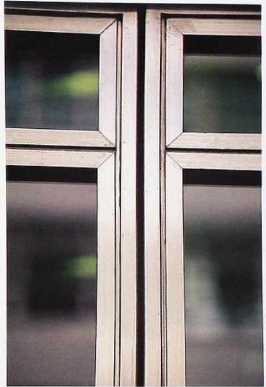
WI-6 Fixed window with stainless steel muntins and mullions, modern commercial building
