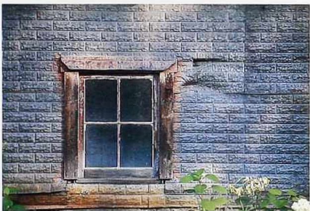
FA-3 Weathered stamped-tin sheathing in faux stone pattern
