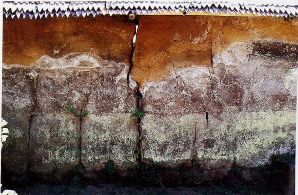
WA-253 Weathered tinted mud stucco revealing rammed mud wall
