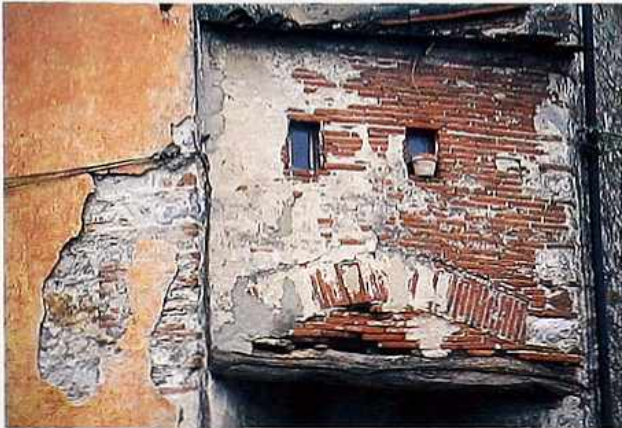
WA-256 Weathered colored stucco revealing timber lintel, scratch coat and structural stone, and Roman brick
