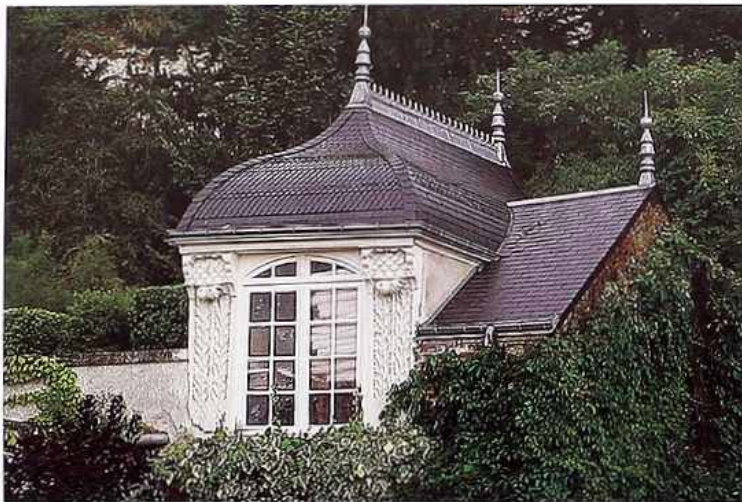
CR-134 Ogee slate roof adjacent to gable roof, both with metal ridge ornamentation
