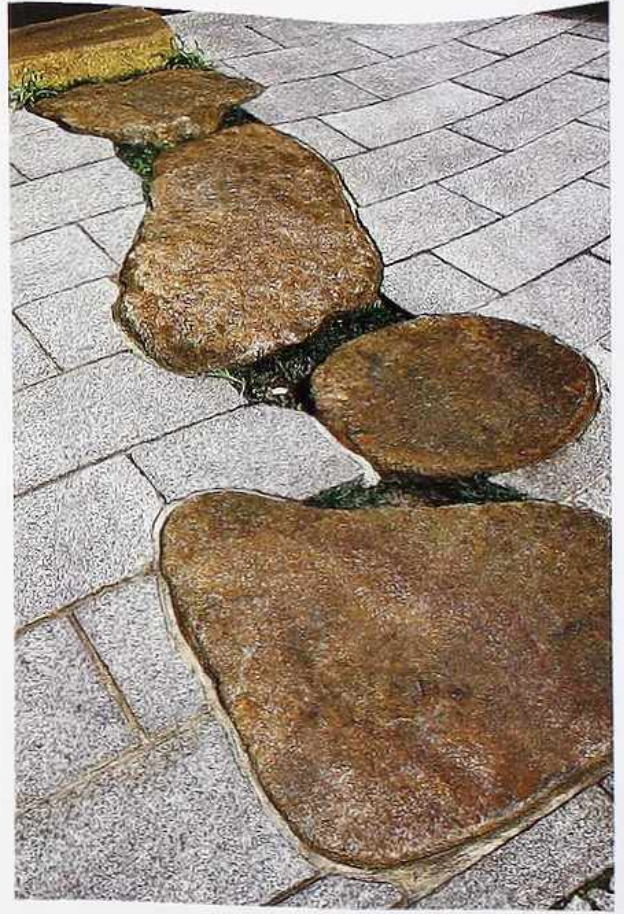
FP-41 Split, polished boulders between squared and textured paving stones in running bond, urban public space
