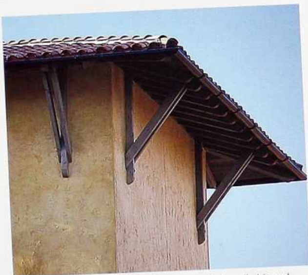
CR-107 Wood eave brackets supporting mission-tile hipped roof, American Southwestern mission-style house
