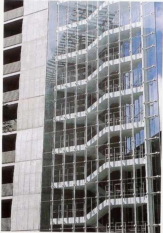
FA-33 Curtain wall around a stair tower with glass panels secured at corners by a bracket system and seams sealed with silicone
