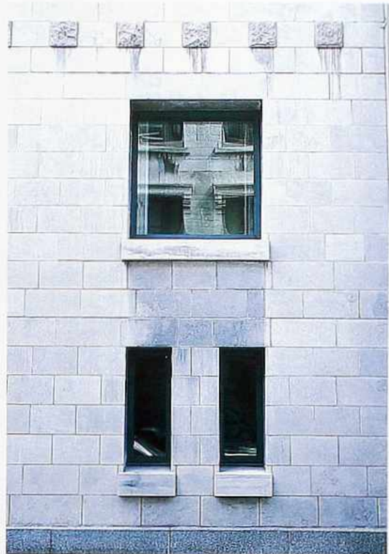
WA-139 Stone in running bond with projecting window sills and rock-faced decorative blocks, modern commercial building
