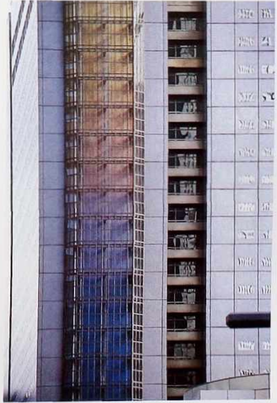
FA-39 Panelized cladding system with fully glazed curtain wall of light spectrum-producing glass or plastic enclosing elevator shaft
