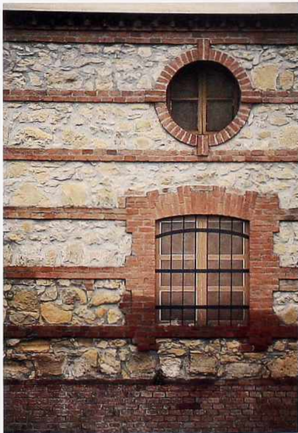
WA-288 Uncoursed rubble wall with brick-framed windows and brick belt courses; cambered arch window with trompe l'oeil grille and shutters
