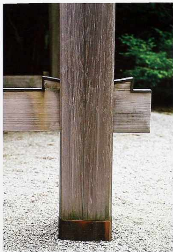
CP-108 Timber post with a horizontal brace attached by a double-wedged through-tenon joint with metal striping on the top
