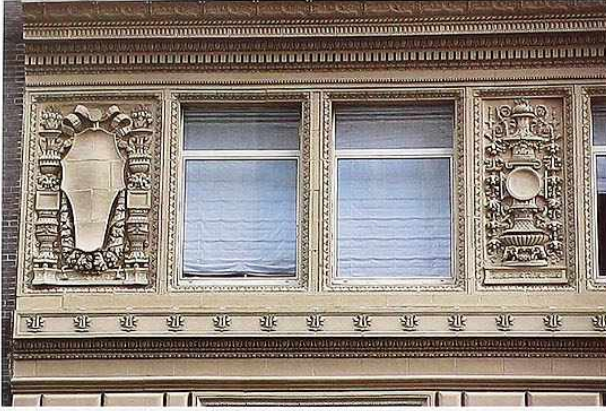
WI-126 Stone cartouches flanking upper-story windows with molded casings, replacement windows, early 20th-c. apartment house
