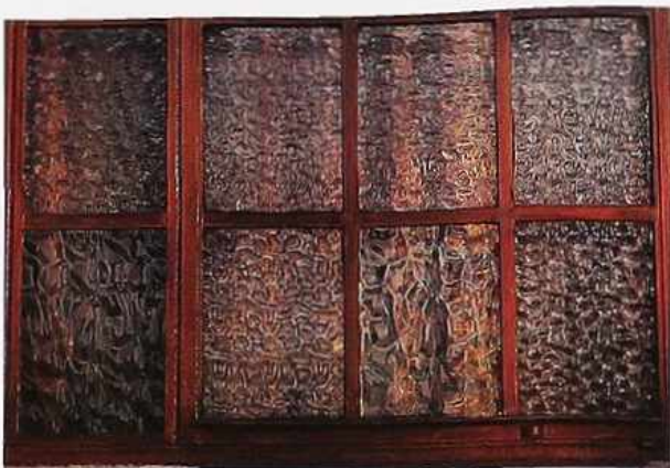
WI-11 Figured glass with flat metal muntins in a metal frame, industrial building
