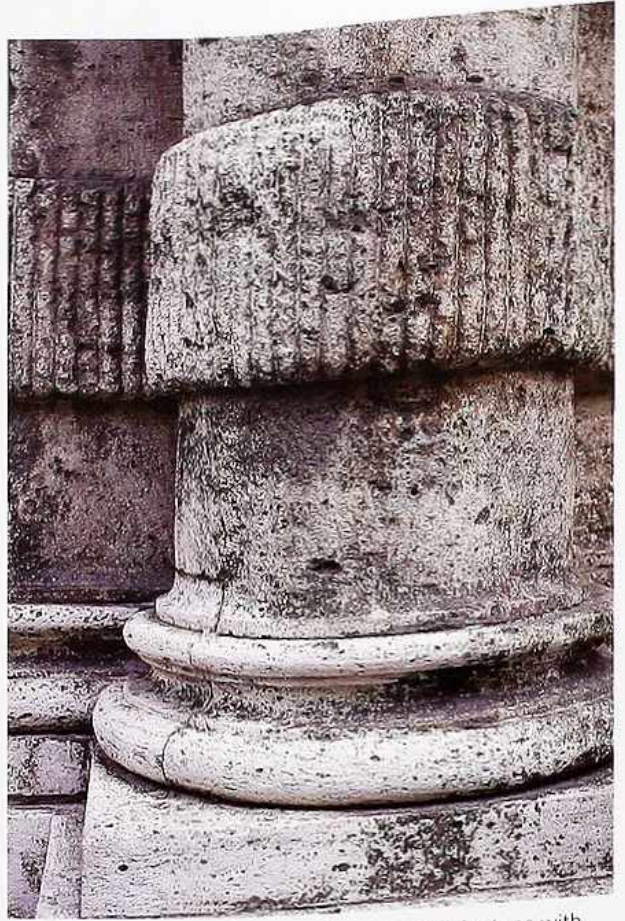
CP-32 Attic base of weathered column in volcanic stone with banded rusticated shaft
