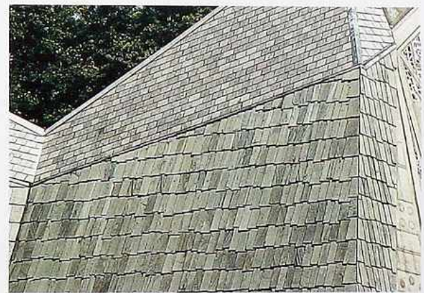
WA-129 Inside and outside corners of slate roof and cladding, modern commercial building
