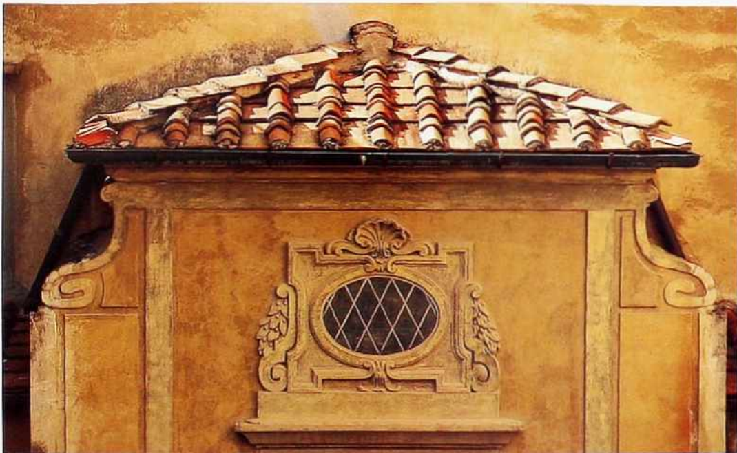
WA-250 Weathered colored smooth stucco surrounding oval window with grille and ornate frame; hipped tile roof
