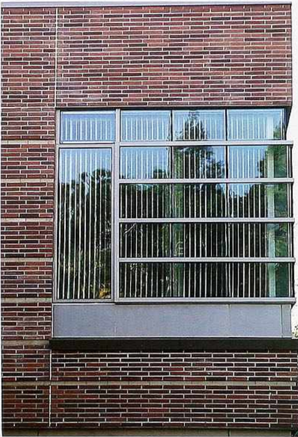
WI-86 Corner window: fixed lights with metal sashes, muntins, and mullions, modern commercial building
