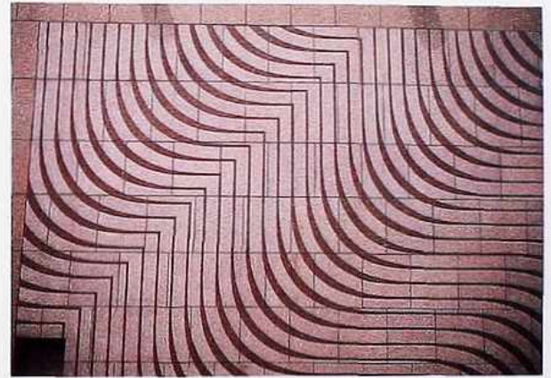
WA-69 Pink granite in running bond with polished and flamed finishes forming supergraphic, modern commercial building
