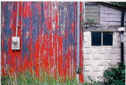
FA-100 Weathered painted vertical board-and-batten wall and adjacent masonry structure
