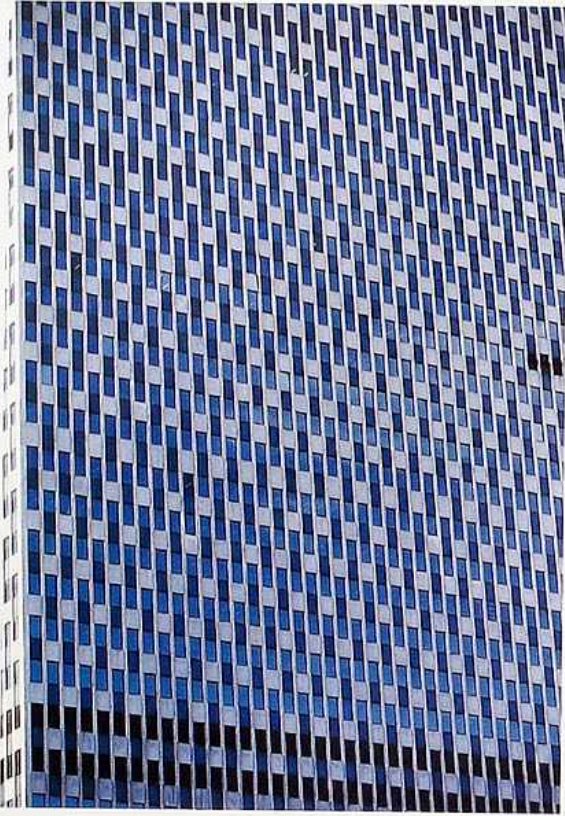
FA-32 Cladding system of staggered spandrel elements, probably pre-cast concrete and glass
