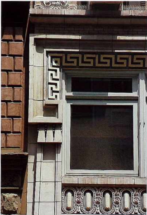
OM-55 Crossette surround with Greek-key motif, terminated with three guttae; framed lozenge design in spandrel panel
