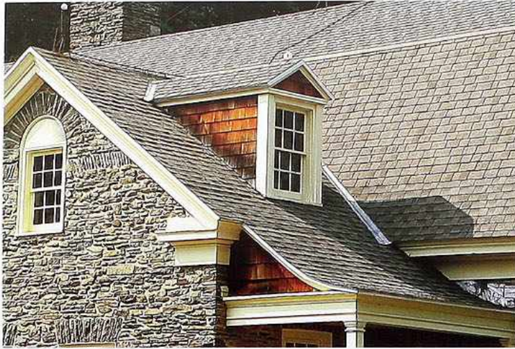
CR-86 Shingled roof dormer above flared eave covering porch; stone gable-end wall
