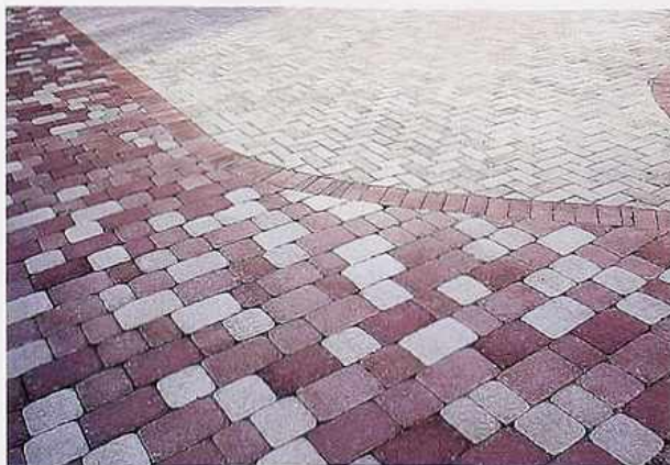
FP-89 Flexible paving: concrete pavers in herringbone pattern (top), with border course; tumbled random-size concrete pavers in running bond (bottom), urban public space
