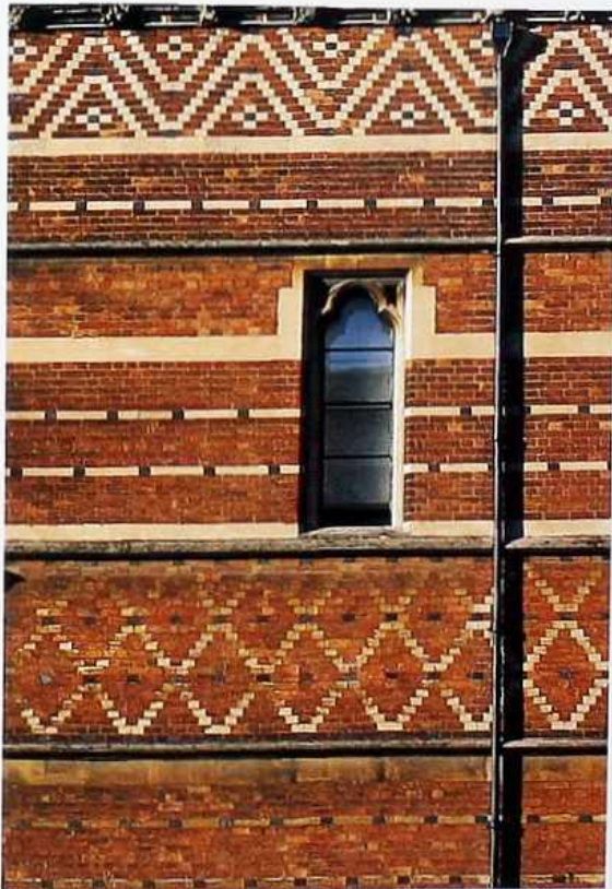
WA-203 Bands of decorative brickwork. Top to bottom: chevron, horizontal banding, diaper-work
