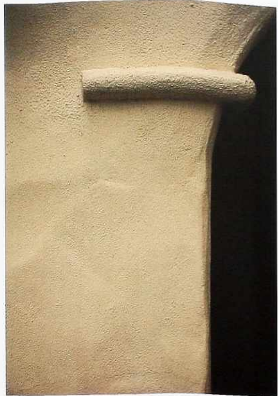
WA-231 Detail of arched opening with impost-like molding, stucco over adobe, American Southwestern mission
