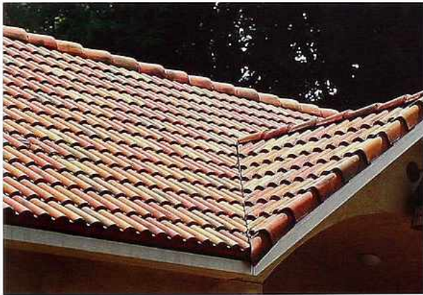
CR-51 Detail of mission tiles at junction of gable and main roof
