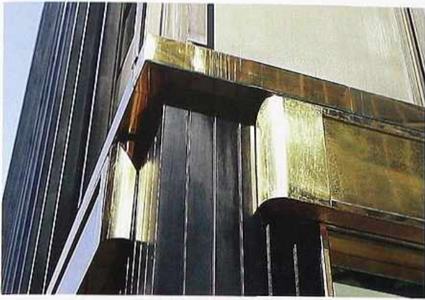
OM-73 Metal cladding suggesting a frieze and cornice, "entablature" broken at corner to reveal the soffit of the "cornice," modern building facade
