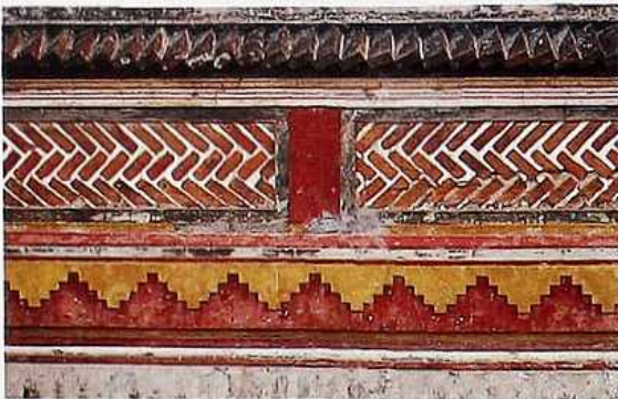
WA-266 Courtyard wall. Top to bottom: cast-concrete coping; saw-tooth brick course; light-colored stone, herringbone-bond brick in concrete frame; painted brick; stone base
