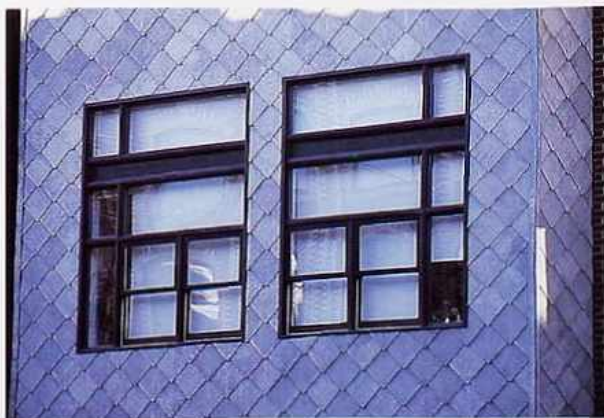
WI-102 Top to bottom: rectangular transom lights; fixed lights; pairs of one-over-one double-hung windows and fixed side lights, modern apartment house
