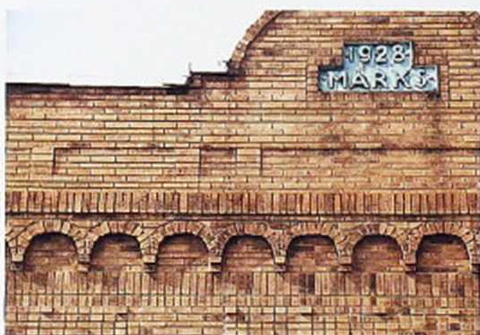
WA-161 Parapet wall in running bond with blind semi-circular arches and corbels below soldier course
