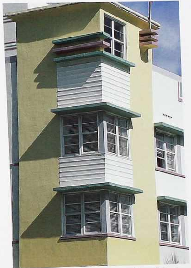
WI-91 Corner windows: single-hung sashes with fixed upper lights, Art Deco apartment house
