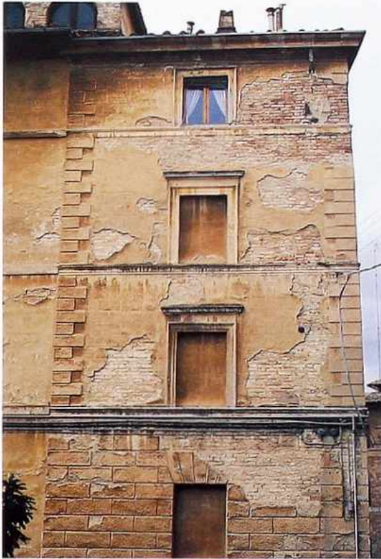
WA-260 Weathered stucco exposing structural brick and stone. Original plasterwork included faux-stone quoins and blocks in running bond
