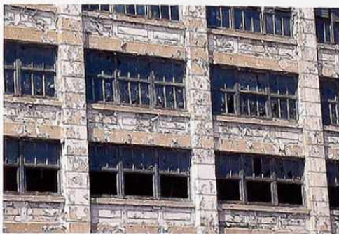
FA-98 Peeling paint on poured-in-place concrete frame with scored simulated masonry joints
