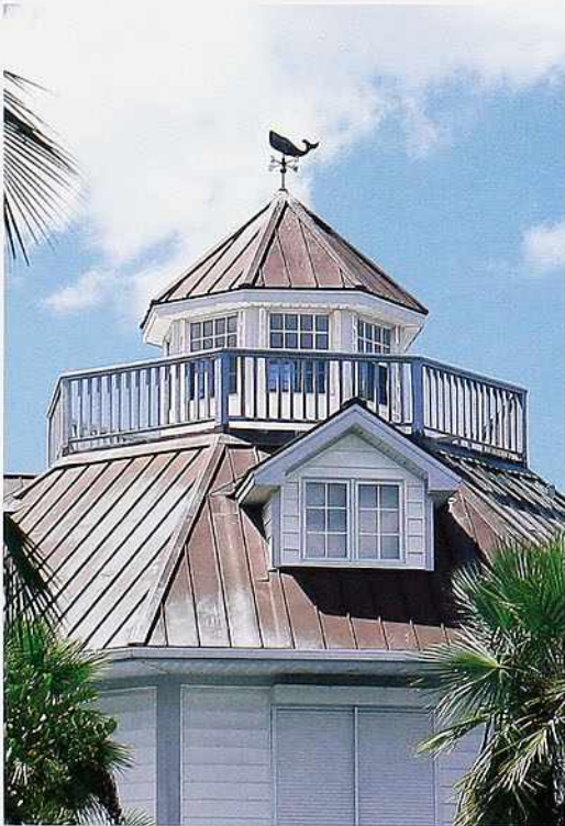
CR-128 Octagonal painted standing-seam metal roof with widow's walk and gabled roof dormer
