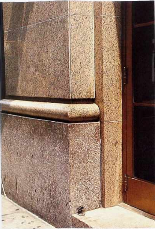
WA-89 Honed granite veneer with solid granite base and bead molding beside granite door casing
