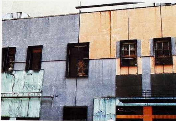
FA-24 Painted and patinated metal panels with lapped seams, modern commercial building
