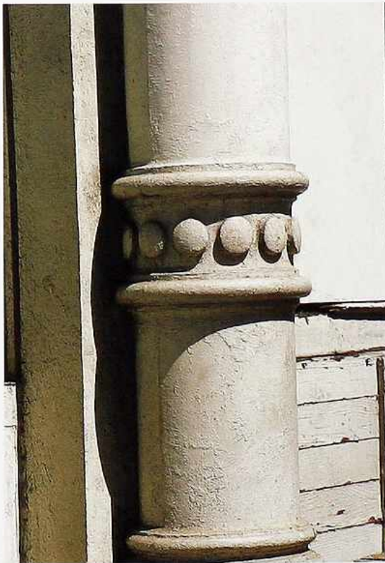
CP-63 Cast-iron column with Doric/Tuscan base and a band of round ornaments on round pedestal with Attic base
