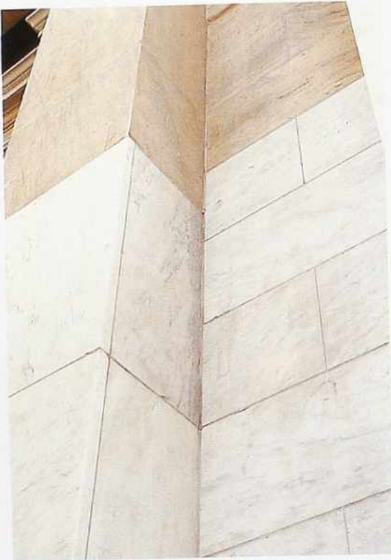
WA-97 Inside corner of honed-veiner marble in running bond, bottom recently cleaned
