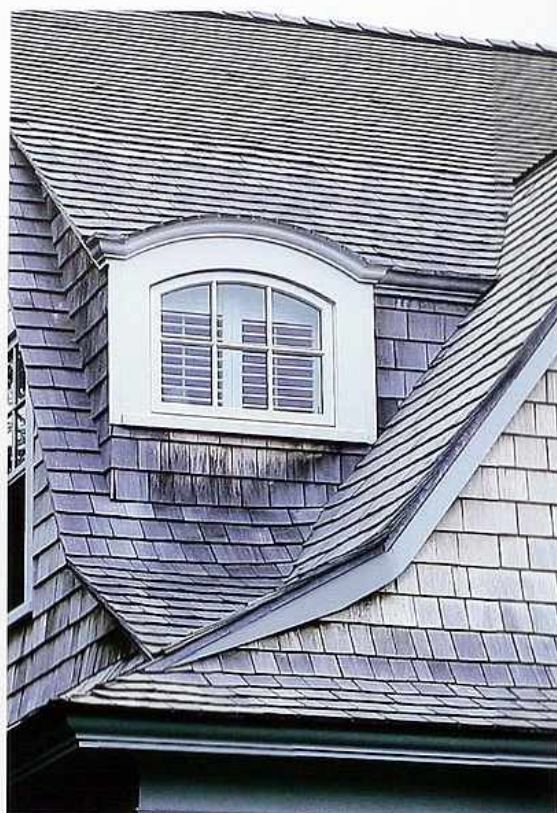
CR-65 Alaskan yellow cedar shingles; roof valley at intersection of gables; traditional American house.
