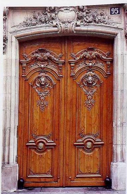
DW-8 Two panels, double doors with carved bas-relief ornament and trompe l'oeil wood finish. Cambered stone arch doorway with cartouche keystone
