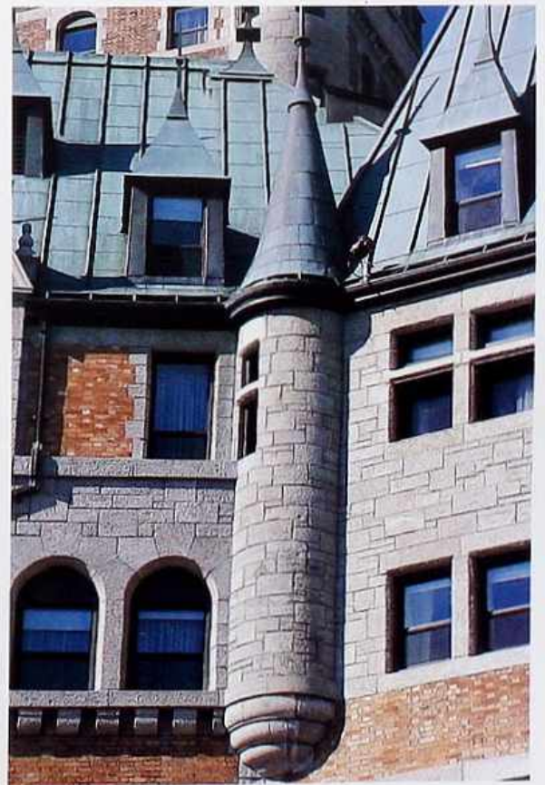
WA-289 Coursed ashlar on inside-corner turret with corbelled jetty and adjacent upper story; remaining walls of brick
