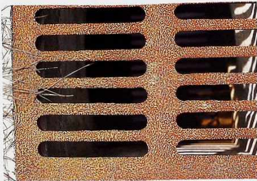
FP-115 Rusting cast-iron drain grate
