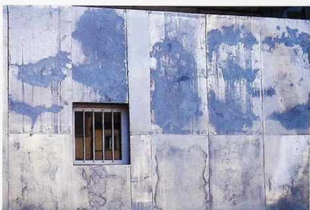
FA-6 Weathered flat metal panels with visible fasteners, probably lapped, exterior wall of industrial building
