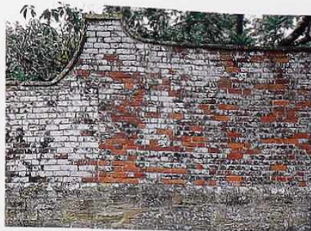
FA-99 Peeling paint on brick garden wall with stone base
