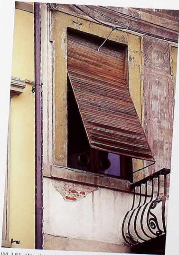
WI-181 Weathered metal awning
