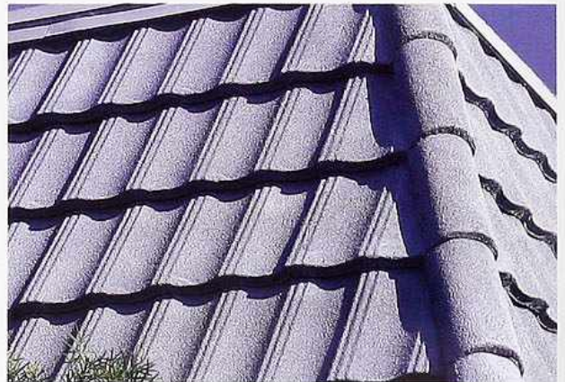
CR-47 Cast concrete pantiles on hipped roof with concrete ridge tiles on hip
