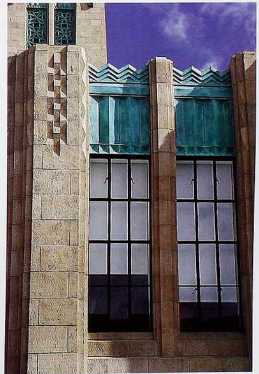
WI-149 Copper panels capping windows with metal sashes in recessed stone casings, 20th-c. commercial building
