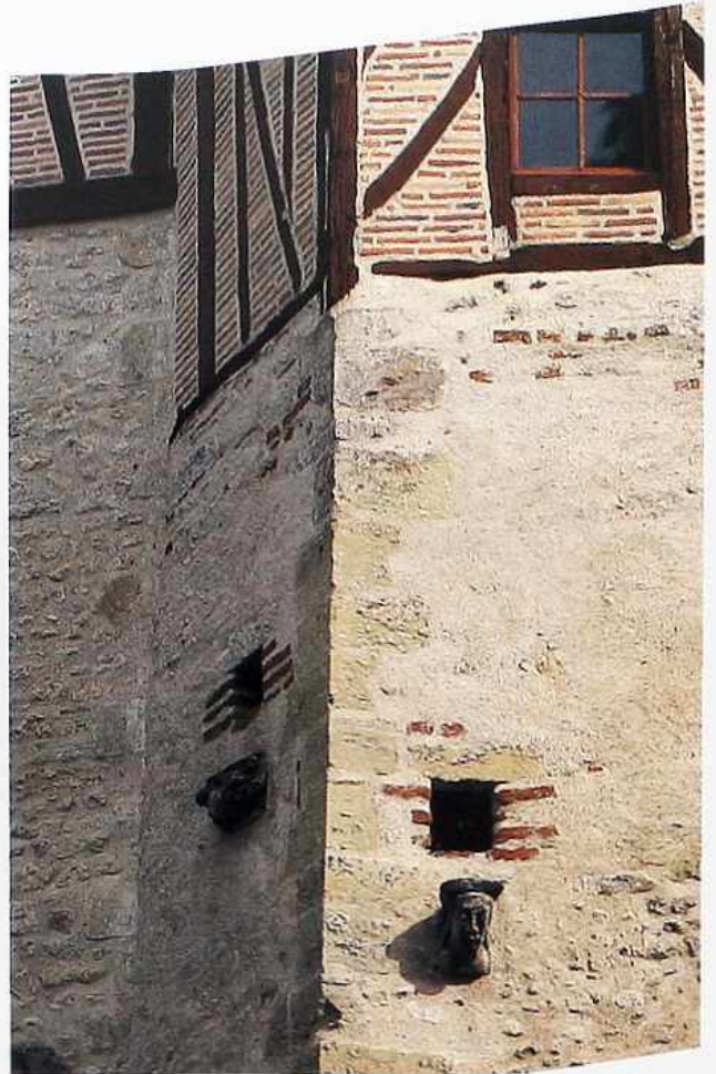
WA-291 Half-timber upper story with brick infill and stucco lower story with stone quoins
