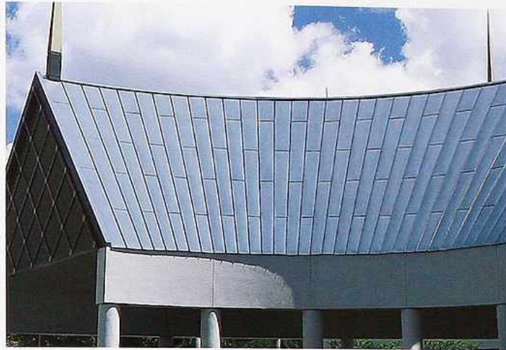
CR-27 Anodized aluminum or coated sheet steel with standing seams, curved gable roof, modern commercial building
