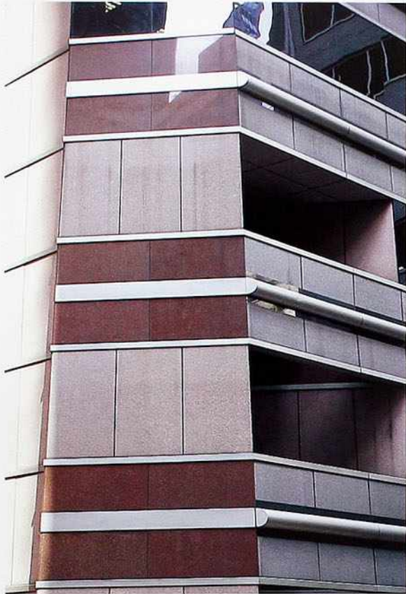
OM-79 Metal molding in a panelized wall system resembling an exaggerated bead molding flattened when it turns the corner
