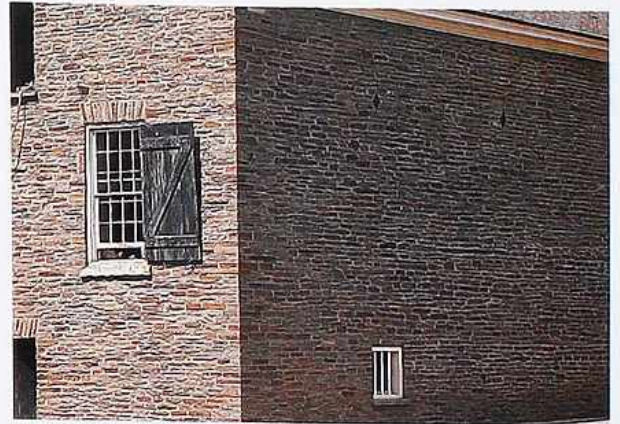
WA-102 Corner of coursed, random ashlar with anchor irons; window with jack arch
