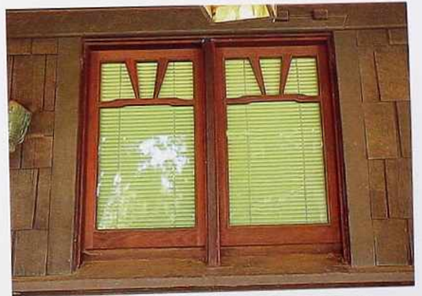
WI-28 Wood-framed awning windows with shaped wood muntins, Arts and Crafts house
