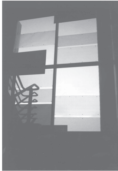
Figure 10.8 Installation of translucent panels in a grand staircase. The exercise gave an interdisciplinary team of design students (architects, interior designers, landscape architects) the opportunity to simulate a process of design, documentation, and construction with real-world time and budget constraints. Courtesy of Professor Nancy Clark Brown.
