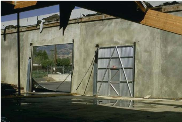
Figure 10. Separation of wall panels from roof diaphragm during 1971 San Fernando earthquake (NISEE, 2005)
