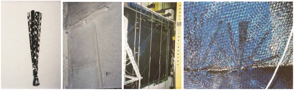
(a) FRP anchor (b) Anchor holes (c) Wooden Guides (d) Anchors in place
