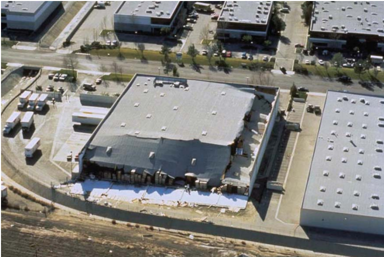
Figure 4. Damage to tilt-up warehouse during 1994 Northridge earthquake (EERI, 1996)
