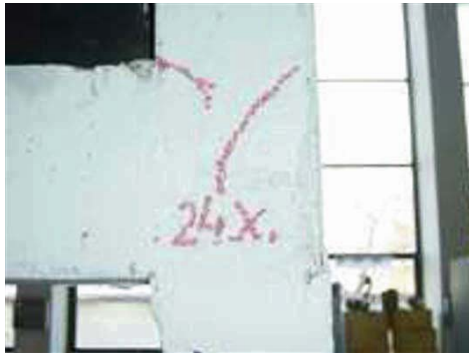
Figure 12. Small cracks in the column-beam joint
