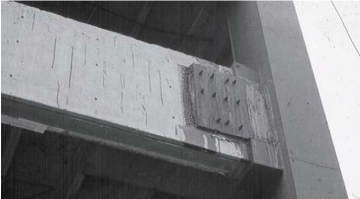
Figure 4. Detail of brace connection and column jacket
