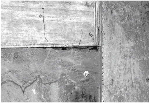
Figure 15. Beam/Column Joint Void
