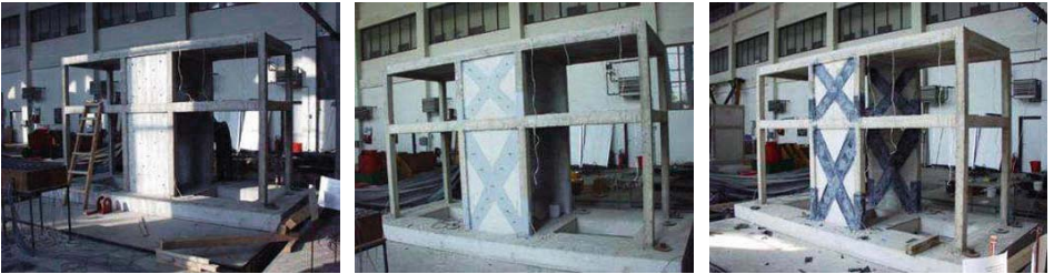
Figure 2. Phases of construction of Specimen 2; (left)-anchorage holes are drilled; (right)-anchor dowels are placed; (right) completed model with added carbon fibers
