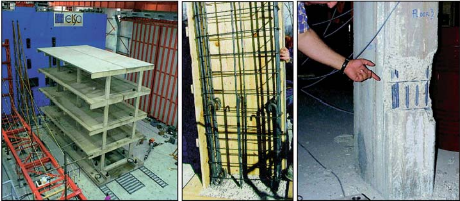
Figure 3. Four-storey R/C models: a) General view of the mounting phase (left), b) Stocky column reinforcement at the 3 rd storey (lap-splicing) (centre), c) Column failure at the 3 rd storey at the bars termination zone during the BF975 test
