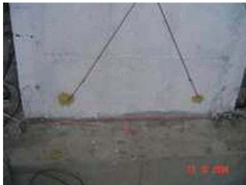
Figure 10. A major crack infill/foundation
