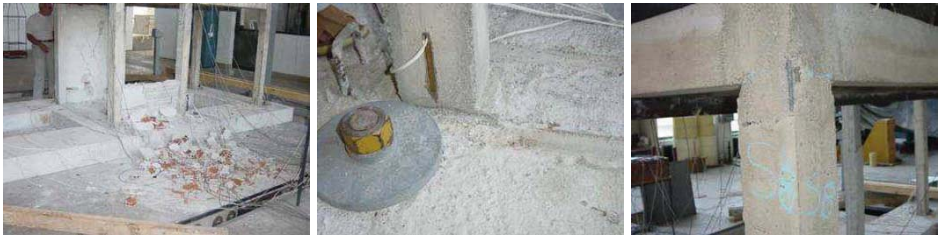
Figure 14. Specimen 1 at the end of test: Shear-slip failure between the concrete elements and masonry infill wall due to poor connection (left); brittle failure between the columns and foundation due to inadequate stirrup lap-splice-length (middle); and crushing and spalling of concrete near beam-column joints(right)
