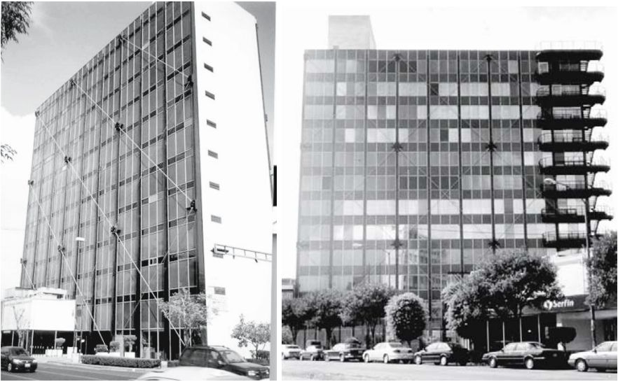
Figure 18. Views of cable bracing on 10-story structure
