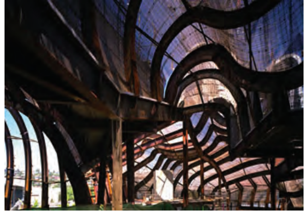
Figure 4: Structural frames in Frank Gehry's Experience Music Project in Seattle, produced by contouring (Kolarevic 2001).
