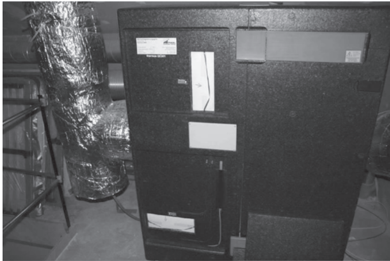
Figure 5.8 Heat-recovery ventilation unit in the loft space
