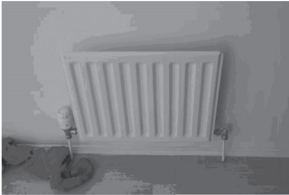
Figure 5.5 Radiator in a low-energy home
