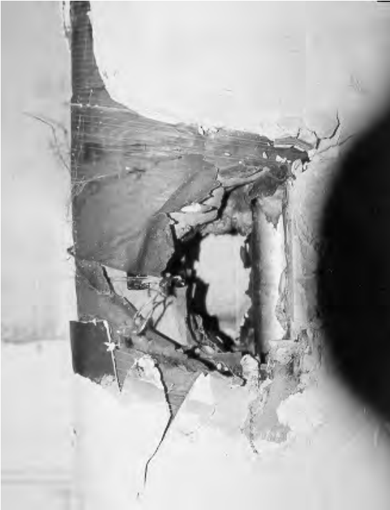
Figure 11.3 Defective insulation of the distribution pipe
