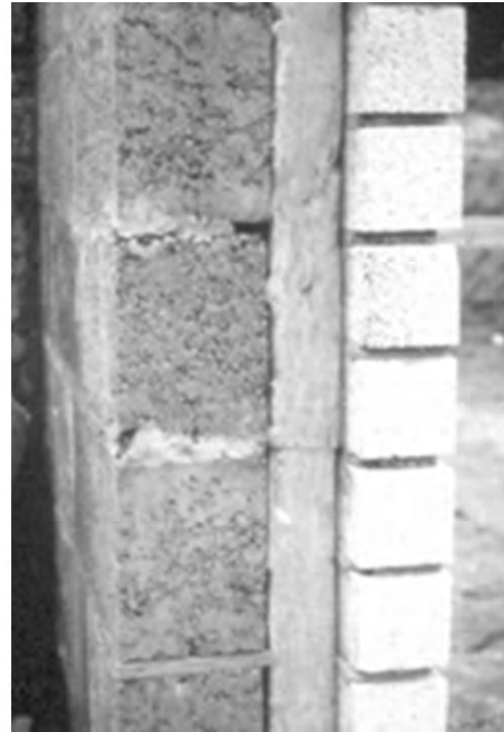
Figure 16.6 Example of two-stage rain protection: Cavity wall with water-repellent fibrous insulation touching the veneer; the inside leaf is still lacking its air-retarding plaster finish
