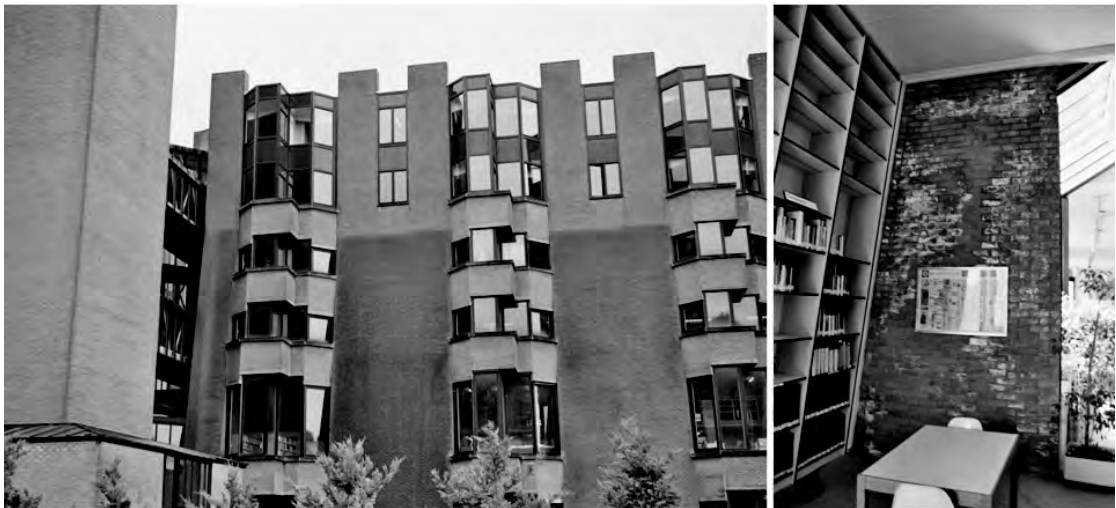
Figure 16.7 Building with rain penetration
