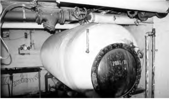
Figure 11.5 Hot water storage tank
