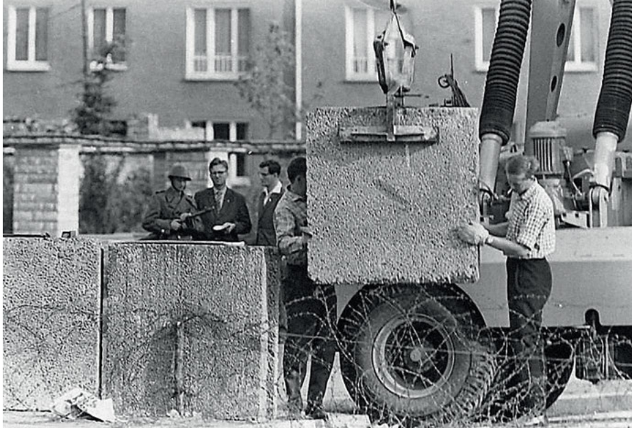
Fig. 4.1: Berlin Wall construction: cement blocks being lifted with a crane behind barbed wire (Germany)
