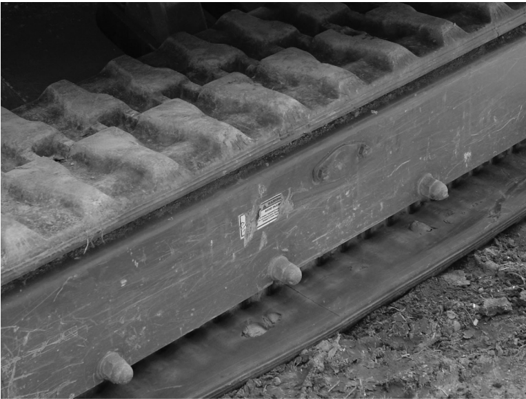
FIGURE 9.9B In this instance, a different location or different kind of warning “label” (that is, more permanent than a stick-on label) would have been a better choice.
