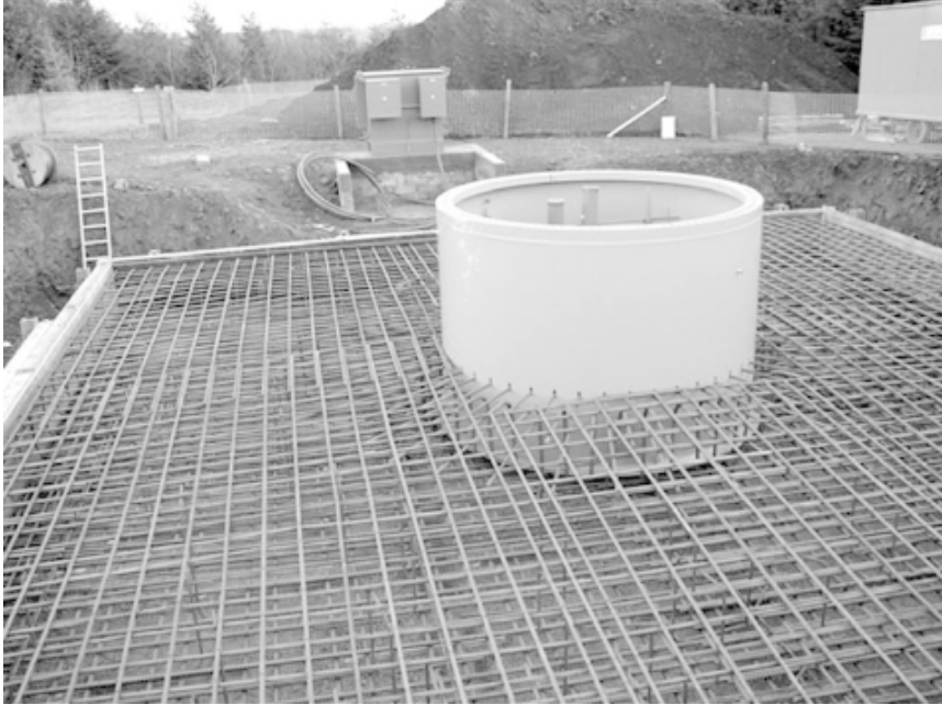
Figure 9.16 Stub tower foundation under construction for a Vestas V52. The steel 'can' is threaded with reinforcing bars and forms an integral part of the base once the concrete is poured. The bottom tower section is bolted to the flange ring at the top of the can.
