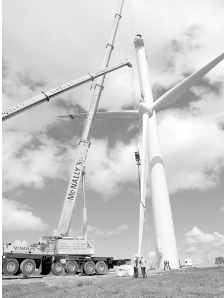
Figure 9.26 Main rotor lift for a Vestas V52. A tailing crane (out of picture) is steadying the rotor. Single-crane rotor lift is also possible using a proprietary turning mechanism under the crane hook.
