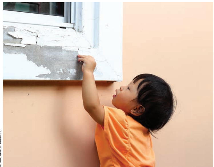
> PHOTO 16-8 Old, lead-based paint threatens the health of an exploring child.
