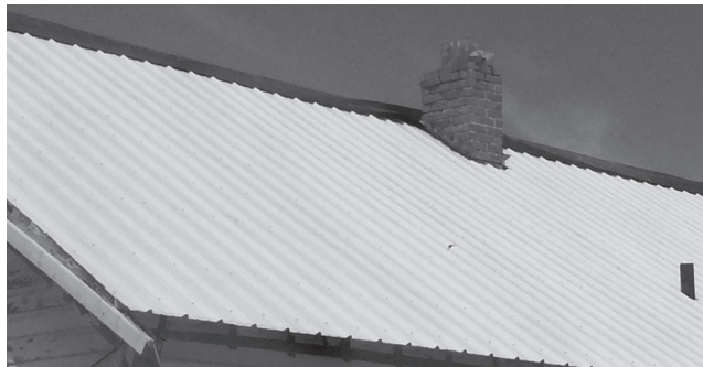
A Depression-era home in the middle of a remodel. Note how the chimney's condition remains untouched.
