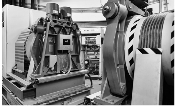
Figure 2.4 Dead Load—elevator machinery
