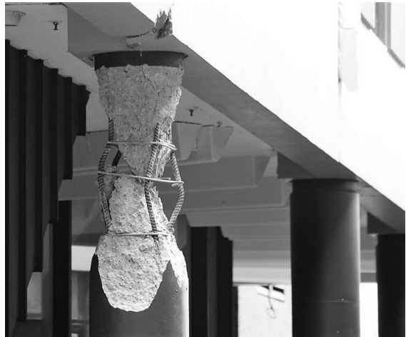
Figure 10.36 Outward Buckling of Vertical Reinforcing
