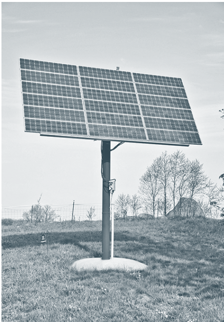
Figure 1.11. Ground-mounted solar arrays like this one accommodate numerous modules and can be oriented and angled to maximize production. Because they allow air to circulate freely around the modules, systems such as these stay cooler than many roof-mounted arrays and thus tend to have a higher output. Credit: Dan Chiras.
