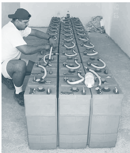
Figure 7.3. Lead-Acid Batteries for RE System. Lead-acid batteries are commonly used in renewable energy systems. Be sure to purchase deep-cycle batteries; keep them in a warm, safe place; recharge quickly after deep discharges; and equalize them periodically. Credit: Surrette Battery Company LTD.
