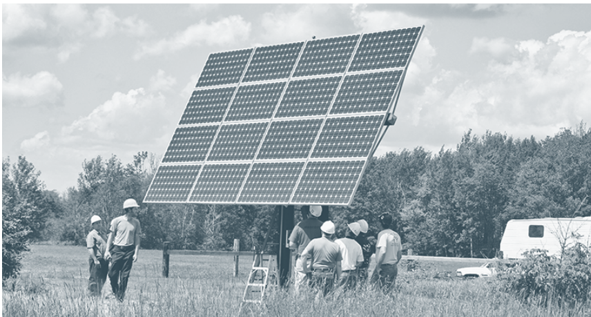
Figure 8.12. Tracking Array. This tracking array was installed by Dan and fellow students at a workshop in Minnesota sponsored by the Midwest Renewable Energy Association located in Custer, Wisconsin. Credit: Dan Chiras.
