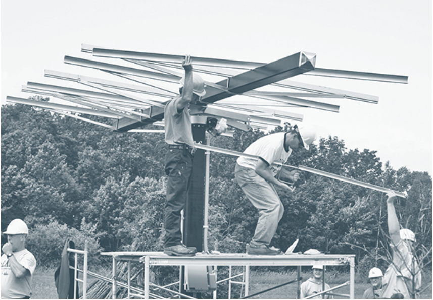
Figure 8.8. Pole-Mount Being Assembled. Students at MREA workshop installing rails on the strong back (center beam) on a pole-mount. Credit: Dan Chiras.
