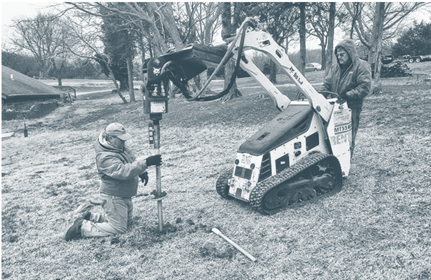
Figure 8.5. Steel Augers Being Installed. We use this machine or a skid steer equipped with an auger attachment to install augers to mount PV systems. One thing I like about this system is that it minimizes ground disturbance and makes for a much neater installation. Credit: Dan Chiras.
