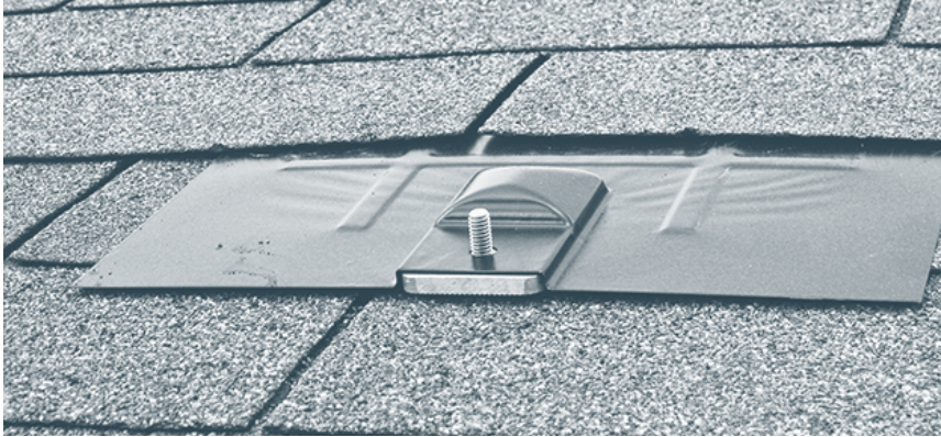
Figure 8.21. Mounting Kit with Flashing. We used this roof mount with flashing on a job on a steel company in Winfield, MO. Flashings such as this help reduce the chances of leakage, giving the homeowner and the installer a little more peace of mind. Credit: Dan Chiras.
