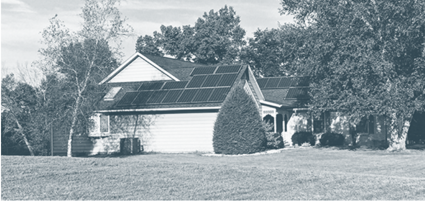
Figure 8.1. East-facing Array. Irresponsible and uninformed solar installers sometimes install PV arrays on east- and west-facing roofs (like the one shown here) under the misguided notion that this orientation will only reduce PV output by 15%. That’s not true for steep roofs like this one. This array, which faces due east, is in the shade shortly after solar noon each day. There are also several large shade trees east of the array that block sun part of the year. And, making matters worse, the east-west oriented roof of this house shades the lower part of the array on winter days when the Sun is low in the sky. Don’t make this egregious mistake. Credit: Dan Chiras.
