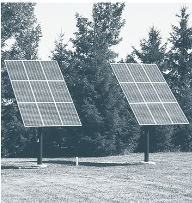
Figure 8.7. Pole-Mounted Array. Each array is mounted on a pole anchored to the ground and is installed at the optimum angle for its location. Pole-mounted arrays provide some flexibility in placing an array on a lot. Credit: Anthony Powell.
