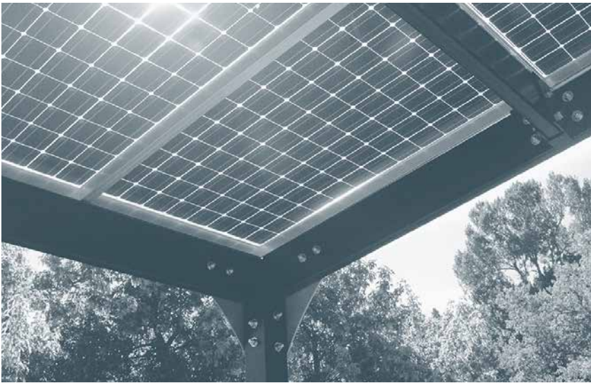
Figure 8.29. Solarscaping. PV modules can be used to create roofs of shade structures, a technique known as solarscaping . This photograph shows a portion of a carport made from PV modules by Lumos Solar. Credit: Lumos Solar.
