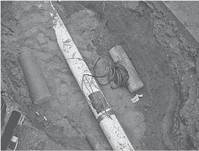
Figure 17.29 Ductile iron municipal water main protected with tape wrap and sacrificial magnesium anodes. Source: Reproduced with permission from P. R. Roberge, Handbook of Corrosion Engineering , 2nd edition, McGraw-Hill, 2012.
