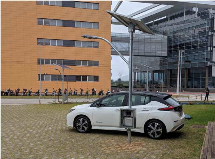
FIG. 11.16 Example of solar light system installed in Fotovoltaica/UFSC solar lab [66, 71].
