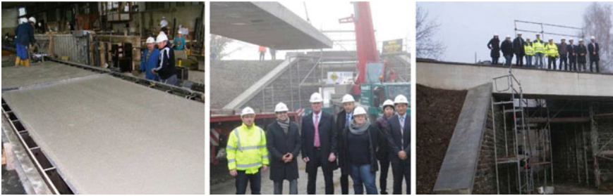
Fig. 21.1 Concrete prefabrication: set-up of the Rosenthal bridge at Olpe in Germany on 14 November 2012
