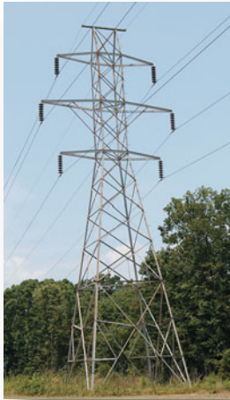
a. Electric power transmission line.
