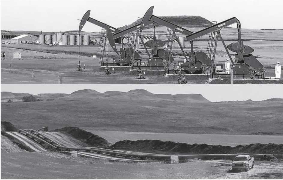
Figure 3.11 An oil well and pipeline construction in North Dakota. Source: Photo © H&O Soysal.
