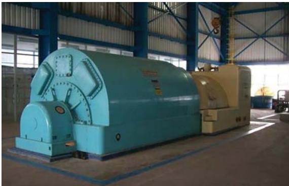
FIGURE 1.34 25 MW 850 psi generator and steam turbine. (Courtesy of Teco-Westinghouse.)
