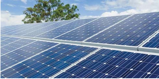
FIGURE 1.62 Array of PV panels. (Courtesy of Ener Power.)
