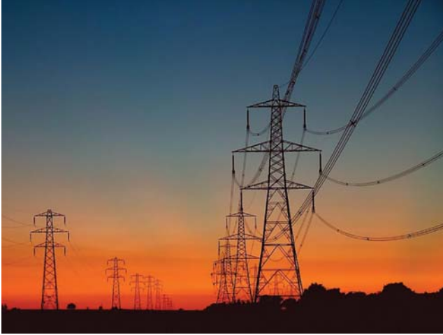
FIGURE 1.28 765 kV Transmission lines. ( http://www.tonyboon.co.uk/imgs/pages/power-lines.htm .)
