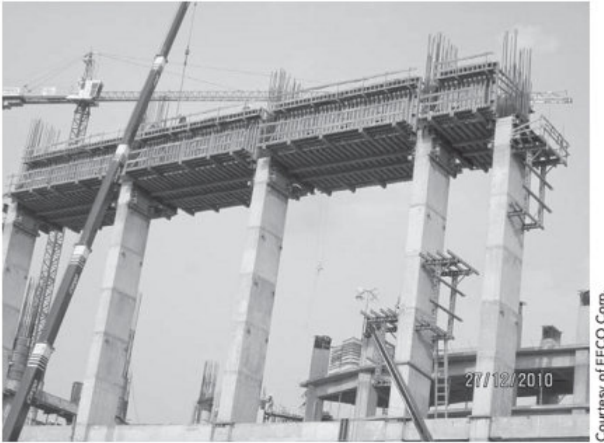
Mega beam concrete construction 100' above grade. Arena ciudad de Mexico, Mexico City, Mexico.
