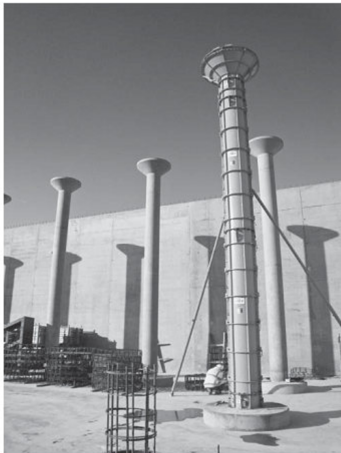
A 10M gallon water reservoir required 144 30' columns to support its roof in Oxford, United Kingdom.
