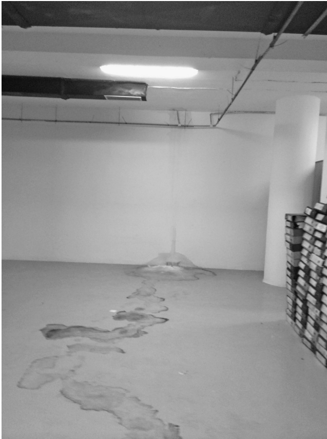
Figure 4. The basement (and depository) of the Macedonian National Archives after a water leak. Note the binders of documents on the floor, close to water marks. Photo: Anonymous
