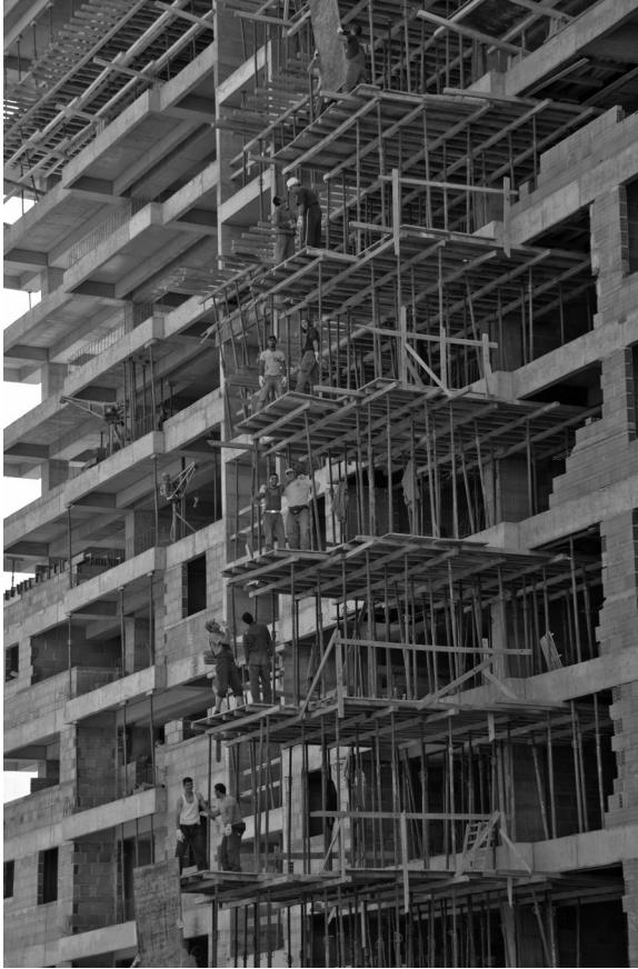
Figure 12. Workers without harnesses stand on scaffolds while they lower materials manually at a work site of one of Construx's competitors. Photo: Author
