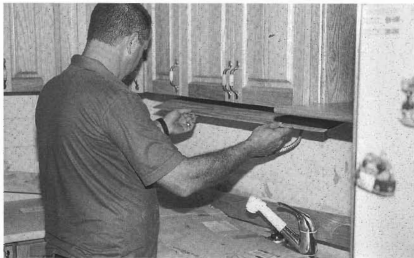
Fig. 17-7 \frac{1}{4} " plywood veneer is applied to the underside of the upper cabinets.
