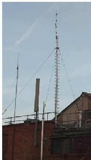
The TETRA mast on top of the Commodore Cinema in the centre of Ryde
