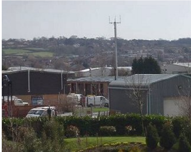
A TETRA mast appropriately placed in front of the mental health unit at St Mary's hospital, Newport, Isle of Wight
