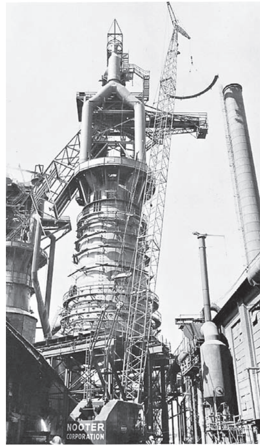
Fig. 3-7 This blast furnace will produce over 1,800 tons of pig iron daily. The furnace stack and other accessories, fabricated by welding, contain over 2,400 tons of steel plate and structurals. © Nooter Corp.
