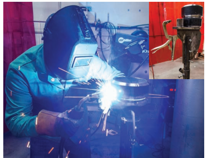
Fig. 24-23 Tacking 2G position joint with appropriate bent filler wire to hold root opening. It is being held in place by a shop build pipe stand. A small surface is used for initial set up like high low alignment. It can then be clamped into place for positions 2, 5, and 6 as required. The height can also be adjusted. Location: UA Local 400 © McGraw-Hill Education/Mark A. Dierker, photographer
