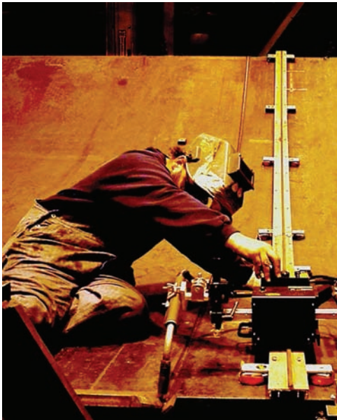
Fig. 26-22 A vertical V-groove butt joint is being welded uphill with the FCAW-G process. This is a mechanized application using semiautomatic welding equipment. The carriage is performing accurate speed control, side-to-side weave can also be machine controlled. However, the operator is required to monitor and control joint alignment and various other weld variables as required by the weld pool and bead formation. © BUG-O
