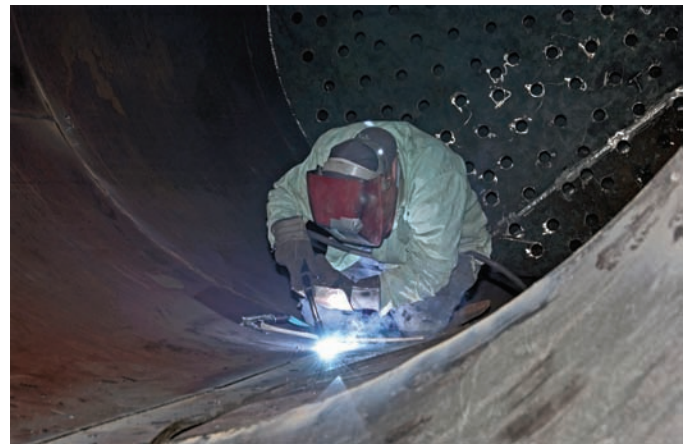
Fig. 21-4 Welding with the flux cored arc welding process. The welder is working on the longitudinal seam on the inside of a heat exchanger. © Miller Electric Mfg. Co.
