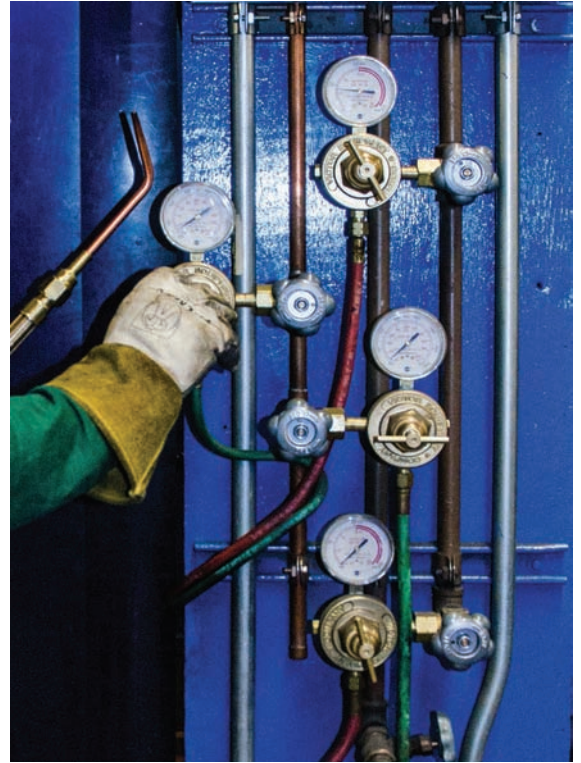
Fig. 5-9 This manifold system is being used to supply oxygen and acetylene to the booths on both sides of it. Location: Northeast Wisconsin Technical College © McGraw-Hill Education/Mark A. Dierker, photographer
