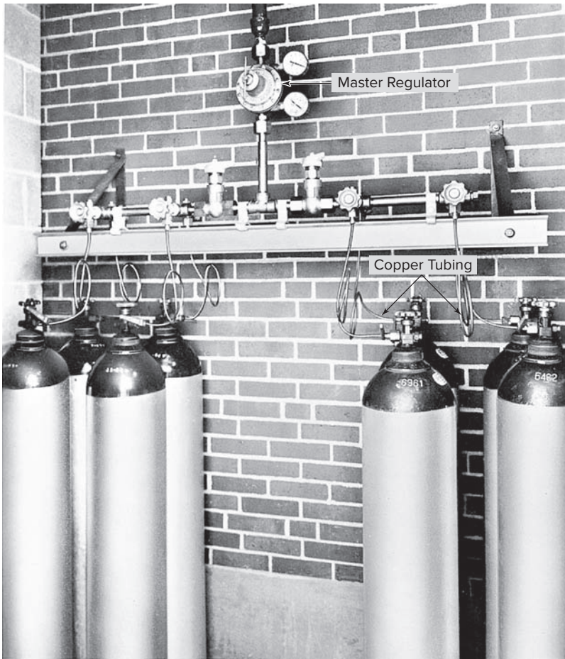
Fig. 5-13 Oxygen manifold system. Note master regulator and flexible copper tubing leading from each tank. © Thermadyne Industries, Inc.
