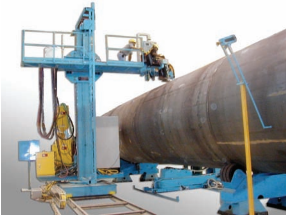
Fig. 23-31 Welds being made on a vessel with the SAW process. The manipulator is equipped with flux delivery and recovery systems. The traveler car and rails allow for making longitudinal welds while the turning rolls allow for making the circumferential welds. Note the operator catwalk and ladder for convenience and safety. © Pandjiris
