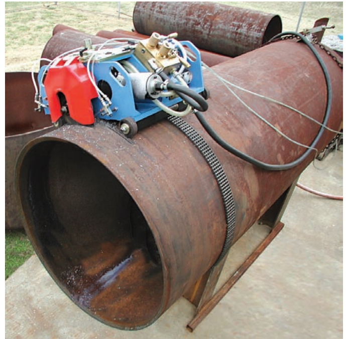
Fig. 16-83 Cutting a large diameter pipe with the automatic pipe saw. © Mathey Dearman
