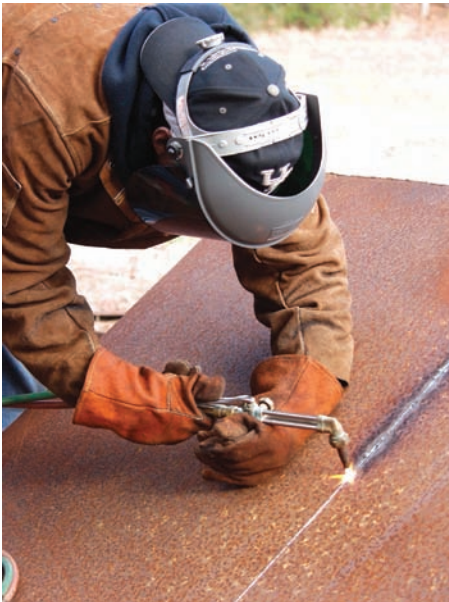
Fig. 7-34 Plates can be cut at the point of fabrication and need not be carried to another machine for cutting and back again for fabrication. © Sonda Dawes/The Image Works
