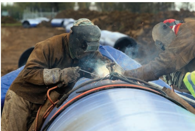
Fig. 16-3 Overland pipeline being welded in the field. Note that a welder works from each side of the pipe. © Nigel Bowles/Alamy Stock Photo
