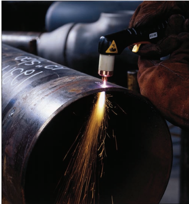
Fig. 17-2 Plasma arc cutting a thin wall stainless-steel pipe that will be used in the food processing industry. Flame retardant material has been placed inside the pipe to protect the inner surfaces from the molten dross of the cut. Note the gloves protecting from heat and flying sparks. © Miller Electric Mfg. Co.
