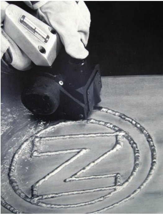
Fig. 26-66 Removing weld reinforcement with a pneumatic portable weld shaver. © Zephyr Manufacturing Company
