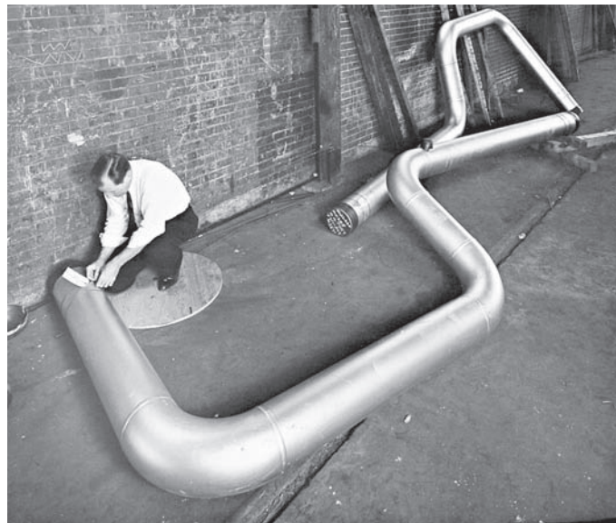
Fig. 2-26 The main steam system piping for the engine room of a nuclear submarine. © Crane Co.
