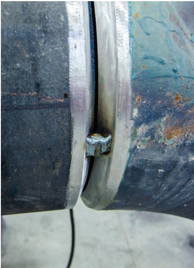
Fig. 20-14 Another form of bridge tacks being used to support large diameter heavy wall pipe and elbow as they are being positioned for welding. These bridge tacks will be evenly spaced around the pipe. © McGraw-Hill Education/Mark A. Dierker, photographer
