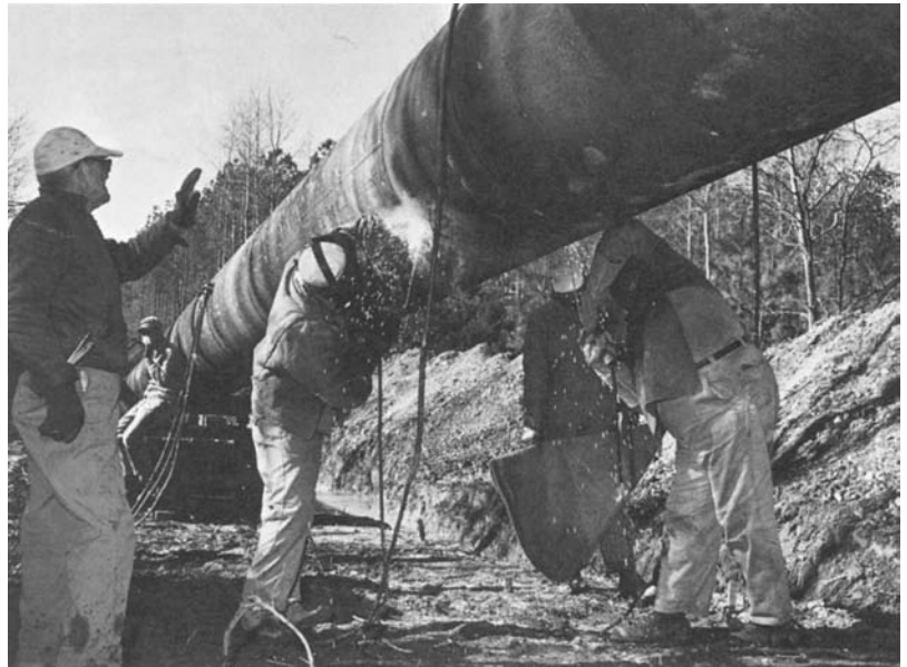
Fig. 16-4 Making a position weld on a pipeline. Travel is downhill, but travel uphill is a welding procedure used on some applications.
