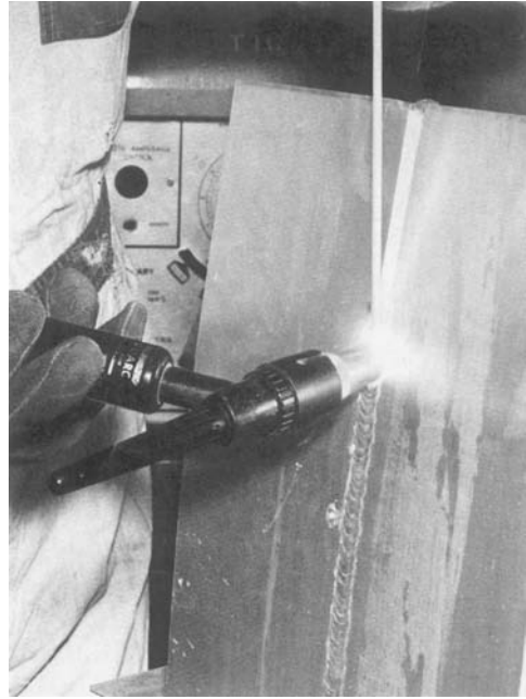
Fig. 19-37 Positions of the torch and filler rod when welding a butt joint in the vertical position in aluminum plate. © Kaiser Aluminum
