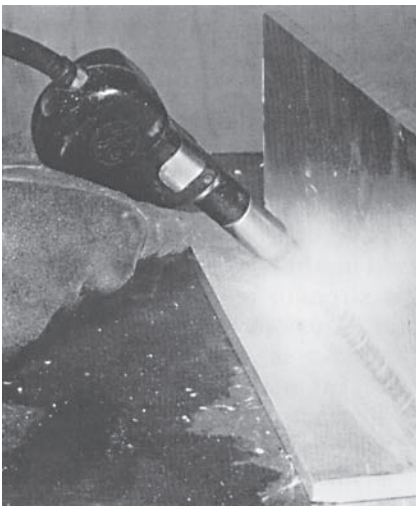
Fig. 22-35 Position of the MIG gun when welding a T-joint in aluminum plate in the 2F position. © Kaiser Aluminum
