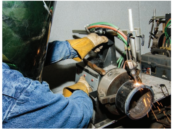
Fig. 16-87 Welding apprentice using a commercial pipe-beveling machine. The short pipe practice coupons can easily be beveled on both ends with this machine. Location: UA Local 400 © McGraw-Hill Education/Mark A. Dierker, photographer
