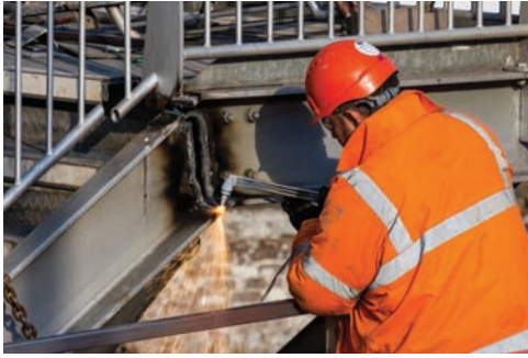
Fig. 6-1 A construction worker using an OFC torch to scrap an obsolete riveted structure. © lowefoto/Alamy Stock Photo
