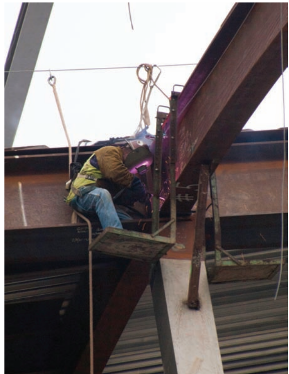
Fig. 2-29 A welder performing FCA welding on a bridge. Keep in mind all the welded joints and thermal cutting that would typically go into the fabrication and construction of a bridge. © McGraw-Hill Education/Mark A. Dierker, photographer
