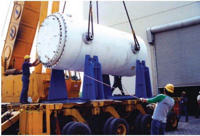
Fig. 1-9 Workers using a crane to lift a cask filled with highly radioactive fuel bundles at a Hanford, Washington, nuclear facility. The construction of this type of vessel relies heavily upon welding. © U.S. Department of Energy/AP Images
