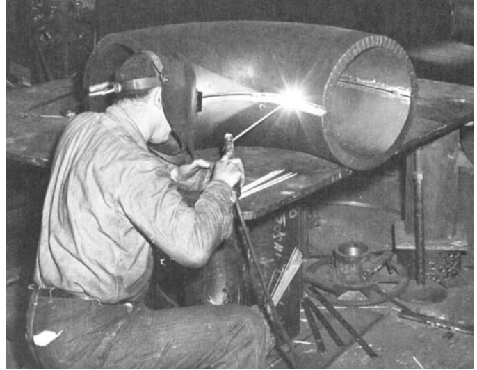
Fig. 16-80 Tacking up a fabricated L. It is 18 inches in diameter and has a wall thickness of 2 inches. © Crane Co.
