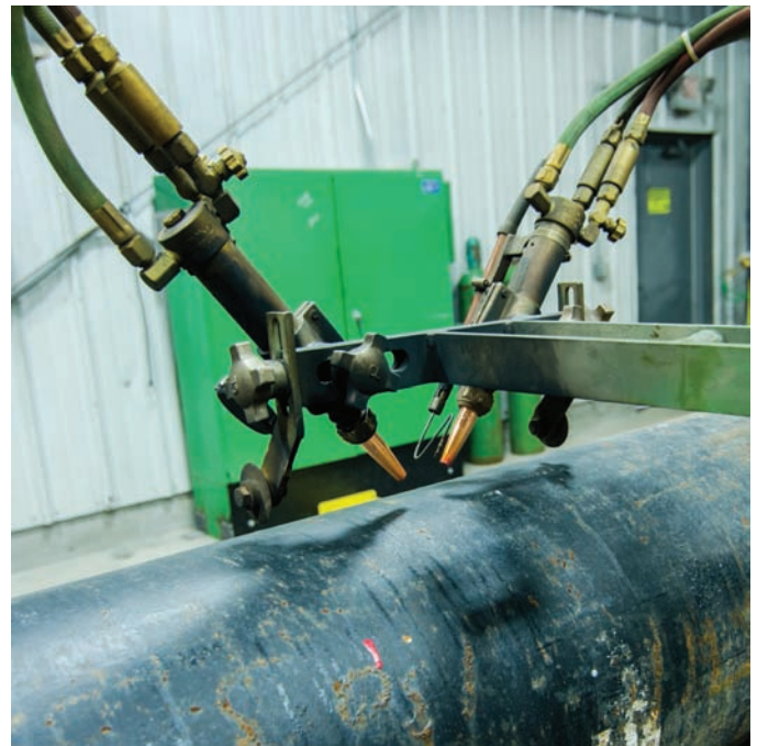
Fig. 7-11 Two mechanized cutting torches mounted in a fixed position over the pipe that is being rotated. This is set up in a high production high quality pipe spool fabrication shop. To cut pipe to length with the appropriate beveled ends. Location: Piping System's Inc. © McGraw-Hill Education/Mark A. Dierker, photographer
