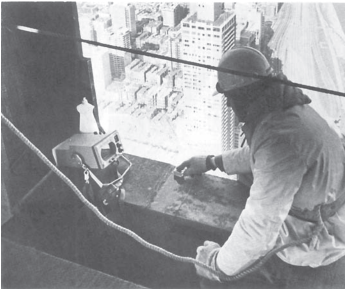
Fig. 28-48 Using portable ultrasonic instrument to check a structural weld on the seventy-sixth floor of the John Hancock Building in Chicago. © Magnaflux
