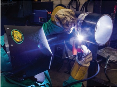
Fig. 20-36 Welding of carbon steel with the pipe axis in the horizontal fixed orientation. The weld is started at the bottom, and travel is up. This is a (5) position weld. Filler metal is being used on this V groove weld on a butt joint. Location: Northeast Wisconsin Technical College © McGraw-Hill Education/Mark A. Dierker, photographer
