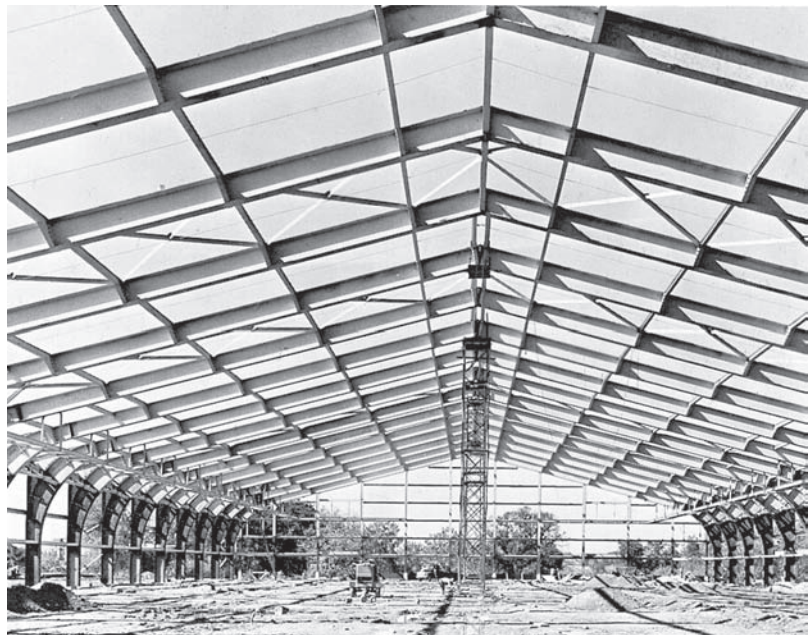
Fig. 2.30 Industrial building interiors take on an entirely new appearance. Arc welded rigid frames replace conventional truss sawtooth framing. Note the absence of columns and the improved headroom. © Lincoln Electric
