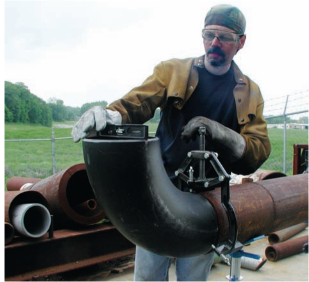
Fig. 16-23 This fast, easy-to-use clamp can be used to hold small fittings in position for welding. This clamp can adjust “Hi-Lo”™ of the elbow level checks the alignment. © Mathey Dearman
