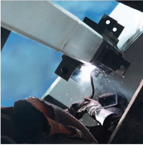
Fig. 23-1 Structural steel being welded with the flux cored arc welding process and a self-shielded electrode. © Lincoln Electric
