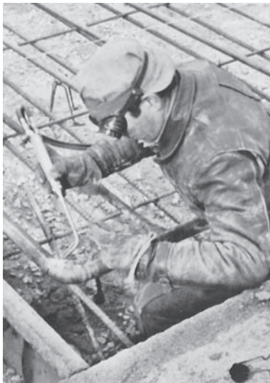
Fig. 5-2 Oxyacetylene welding a small diameter pipe on a construction site. This is a radiant heating installation in the floor.
