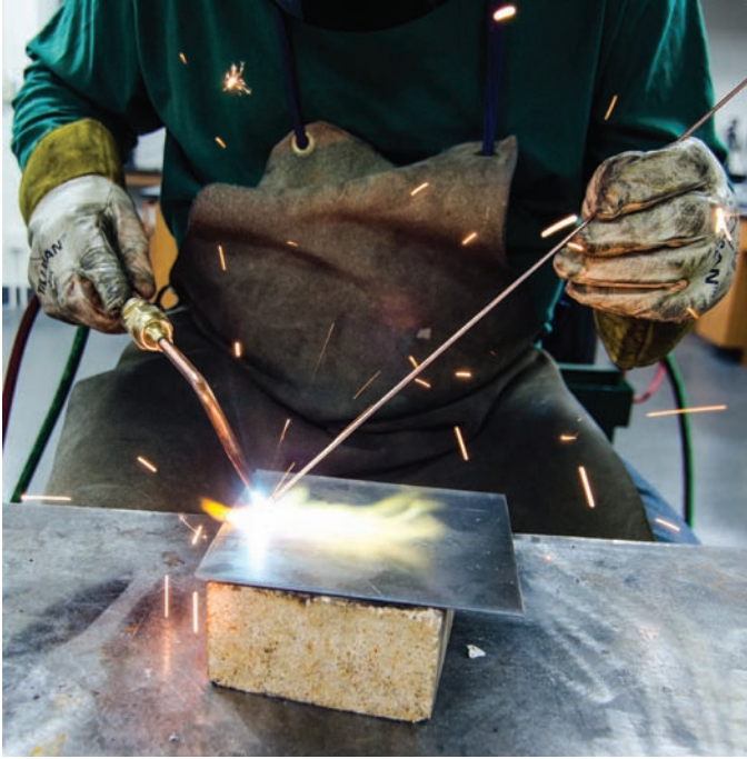
Fig. 5-8 Note torch and filler metal angles and location on this practice plate. Gases are being supplied via a manifold system as shown in Fig. 5-9. Bench top surface being protected with fire brick. Location: Northeast Wisconsin Technical College © McGraw-Hill Education/Mark A. Dierker, photographer
