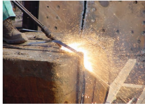
Fig. 6-19 An oxygen lance being used to cut cast steel. © American Welding Society, Welding Handbook , 8th ed. Vol. 2, p. 479, fig 14.26
