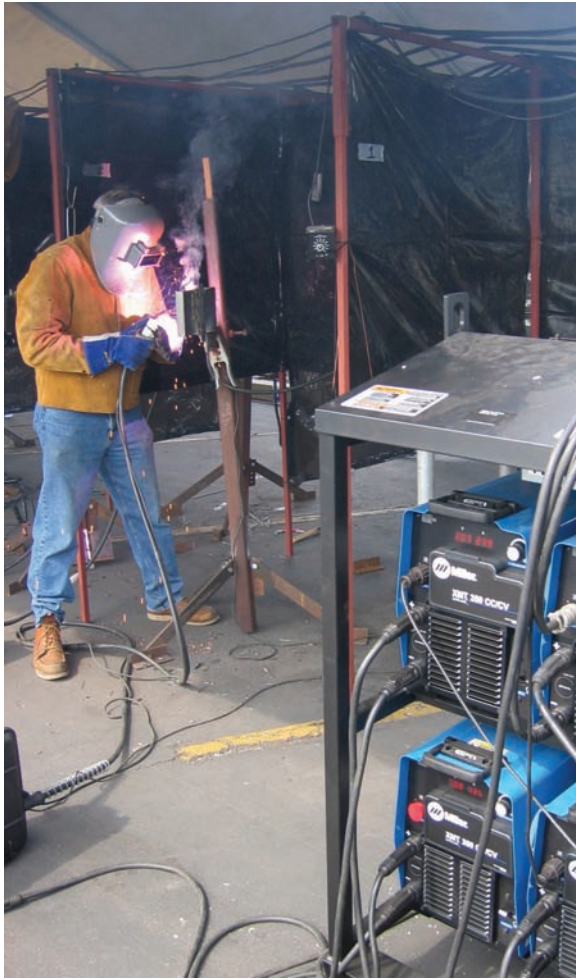
Fig. 23-30 An ironworker testing in the 3G position on 1-inch plate with backing. Note the head position in relation to the fumes and good body posture. This is a typical test that might be conducted on a job site in a temporary structure. © Miller Electric Mfg. Co.
