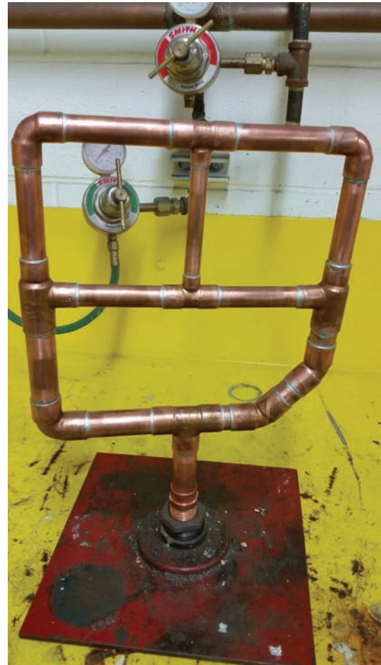
Fig. 10-36 Note all the various pipe sizes, elbows, Tees, and transition bushing from one pipe size to another. This will be visually, leak inspected and sized to the according print. Location: UA Local 400 © Edward R. Bohnart, Photographer
