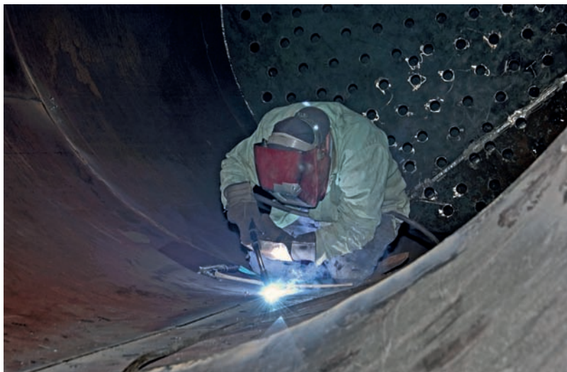
Fig. 32-28 This welder is working inside of a boiler shell that represents one of these conditions. © Miller Electric Mfg. Co.
