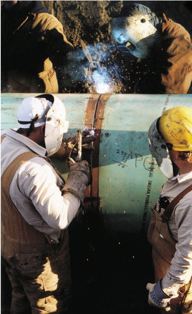
Fig. 15-1 Pipe welders working in unison to shielded metal arc weld a 5G position pipe butt joint with progression in the downhill direction for the root pass. Multi-Operator equipment is being used to supply the welding arc and auxiliary power for power cleaning and grinding tools. © Miller Electric Mfg. Co.
