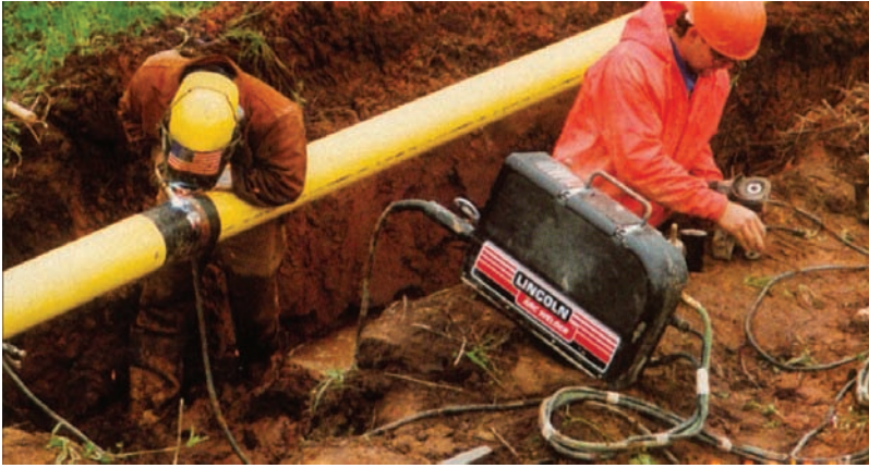
Fig. 24-1 Gas metal arc welding with the short circuit mode of metal transfer on a 5G position V-groove weld on a pipe butt joint for the natural gas industry. This highly skilled journeyman has been trained and skilled in a multitude of welding and cutting processes. The feeder is enclosed to protect it from the elements. The engine driven generator power source is located some distance away. Note the type of conditions that are typically encountered when doing welding in this field. © United Association
