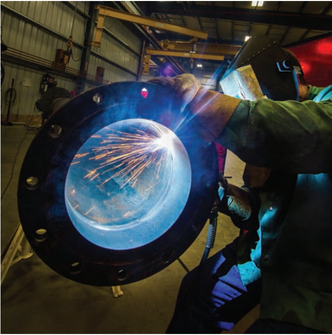
Fig. 24-4 Welding carbon steel pipe in the shop with GMAW-S process. The pipe is being rolled with a pipe positioner so the weld is being done 1G. Note arc and complete penetration weld taking place on this pipe to flange single V-groove weld on this butt joint. Location: Piping Systems, Inc. © McGraw-Hill Education/Mark A. Dierker, photographer
