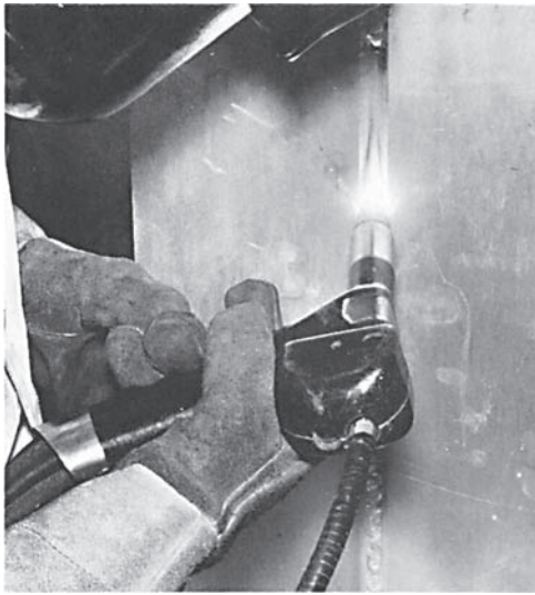
Fig. 22-38 Position of the MIG gun when welding a V-groove butt joint in aluminum plate in the 3G position, uphill. © Kaiser Aluminum
