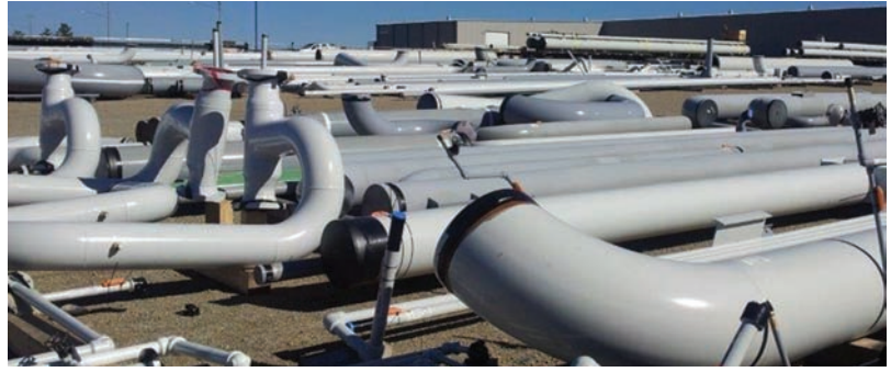
Fig. 16-79 An example of a laydown yard for storage of completed and painted pipe spools can be stored until required on the job site. © Piping Systems, Inc.
