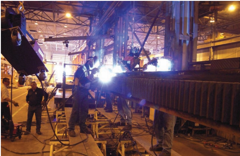
Fig. 2-23 These rack gears being MAG welded are made from forged and heat treated 8630 material. It is being welded to the beam section which is A514, 100K yield material. Four to six welders were engaged in preheating and welding. It was preheated and welded from both sides via fixturing and head and tail stock positioners to reduce distortion. This rack is used to moves a 3.5 million ton counterweight during lifts. © The Manitowoc Company, Inc.
