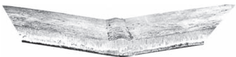
Fig. 3-45 V-groove butt joint shows evidence of extreme distortion, but it may contain no shrinkage stresses.
