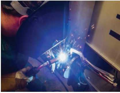
Fig. 24-37 MIG welding pipe in the 5G position. Care must be taken to follow the contour of the pipe. The welder is just leaving the top of the pipe (12 o'clock) portion of the pipe. The root pass is being done in the downhill direction. Location: UA Local 400 © McGraw-Hill Education/Mark A. Dierker, photographer
