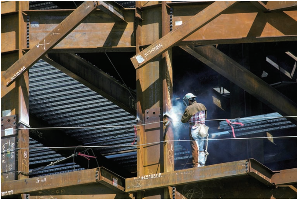
Fig. 3-65 The construction industry uses a tremendous amount of welding. This welder is working on some column splices. Note the safety lines, fall protection, and personal protective clothing for the welding. If you like working out-of-doors and like heights, this might just be the line of work for you. © Network Productions/The Image Works
