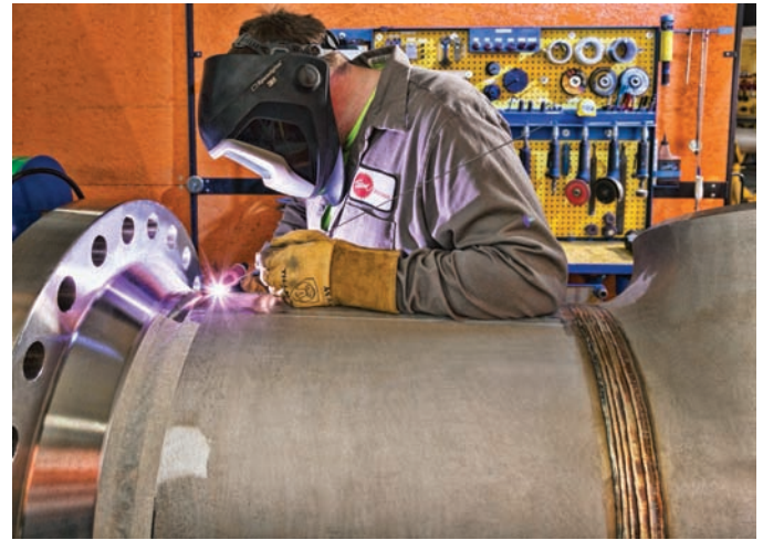
Fig. 20-18 The relative position of the torch and filler rod when making a multi-pass rotational weld on a stainless steel flange to heavy wall pipe butt joint. This is being done on a positioner. Note the completed weld of the pipe to the “T” branch section, also the well-organized tool board in the background. © Team Industries, Inc.
