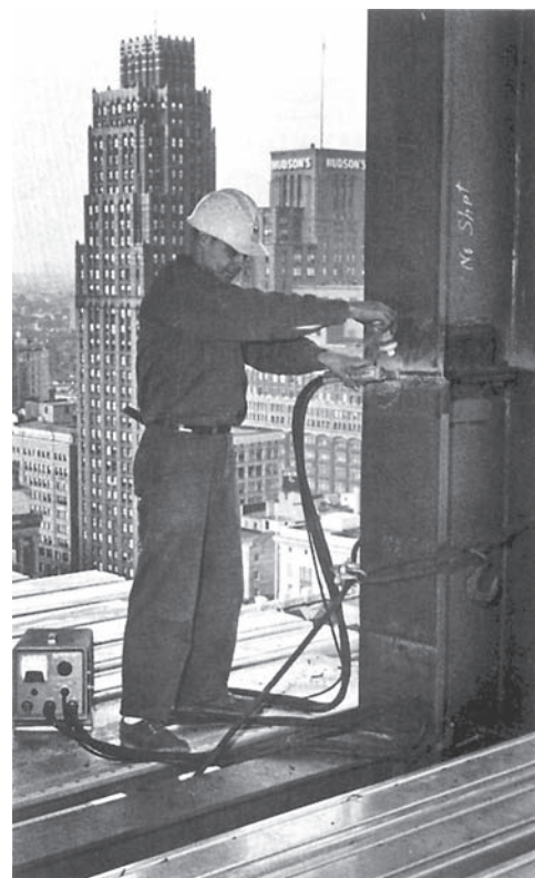
Fig. 28-31 A portable magnetic particle test unit checking critical welds during the construction of a Detroit bank building. Note the use of magnetic powder as the unit is applied. © American Welding Society. B1.10M/B1.10:2009, Figure 17, p. 19
