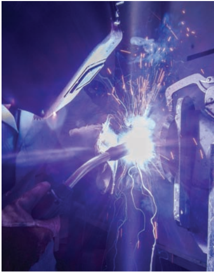
Fig. 24-38 The gun is in the 3 o'clock position of the pipe. Some welders find the 5G position very difficult. It involves a mixing of the flat, overhead, and vertical positions. Location: UA Local 400 © McGraw-Hill Education/Mark A. Dierker, photographer
