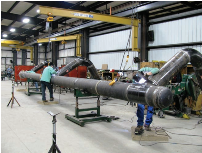
Fig. 2-19 A pipe header being fabricated in the shop. The roller allows the header to be position in the most advantageous position for weld quality and productivity. With a number of branches coming off. © Piping Systems, Inc.
