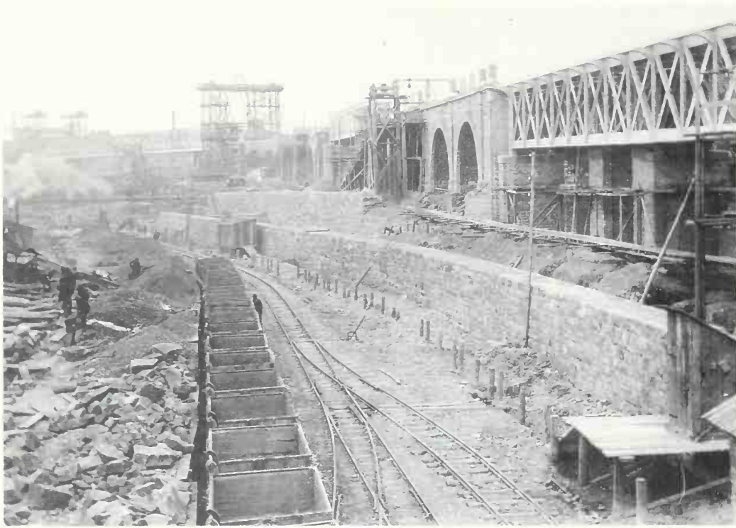
Otto Wagner, S-Bahn bridge across the Wienzeile, c. 1897–98. (Photograph by Otto Schönthal)
