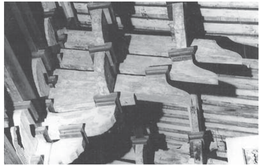
FIGURE 3.11. Bracket set (front part) of the Sanqing Hall (1015) at the Yuanmiao Daoist Monastery in Putian: note platelike board ( minban ) under blocks and inner concave contour of arms (courtesy of the Bureau of Culture of Putian, Fujian)
