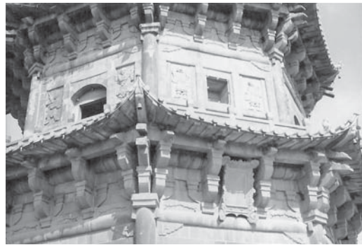
FIGURE 3.12. Bracket sets imitating timber structure on the western pagoda (1237) of the Kaiyuan Monastery in Quanzhou, Fujian: note the minban under the blocks (author photograph)
