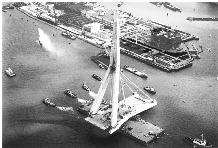
8. ERASMUS BRIDGE CENTRAL TOWER BEING BARGED INTO PLACE, ROTTERDAM, NETHERLANDS, 1996, UN STUDIO
