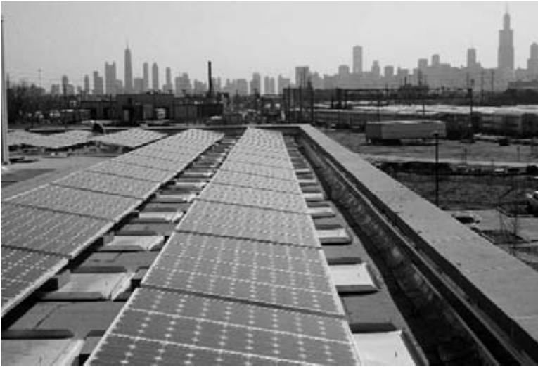
Chicago Center for Green Technology showing rooftop solar and Chicago skyline. (Credit: Timothy Beatley)
