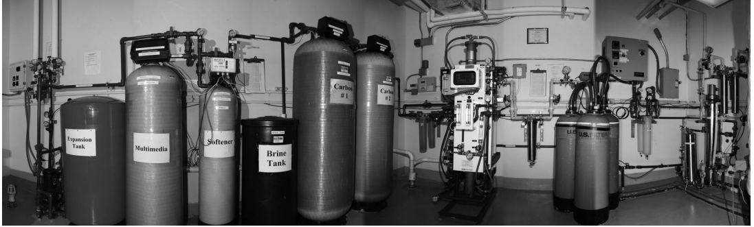
Fig. 1. A panoramic view of a modern water treatment plant.
