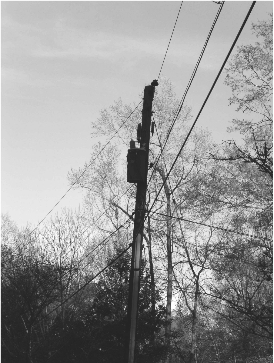
Figure 2.4 A utility pole-mounted transformer.
