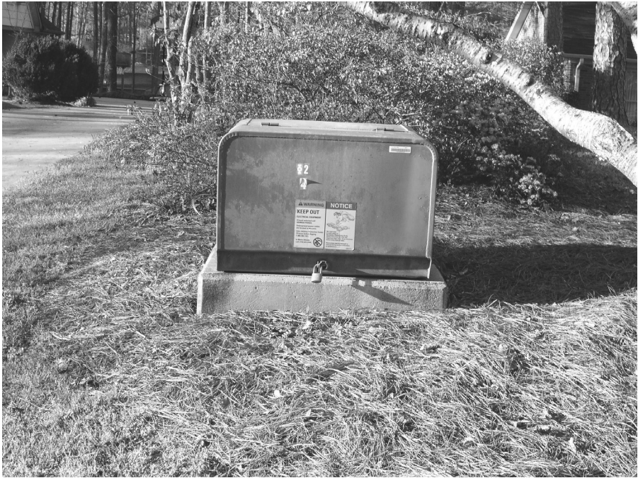
Figure 2.5 A metal enclosure used to house a transformer whose output flows onto underground power lines.
