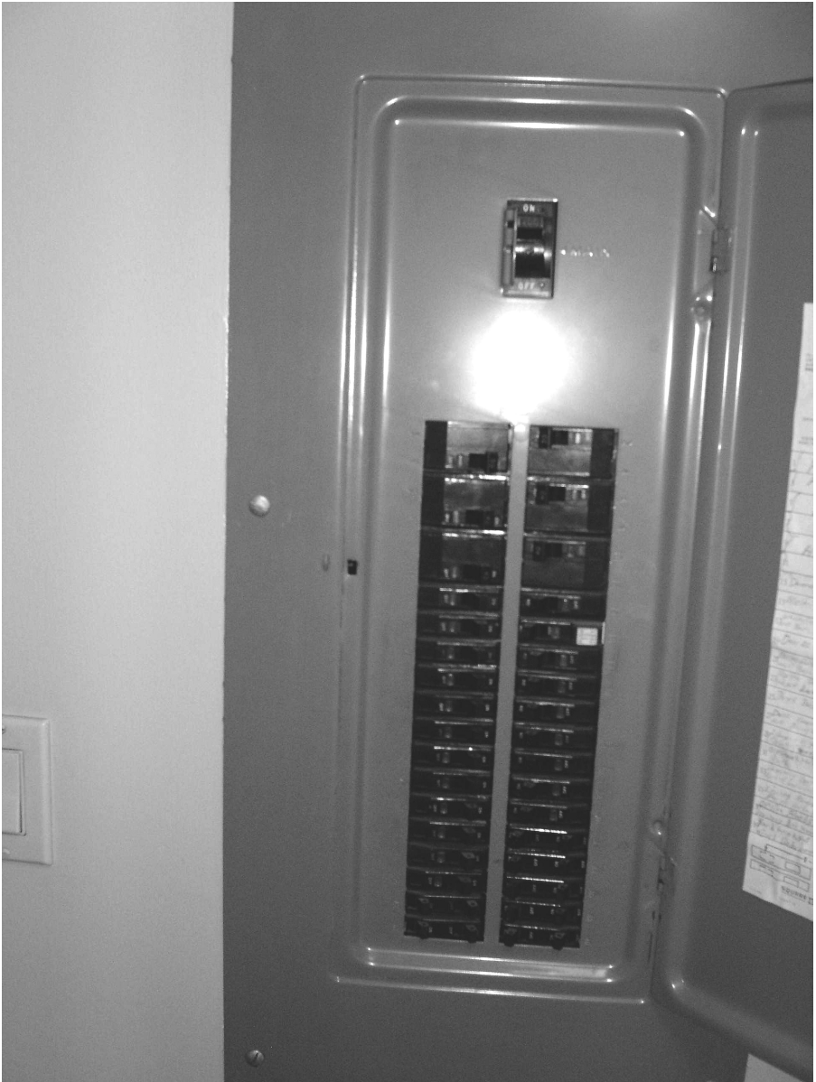
Figure 2.7 A breaker service panel.
