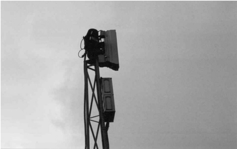
Figure 12.7 A P/T unit where the tilt mechanism gears have failed. This is a fairly common problem with these units, especially if the unit is carrying an excessive load
