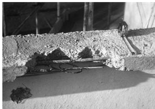
Figure 22.9 Concrete damage (Photograph: John Allan, Avanti Architects, London)
