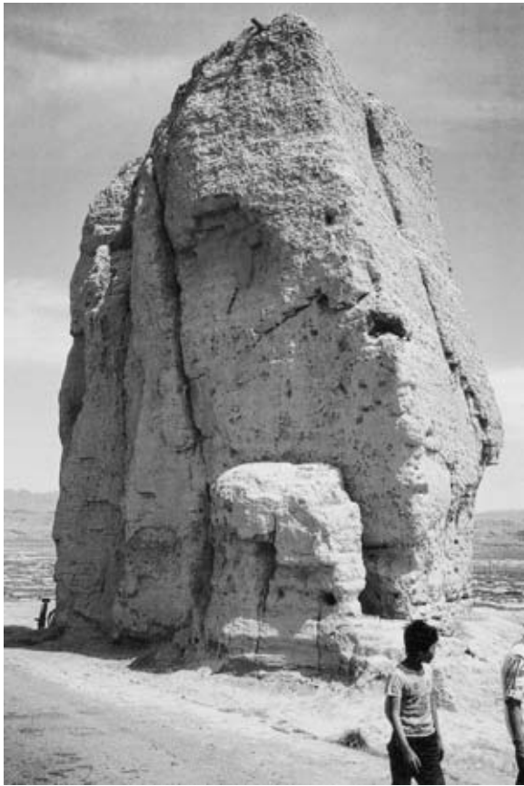
Figure 5.13 A tower, now an isolated fragment of the Great Wall of China, displaying vertical fissuring which causes the loss of segments in vertical slices. The loss of lateral restraint in the lowest zones effectively ‘unloads’ the compression previously applied to the bottom strata by the mass of superimposed earth. The lateral stress-release causes the peripheral mass to form shear cracks parallel to the external surface. This phenomenon is unique to earths, among building materials, due to its compressibility and low shear strength (Courtesy John Warren)
