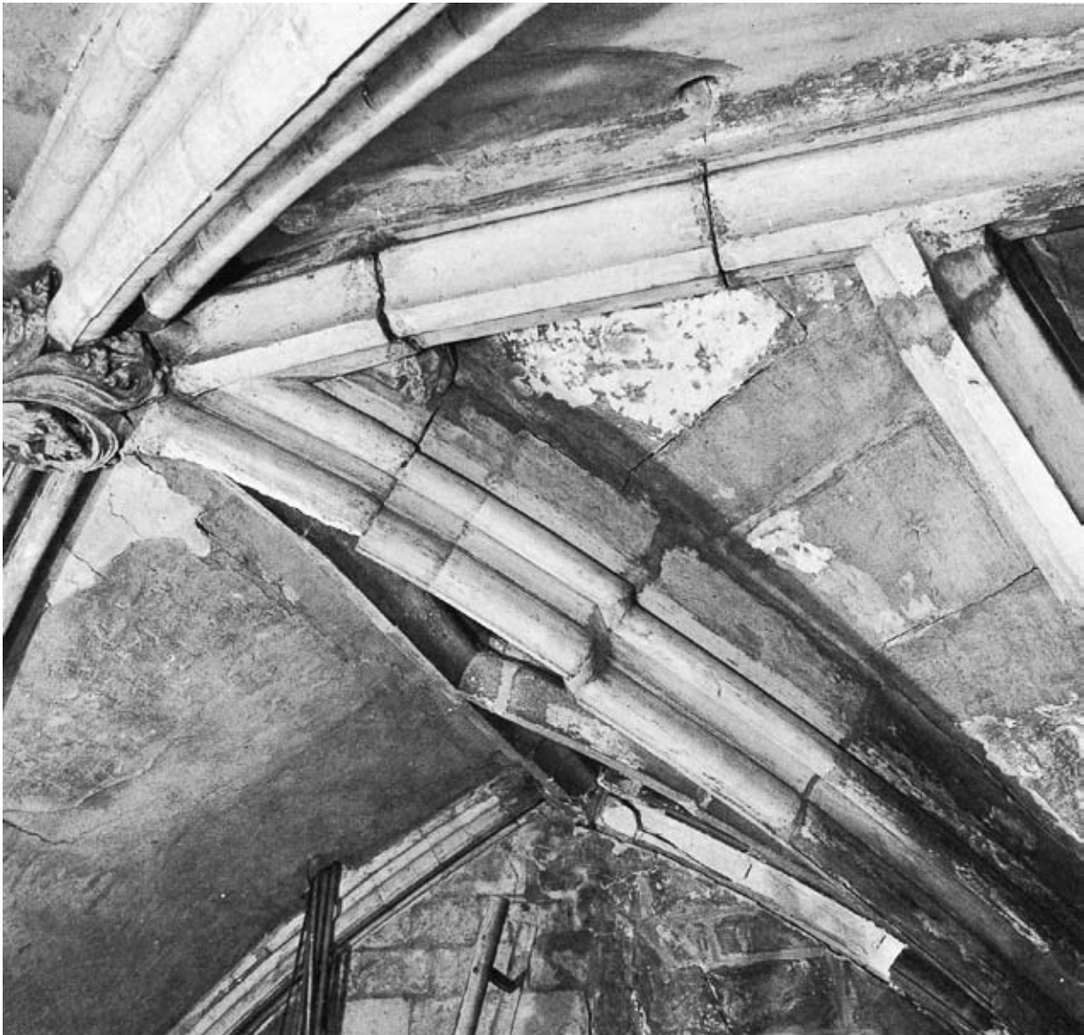
Figure 3.10 North nave aisle vault, York Minster, England (Courtesy: Shepherd Building Group Ltd)
