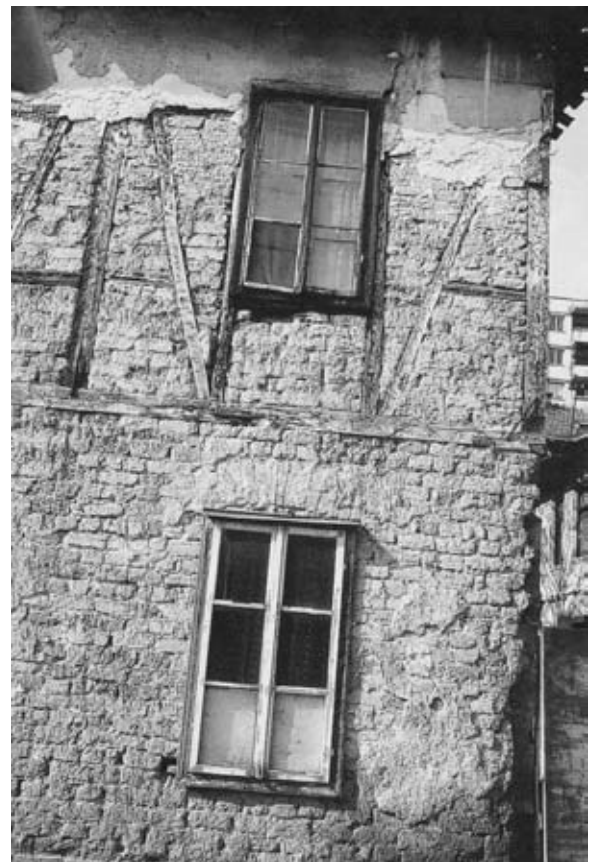
Figure 5.10 Earth construction typical of Europe, the Balkans, through mountainous Turkey, Mesopotamia and the Caucasus to the Himalayas. Here earth block is used in the understorey with a light timber framing above filled with similar block. An outer skin of rendering—stripped from this example—may be used externally
