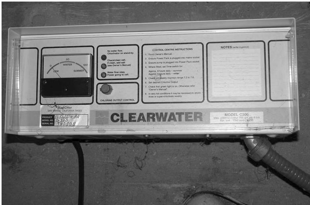
Figure 6.3 Photo of Clearwater chlorinator power supply and control.
