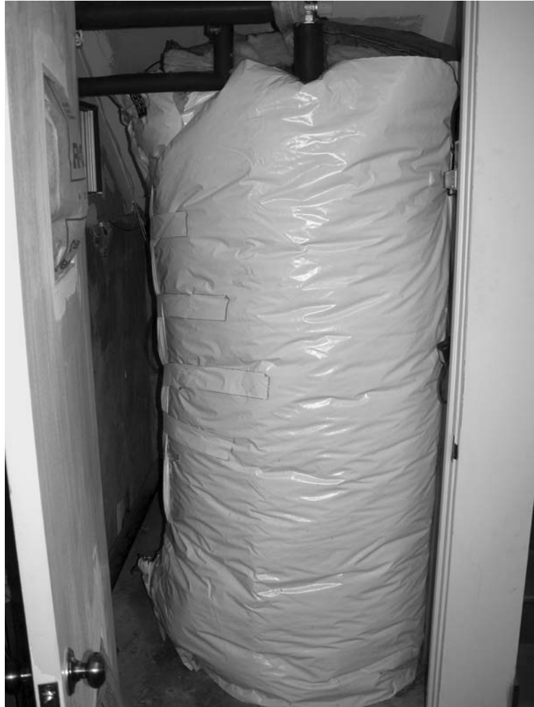
Figure 5.1 Photo of hot water heater in Berkeley solar house.
