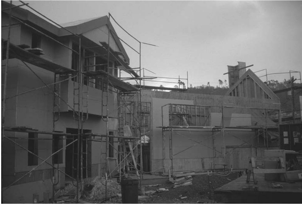
Figure A.5 Roof framing on second floor complete and preparing for the long rafters for the solar roof over living/kitchen/dining section.
