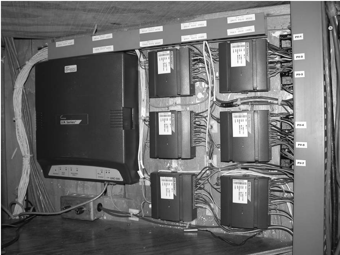
Figure 7.11 Photograph showing control closet hardware.
