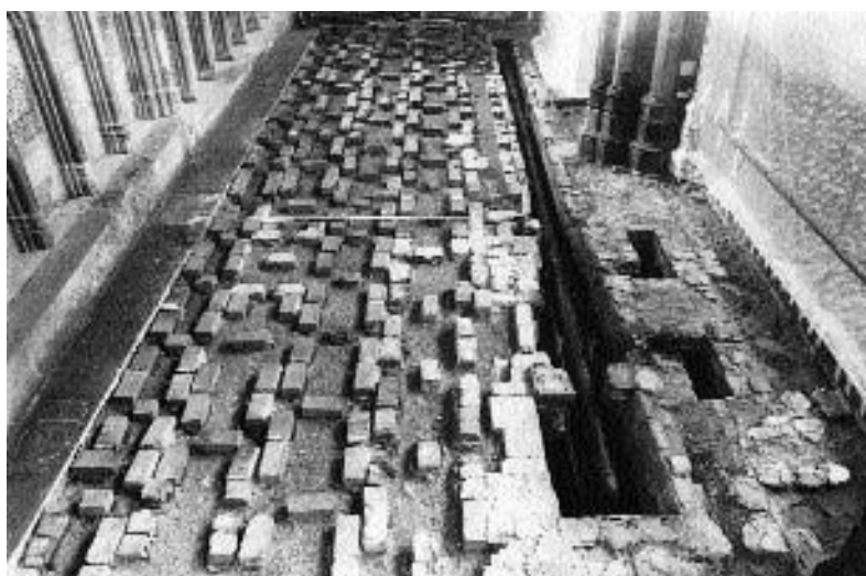
Figure 2.2 Lichfield Cathedral. Unusual brick sub-structure to support Scott's limestone paving of 1860 in the north choir aisle (Photograph, Warwick Rodwell)
