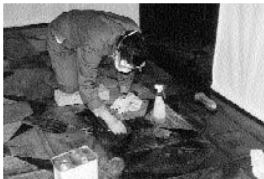
Figure 16.2 The Marble Dining Room: cleaning the marquetry floor of c.1744 in about 1992 (Photograph, F.R. Latham)
