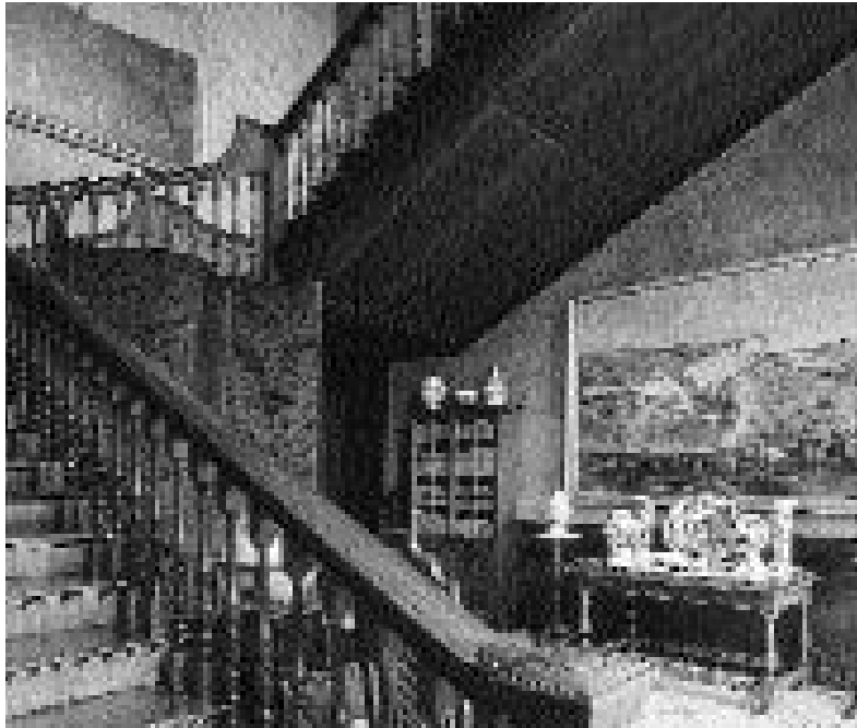
Plate 73 At Dyrham Park, near Bath, this main staircase cannot bear the weight of the constant flow of visitors. The treads and the landing also show damage from sharp heels. Now closed to the public – see page 198 (Photograph, National Trust)
