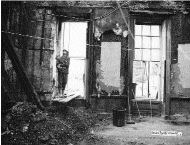
Figure 17.1 Uppark. Ash and debris being removed from the Red Drawing Room, revealing the floorboards intact (Photograph, The National Trust)
