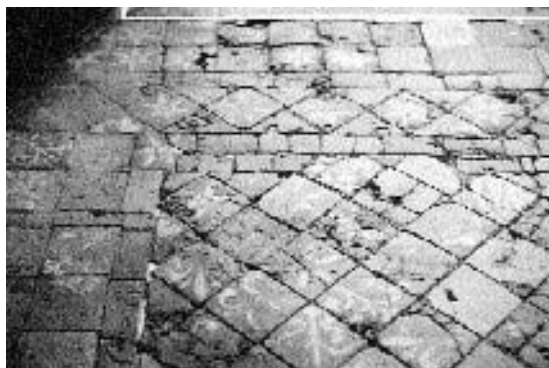
Figure 12.1 Tiles in the central vessel of the retrochoir before cleaning and conservation (Photograph, Cliveden Conservation Workshop Ltd)
