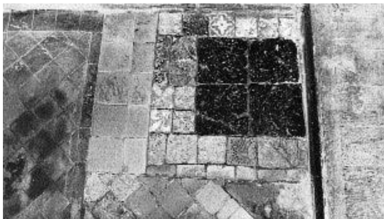
Figure 2.1 Lichfield Cathedral. Scott's 'museum' of tiles on the floor of the Consistory Court, 1861. Various thirteenth- and fourteenth-century designs surround four pieces of cannel coal which had been used for black and white paving in the choir in the late seventeenth century (Photograph, Warwick Rodwell)
