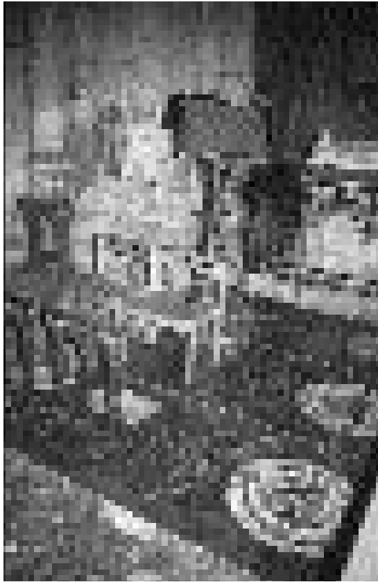
Plate 28 Winchester Cathedral, ledger stones within the nave sanctuary, damaged by furniture, now removed – see page 120 (Photograph, Jane Fawcett)
