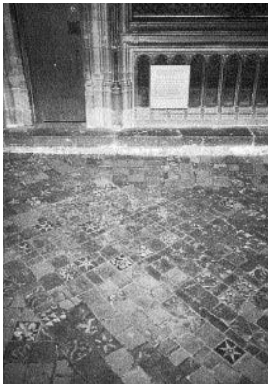
Figure 12.2 Conserved tiles, many of which are in situ, completed in the first stage of work. Isolated replica tiles are visible (Photograph, Peter Bird)
