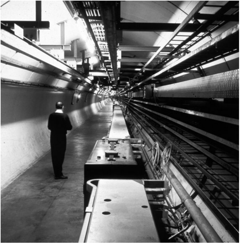
Figure 11.3. A view of the LEP tunnel. The beam travels in a pipe inside the multiple magnets that run down the centre of the picture. To the left is the track for a monorail that runs the length of the tunnel. To the right are various servicing and cooling ducts. (Courtesy CERN.)
