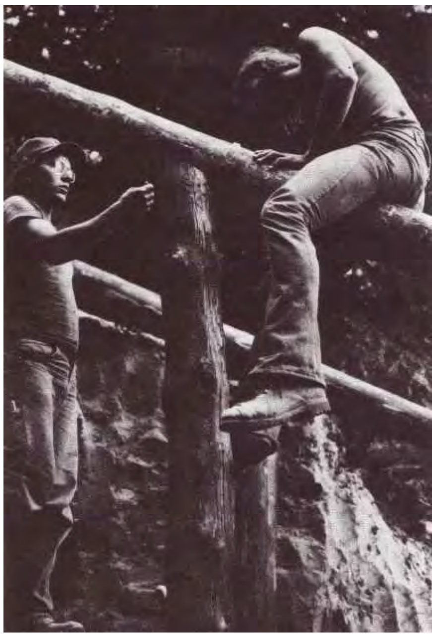
Chris and Steve talk over structural problem.
