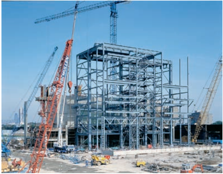
Figure 9.4 General progress shots of a construction site should be taken from the same spot with the same lens, and preferably show some foreground construction action
