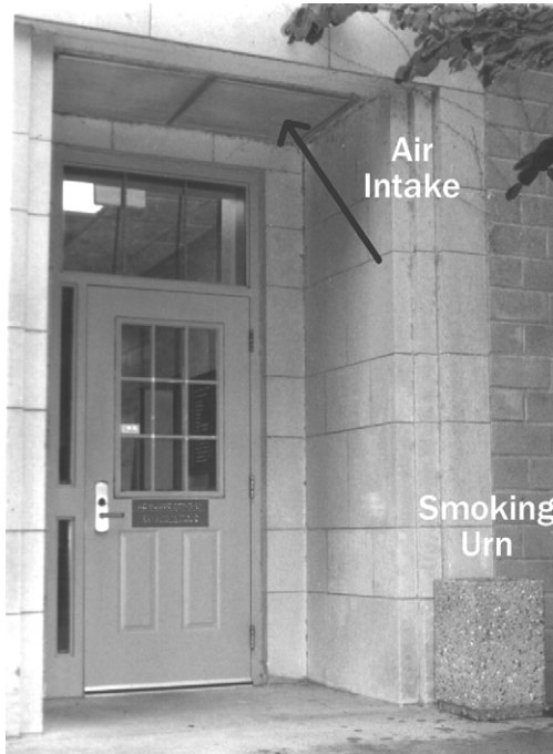
Figure 2.1. Placement of an air intake over a small building’s main entry door. Due to the location of the urn and smokers, outdoor ETS has often been entrained and distributed throughout the building (Rock and Moylan 1998).
