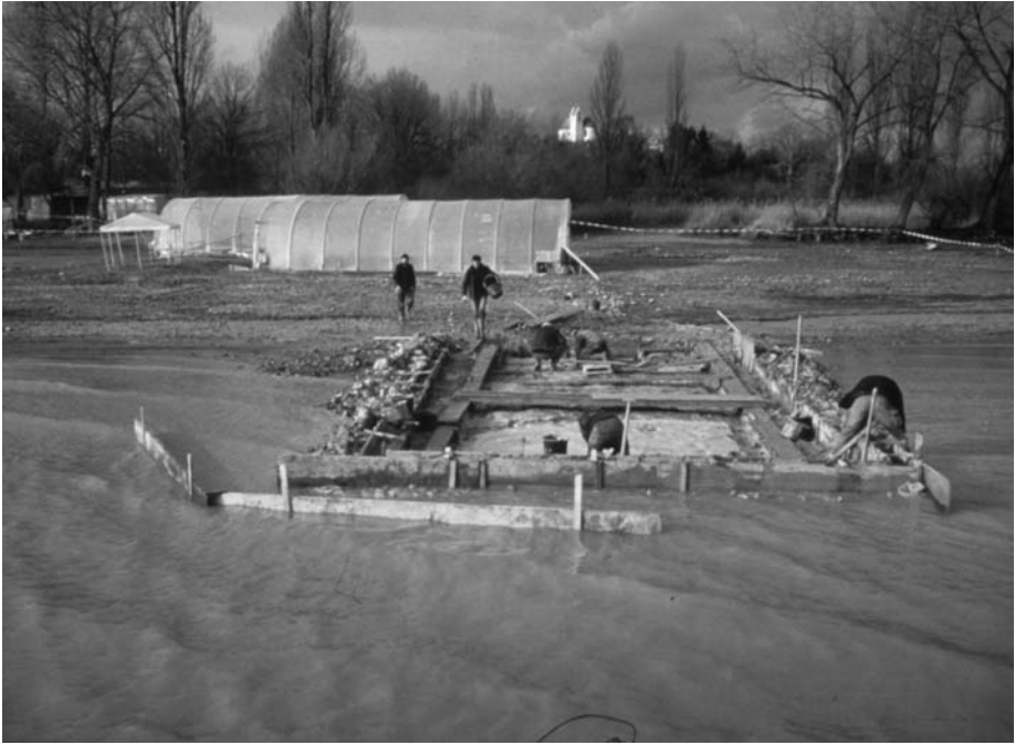
Figure 2.1 Excavation near Hornstaad at Lake Constance during wintry low-water levels. Photograph: Landesdenkmalamt Baden-Württemberg.
