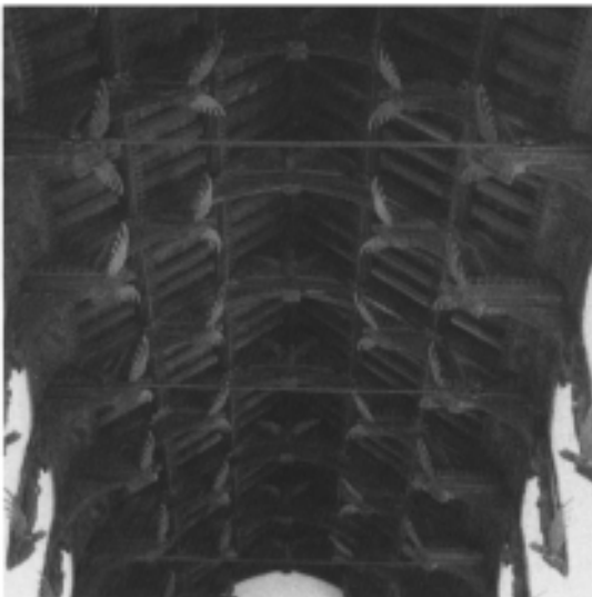
43 The magnificent roof to the church at March, added when the church was refurbished early in the sixteenth century.
