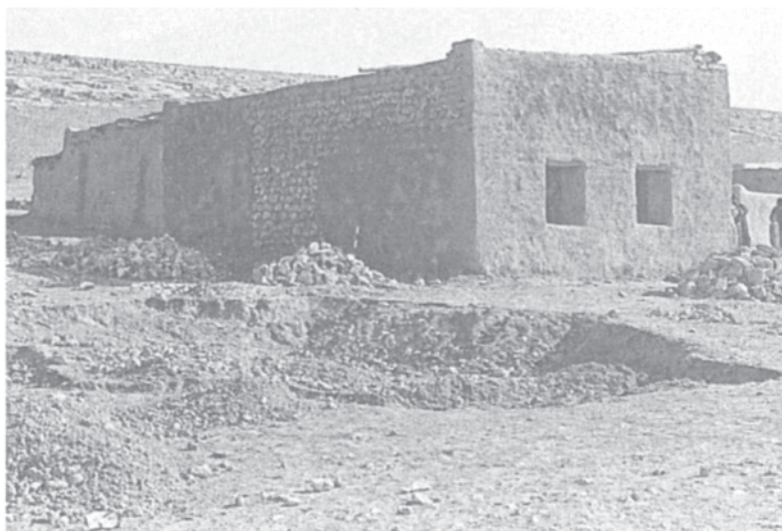
Figure 11.3 Shams ed-Din 1982: building a new house of stone, mudbrick, tin, and wood.
