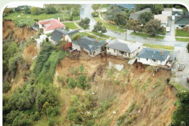
These cliffs on the Californian coast in the United States are made of soft rock. Houses along this coast quite often fall on to the beach as the cliffs erode.
