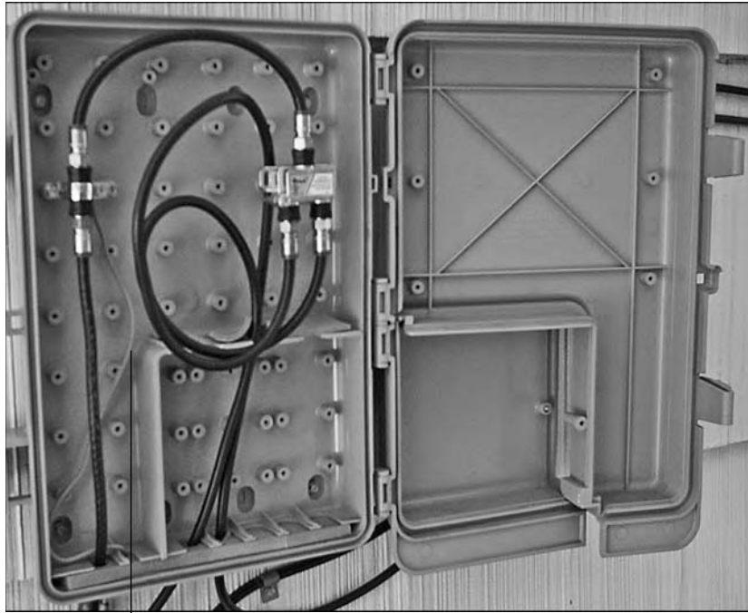
Figure 8-1: A typical cable TV interface box looks like this.
