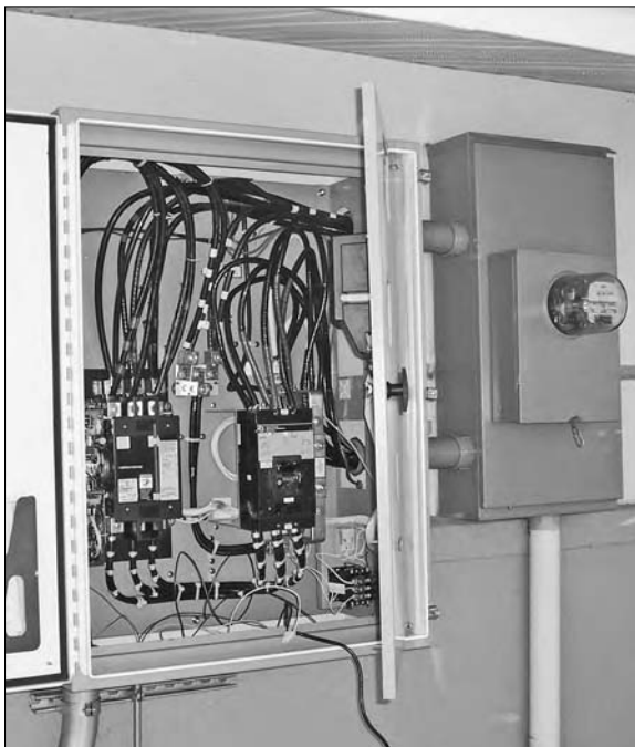
Figure 15-4: This switch transfers power for the whole home.
