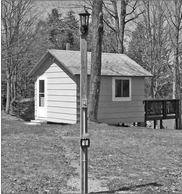
Figure 16-1: This installation brings light and power to an outdoor area.
