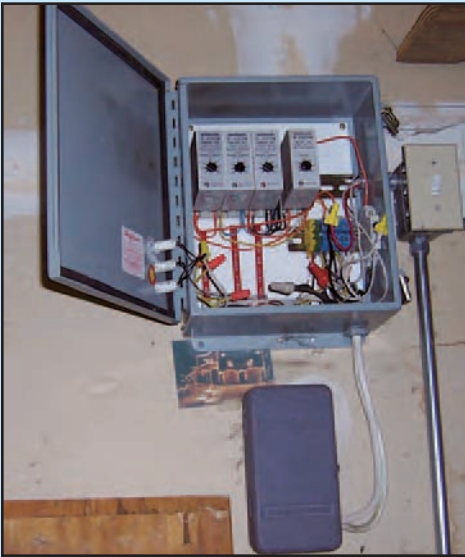
Color Plate 14: The finished control panel operates the antique stop signal shown in Color Plate 12. If you wire a controller for a traffic signal (covered in the “Just for fun: Wiring a traffic signal in your driveway” sidebar in Chapter 17), it may look very similar to this one.
