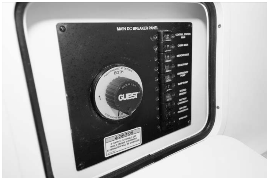
Figure 13-2: A typical battery iso- lator switch.
