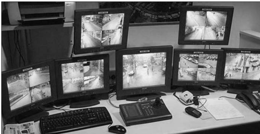
Figure 6-2: Surveillance monitors and camera control equipment.
