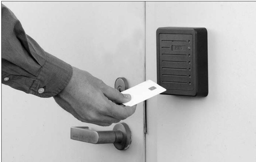
Figure 6-3: A contact-less proximity card reader permits users to enter a secure room or facility.
