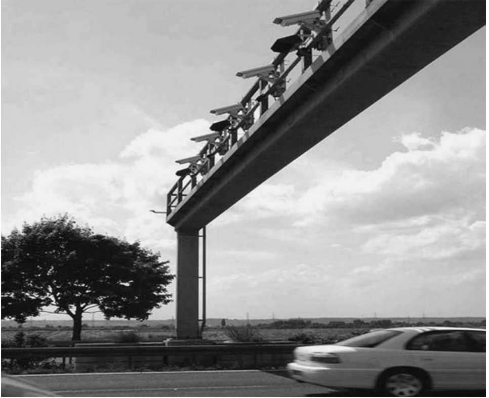
Figure 16.3 Gantry for road tolling and number-plate recognition (© Efkon AG)
