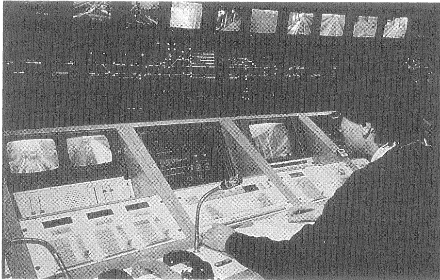
7. The control room for VAL in Lille. The success of big brother VAL cast a shadow on little Aramis. A major innovation: the former drivers are now positioned in front of a control panel, and regulate the movements of the automated trains from a distance. [Photo Matra]
